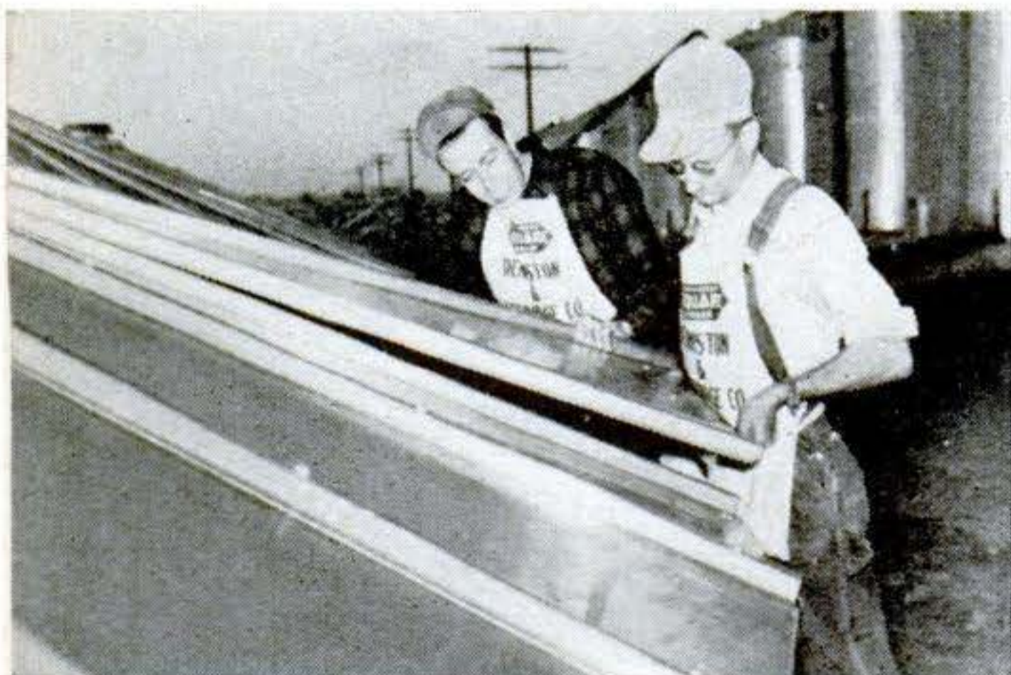
Workmen can put on the roof while standing on the ground. Roof is made up of pie-shaped aluminum wedges that dovetail together. Lightness of aluminum permits this unusual method.
