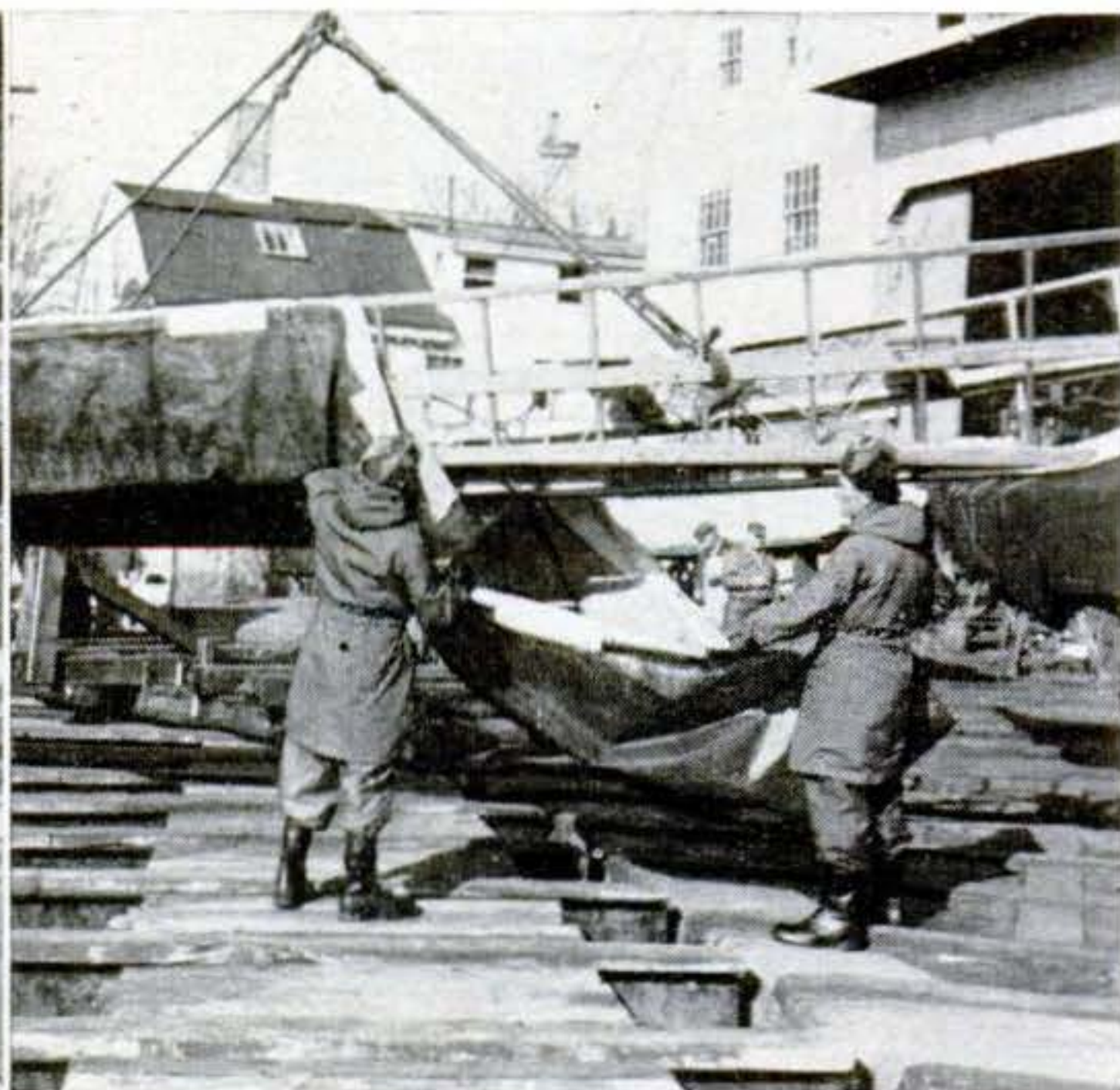
3 When sections are bolted together, skin is slipped on. Lashing draws it tight and secures it. Boat was constructed on dory-type lines at Graves boat yard, Marblehead, Mass.
