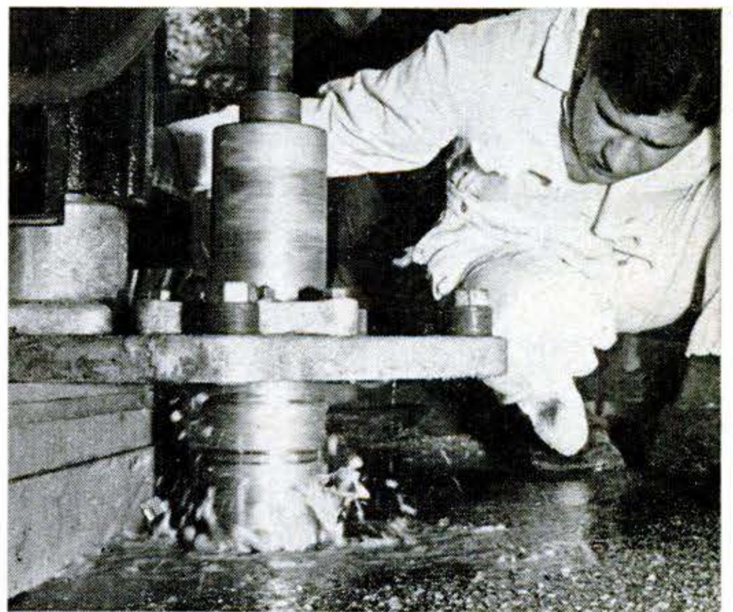
Steel tube edged with diamonds, whirling at 150 r.p.m., bites easily through rock, asphalt, and sand. Stream of water lubricates cutting tool.
