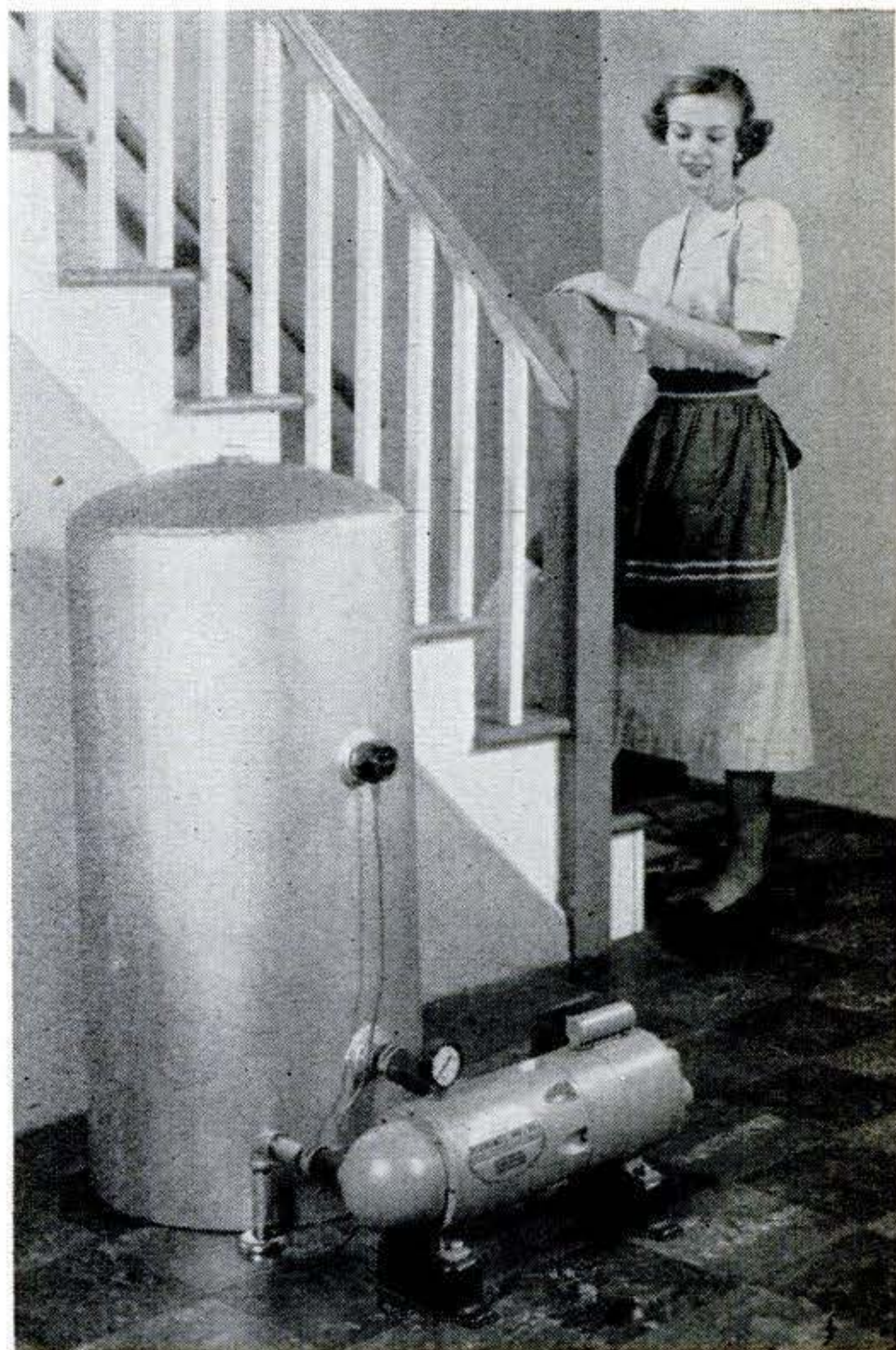
Small, streamlined jet pumps are becoming standard in many homes. This one lifts water about 20 feet, automatically starts when pressure tank gets low and shuts off when it builds up.
