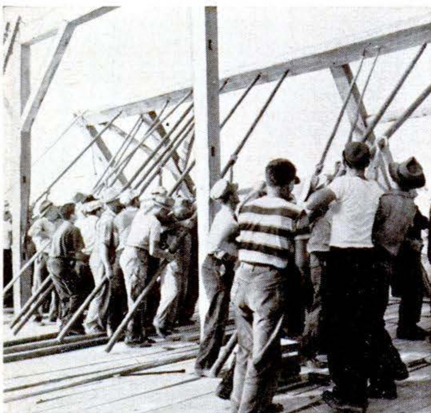
Everybody gets into the act for a major raising job. The men are using long pike poles, or "stockades." The entire section, including diagonal braces, was preassembled on the ground.
