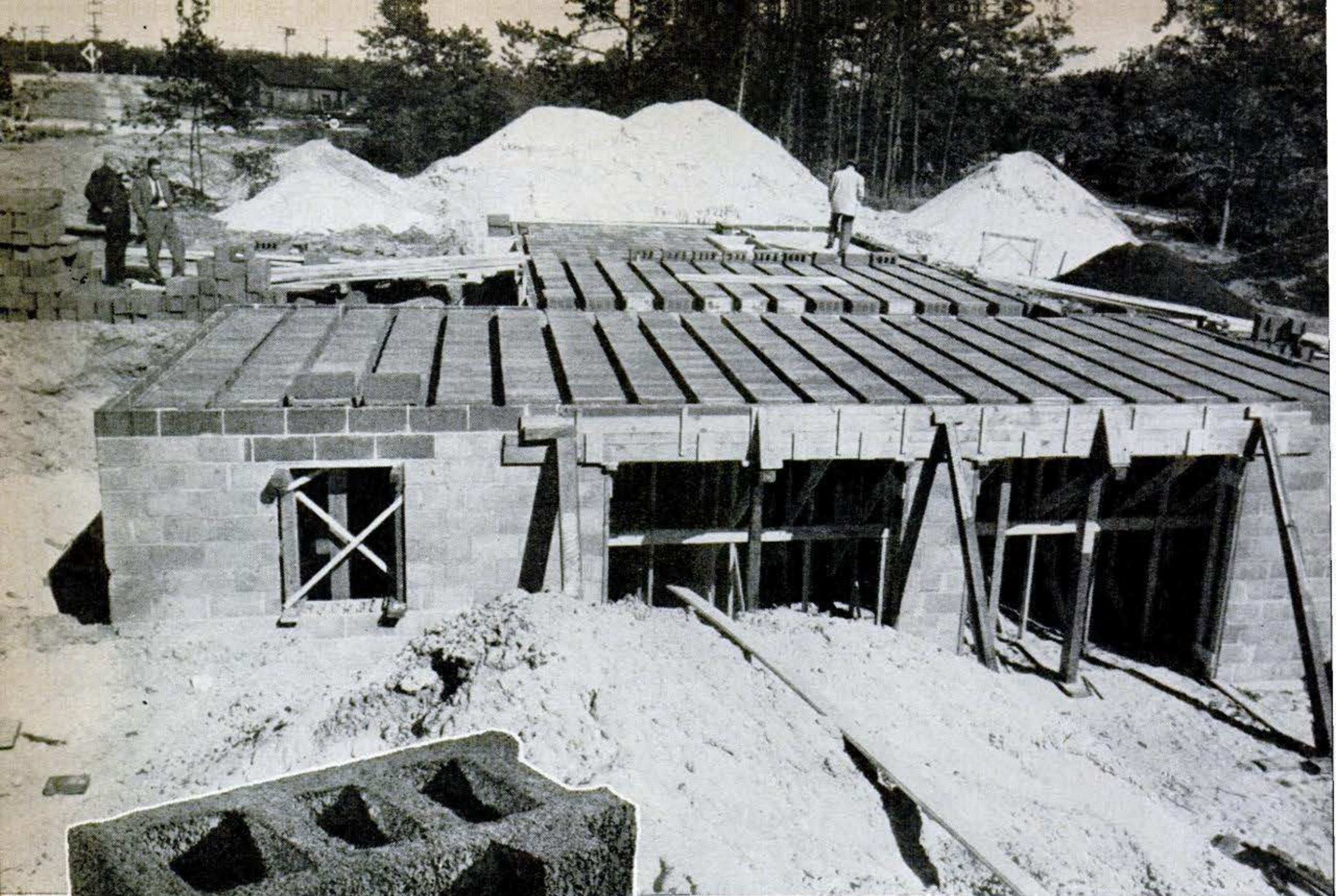
Home of Russell R. Ferrer has cinder-block floor. Concrete was poured between blocks.
