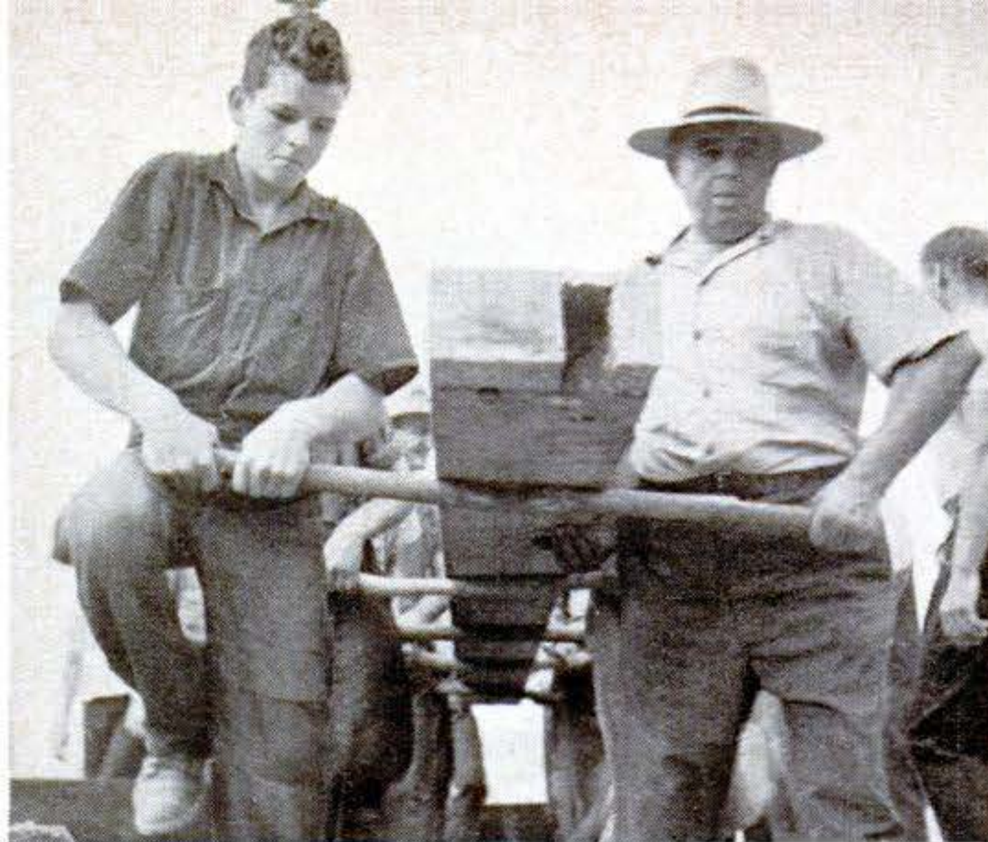
Old-fashioned muscle power puts giant beam where it's needed. Longest single timbers, 45 feet, span entire width of barn. Steel girders are used only in foundation against damp hillside.
