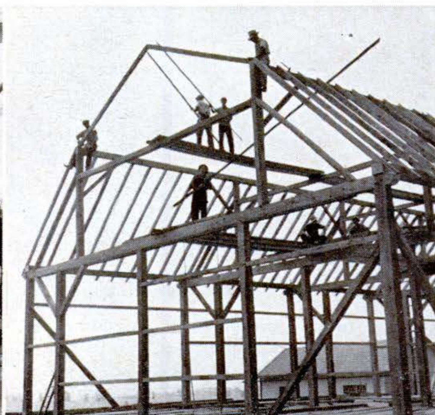
Here first of the top rafters are swung into place. Roof is of gambrel type, with a flatter slope at the top. Haymow is reinforced so sides won't bulge when it is tightly packed.
