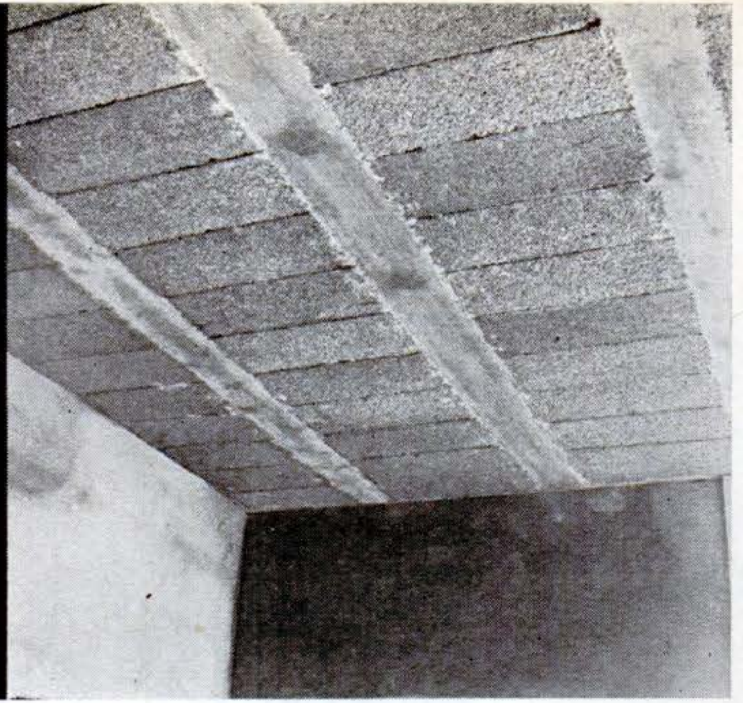
View from underside of floor after shoring was removed. Wood grain and knots in shoring left their imprint in cinder-cement mixture.
