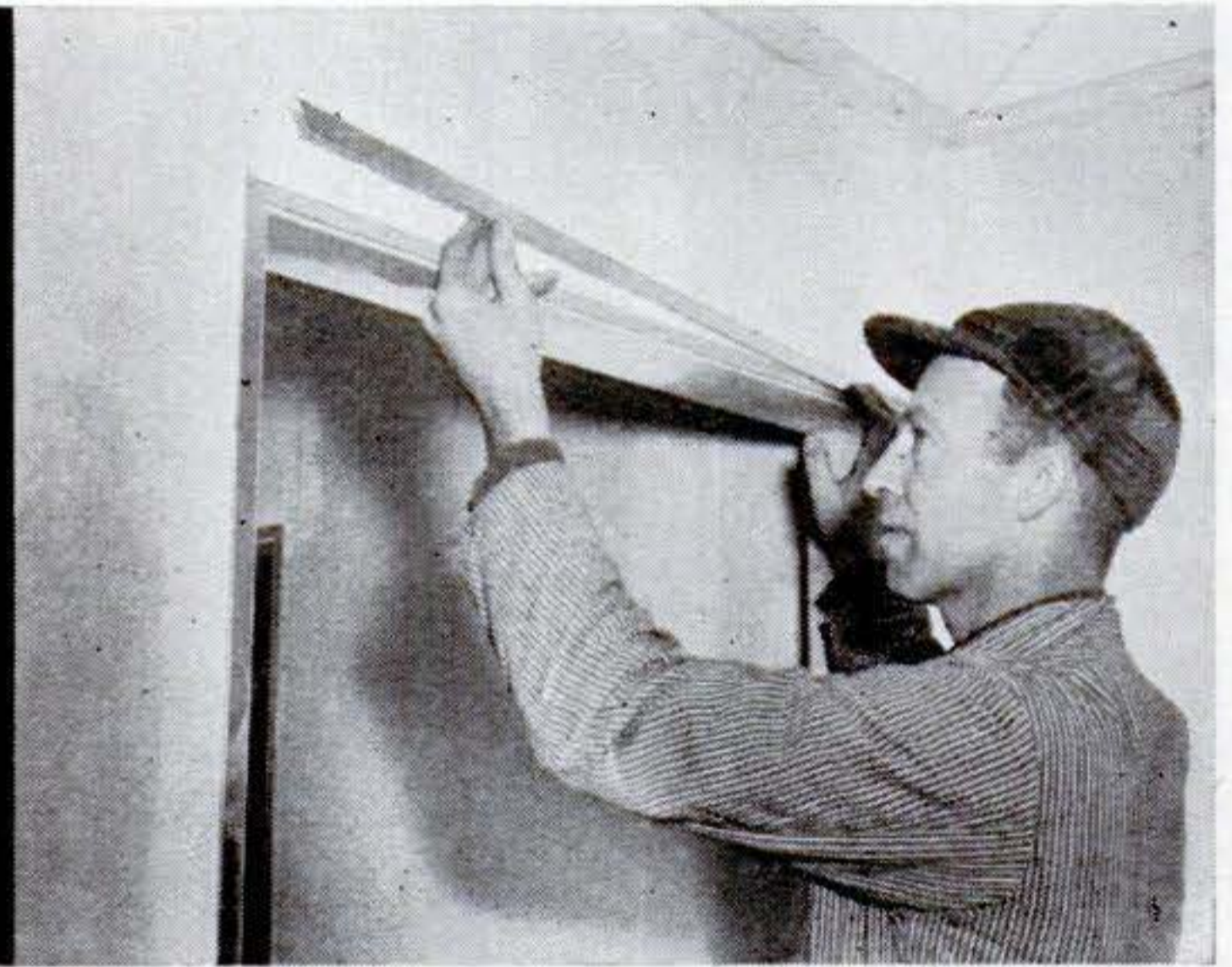
Stainless-steel molding trims all interior doors. Base of two-part molding is screwed to wall. Outer part is then snapped on over base.
