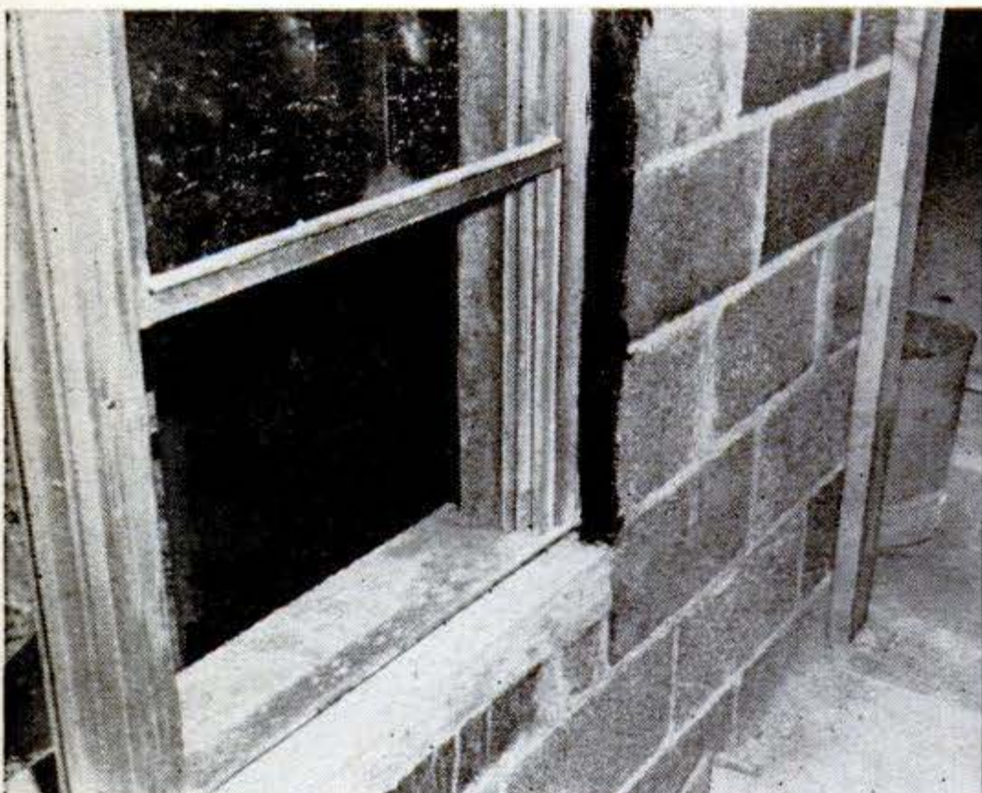
House is fireproof, rotproof, and bugproof. Window sash and frames are aluminum. Photo at left shows window when house was partially
