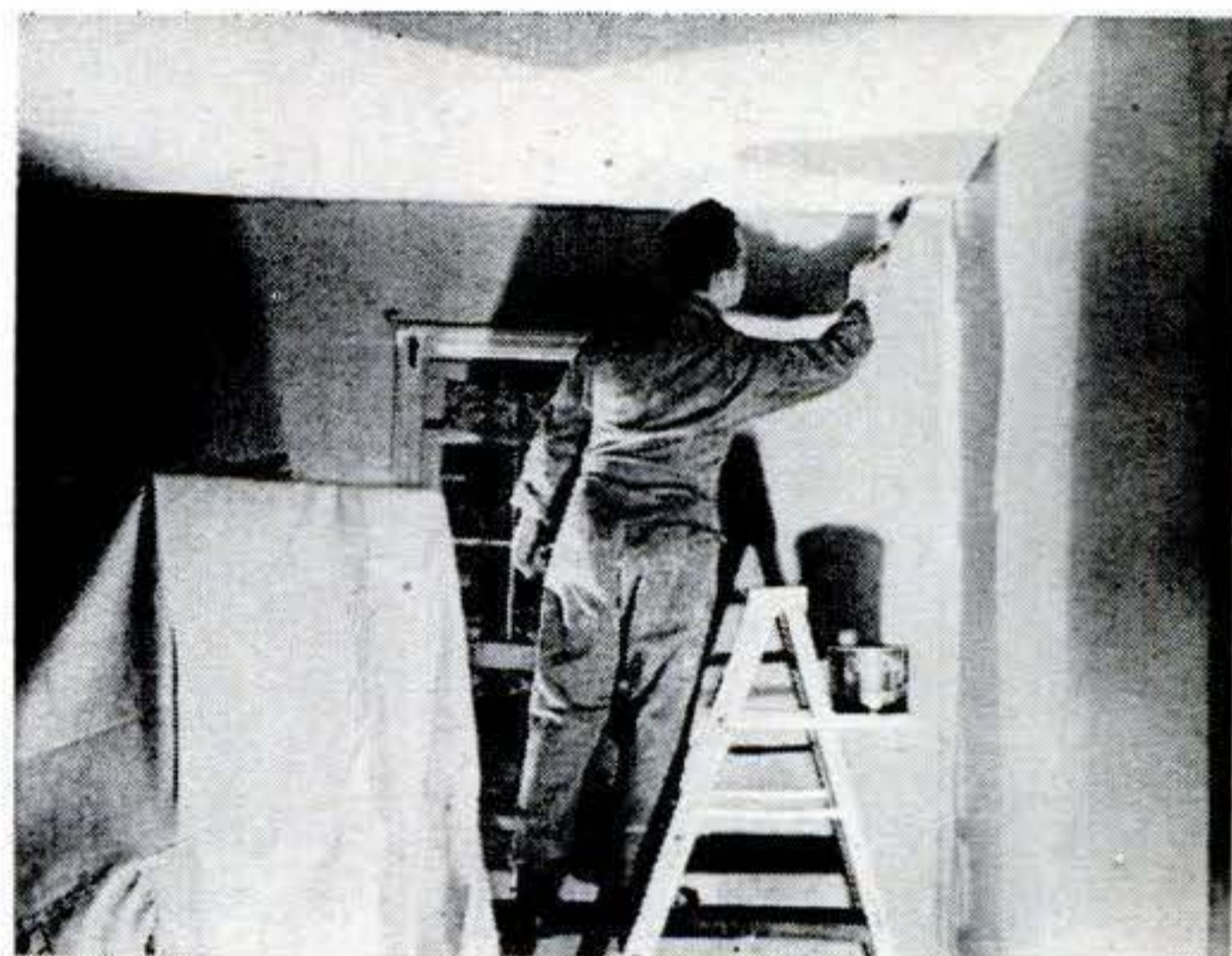
Two stepladders (only one seen here) and stout plank make scaffold for painting ceiling, eliminating extra steps in moving single ladder.
