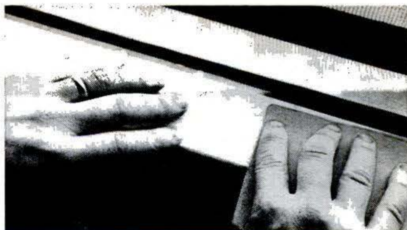
Any rough spots on woodwork should be sanded smooth. Fill all holes and cracks in woodwork with putty and sand smooth when dry.
