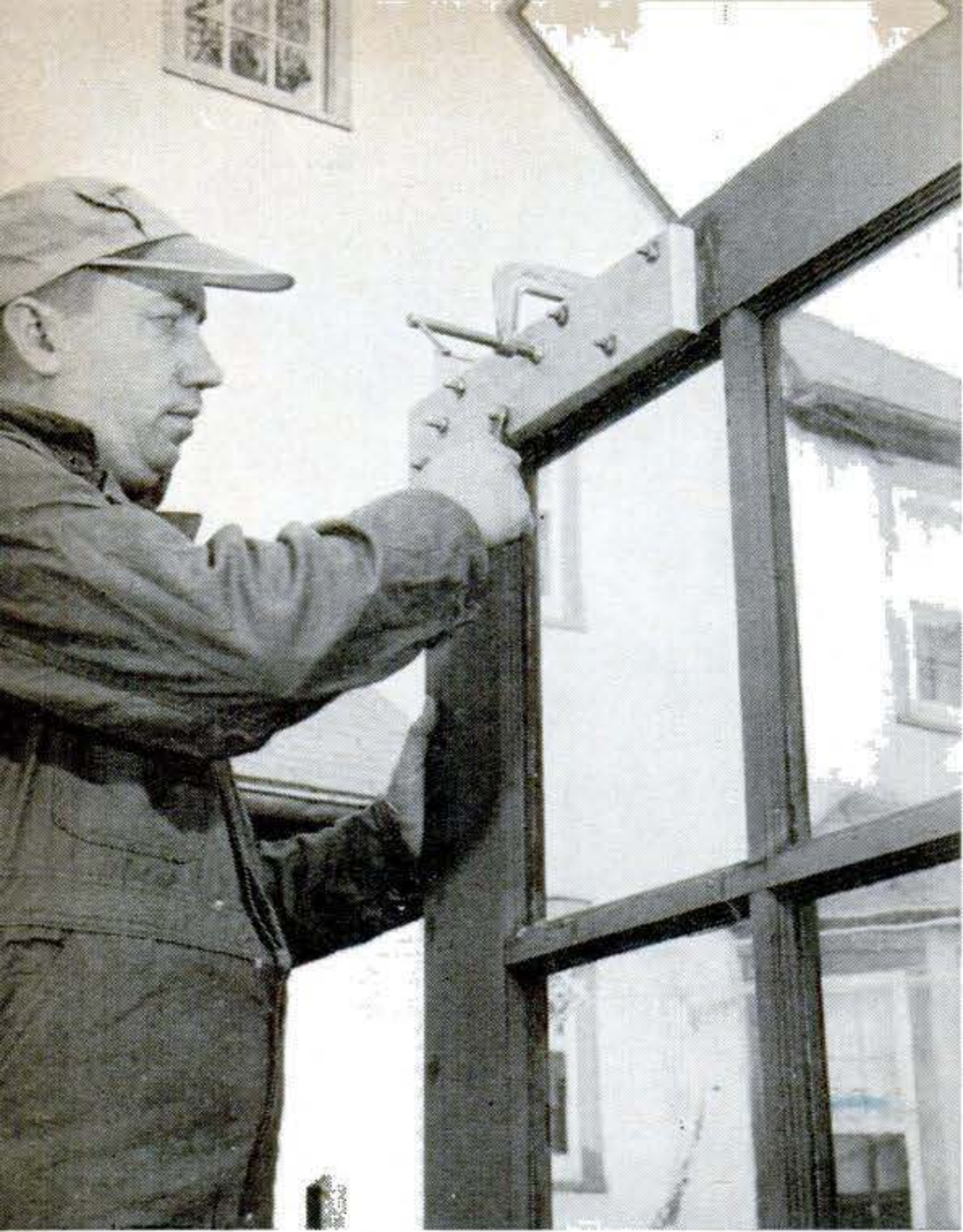
Dowel-repaired joint was reinforced with a batten. Paint was scraped off the door to give glue a good grip, batten was clamped in position, and holes were drilled through. Batten was bolted below rail edge to clear door stop.
