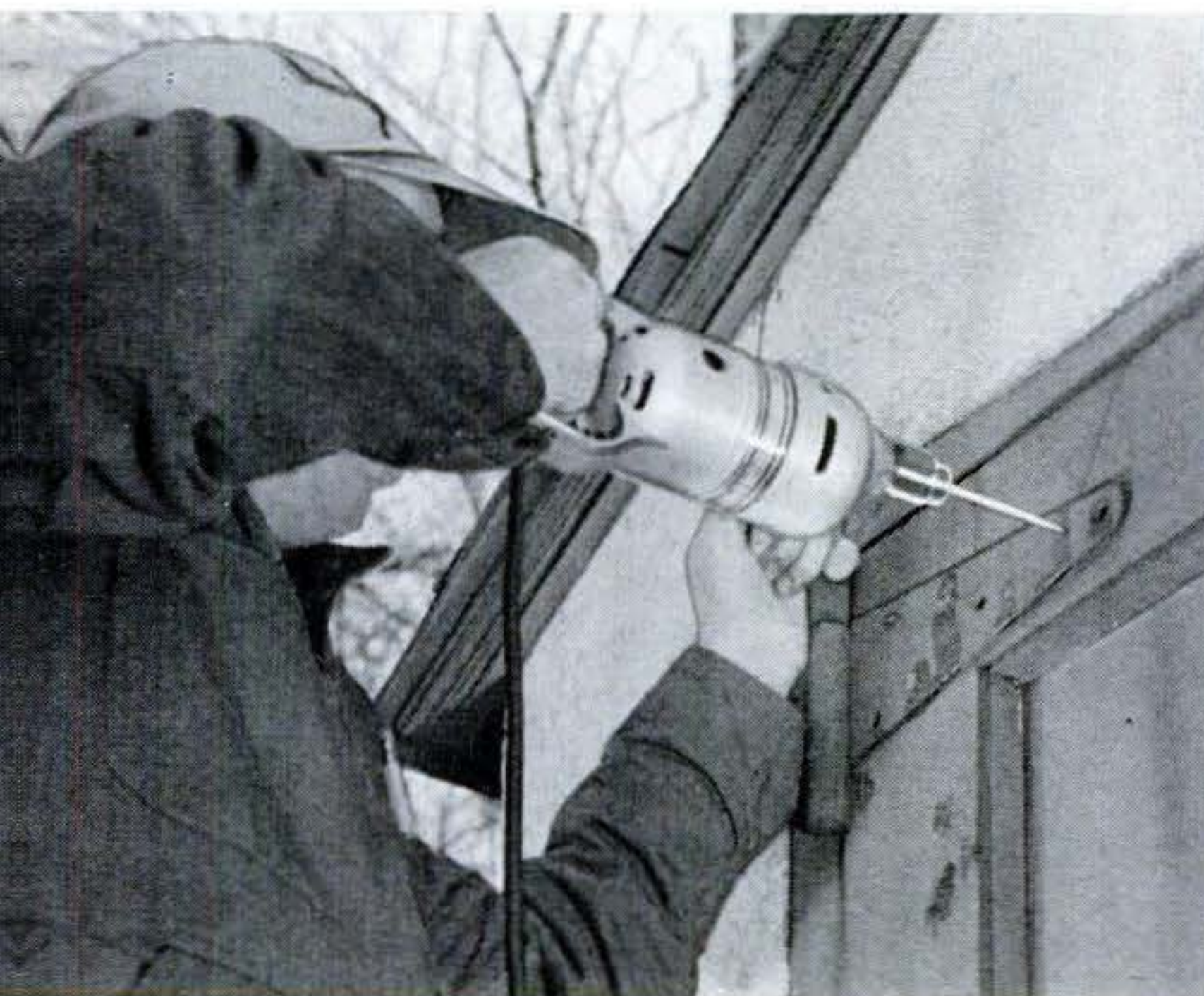
Wood screws in this hinge leaf had rusted loose, leaving holes too enlarged even for bigger screws. Glue was first worked into the open joint. Then the joint was closed with a brace (top right photo). New holes were next drilled
