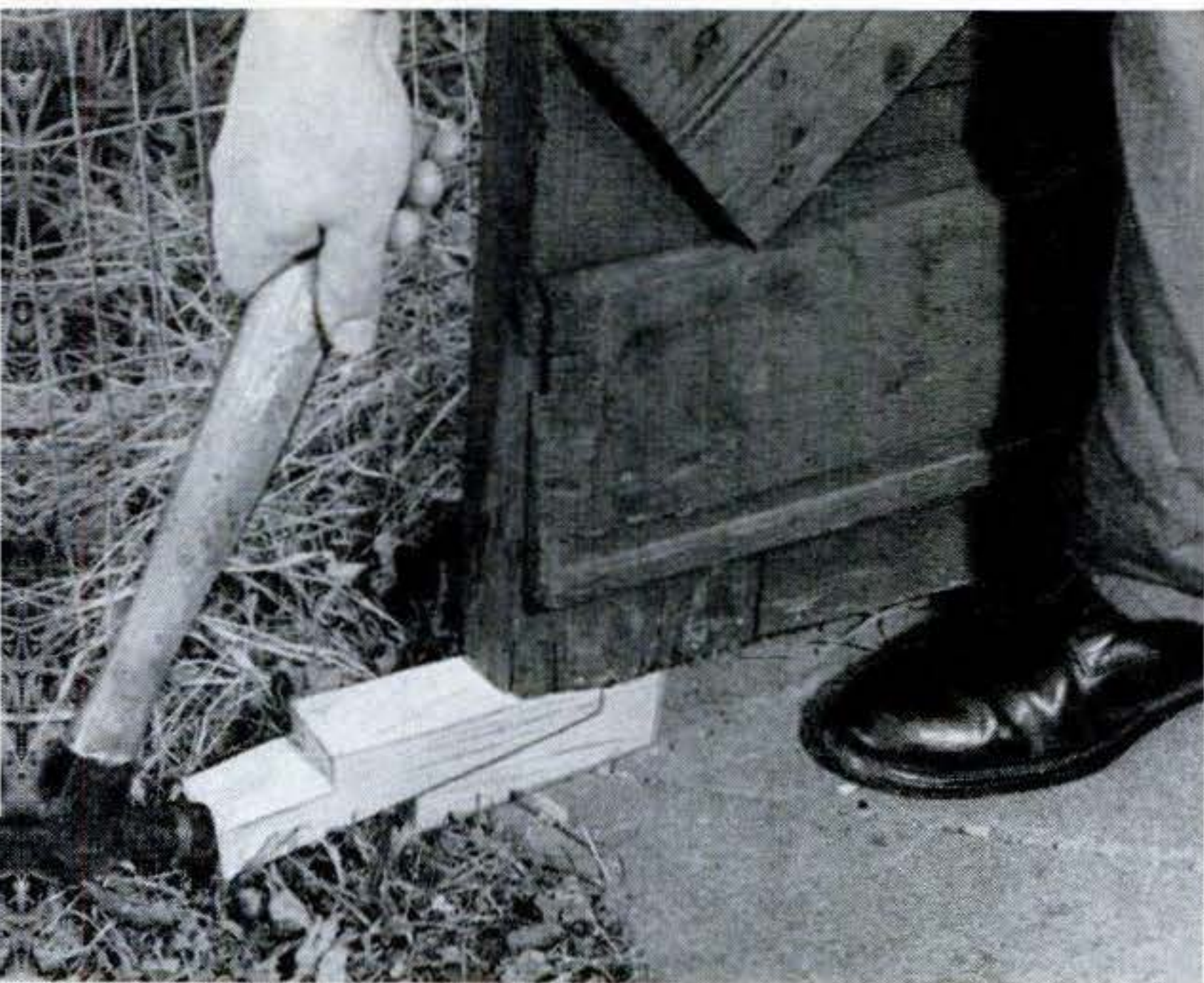
To lift sagging bottom corner, drive in wedges like this. If open top joint doesn't draw together, close the door and drive wedges again.
