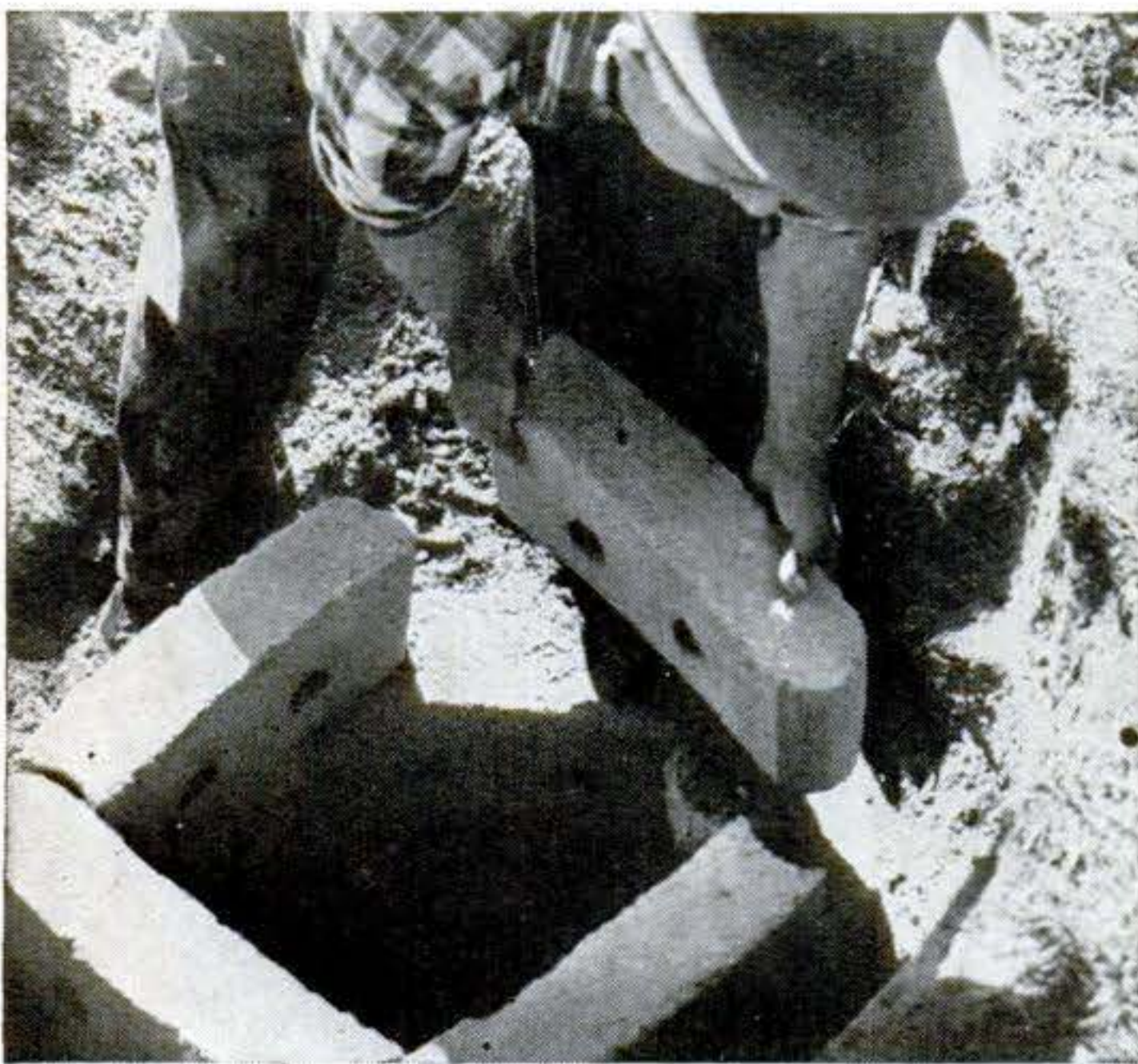
Lay up the blocks in tongue and groove style, giving well a slight conical shape. Fill the space around the outside of well with sand.
