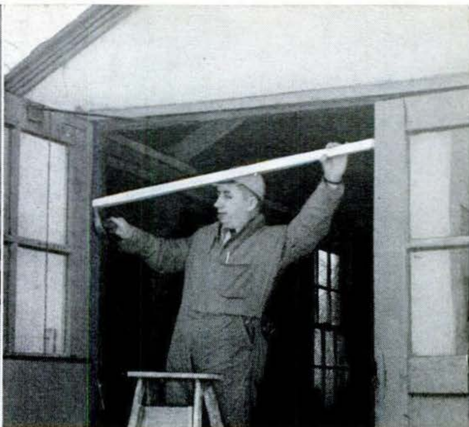
Then insert long prop between the open joint and opposite jamb (above). This will close the joint, but be sure to wedge up the stile too.
