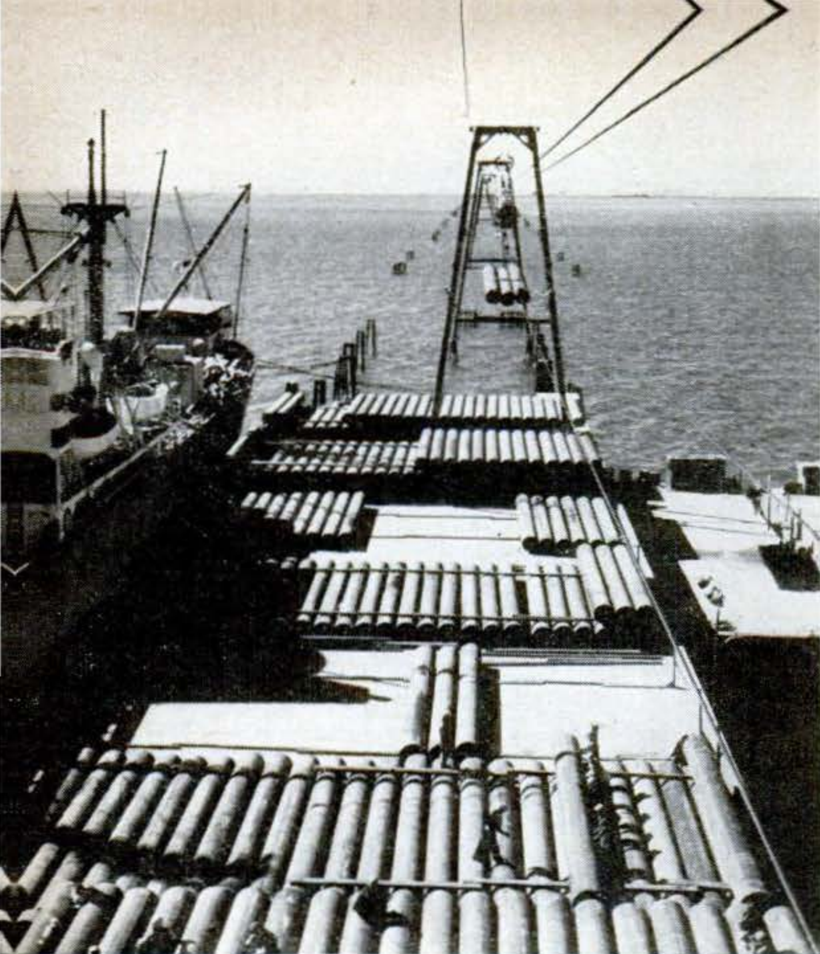
"Skyhook" carries 9 tons of pipe ashore in Saudi Arabia from artificial unloading island built 2\frac{1}{2} miles at sea in Persian Gulf because of shallow water and lack of docks.
