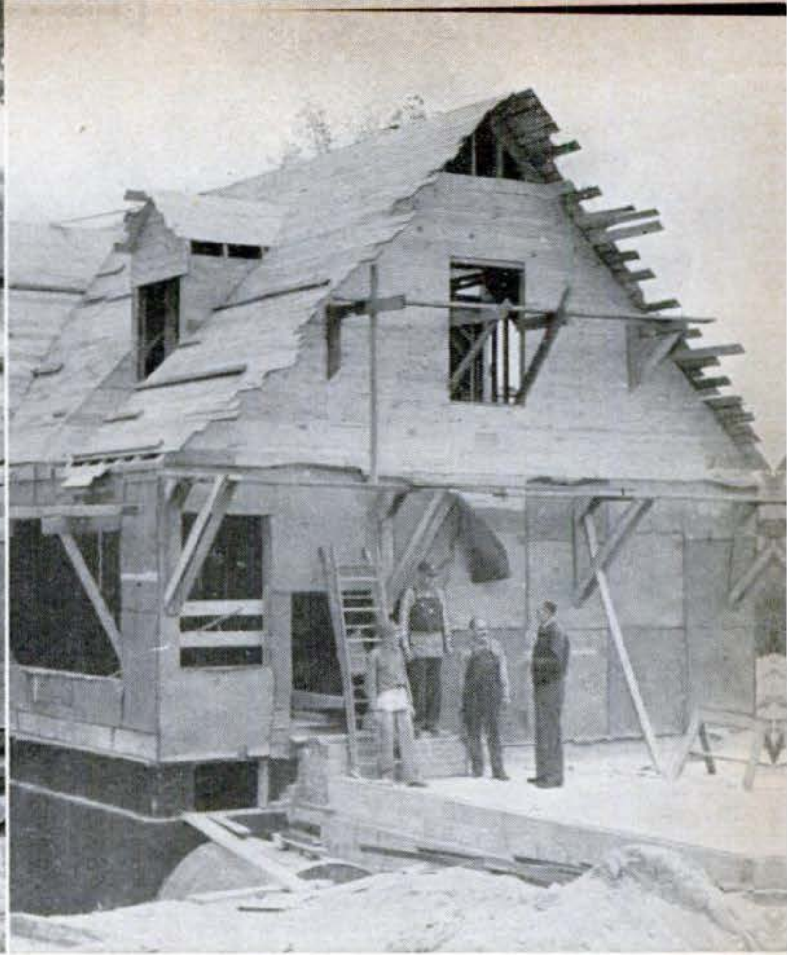
Barenow (in jacket) contracted for and supervised the work his son and he did not do. He used auto deck-lid mats, surplus from 1946 Kaiser car, as an insulating material.
