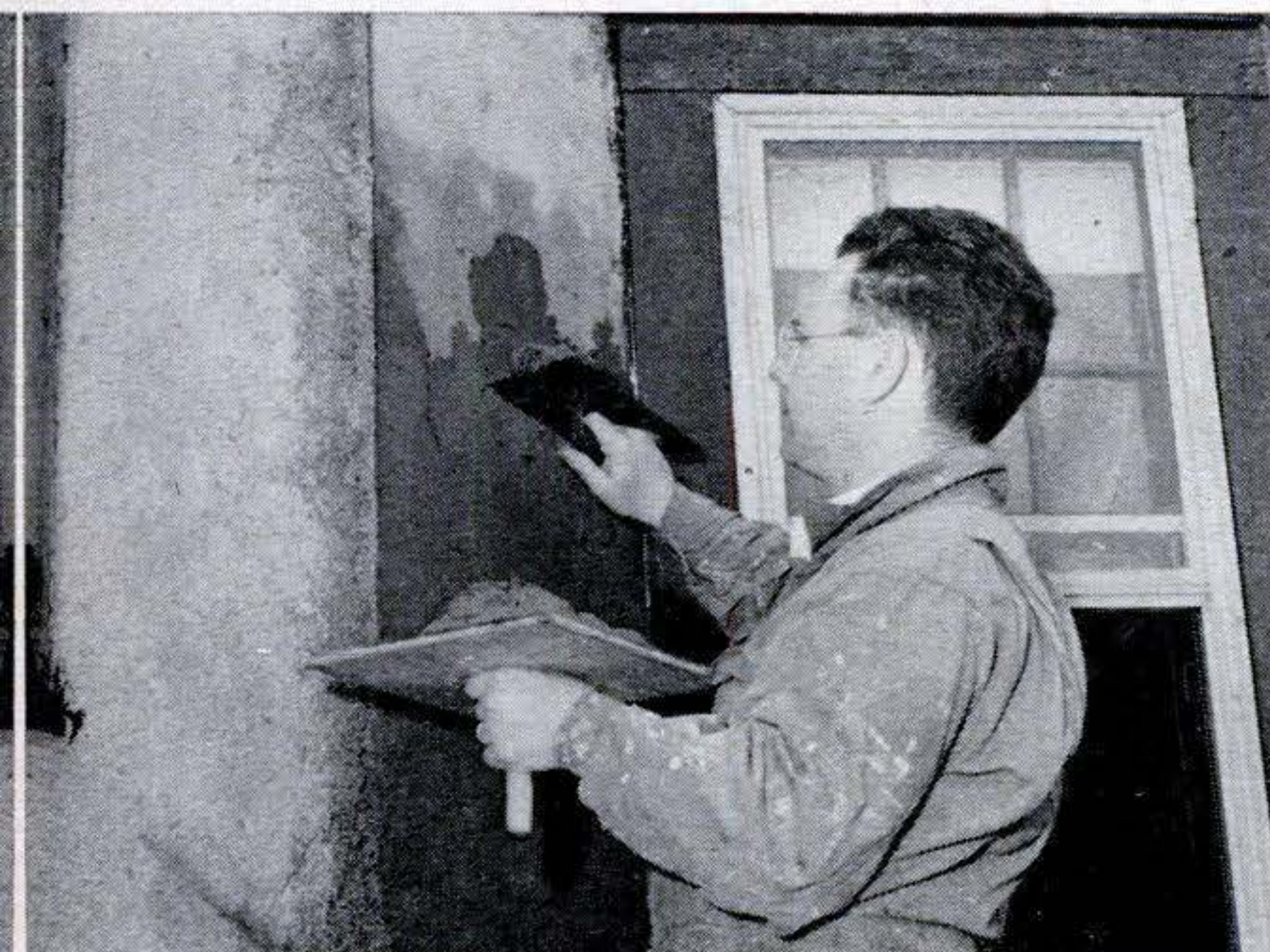
16. Press mortar of second coat firmly against scratch coat to secure a good bond. Build it up to within \frac{1}{4} " of surrounding wall surface.
