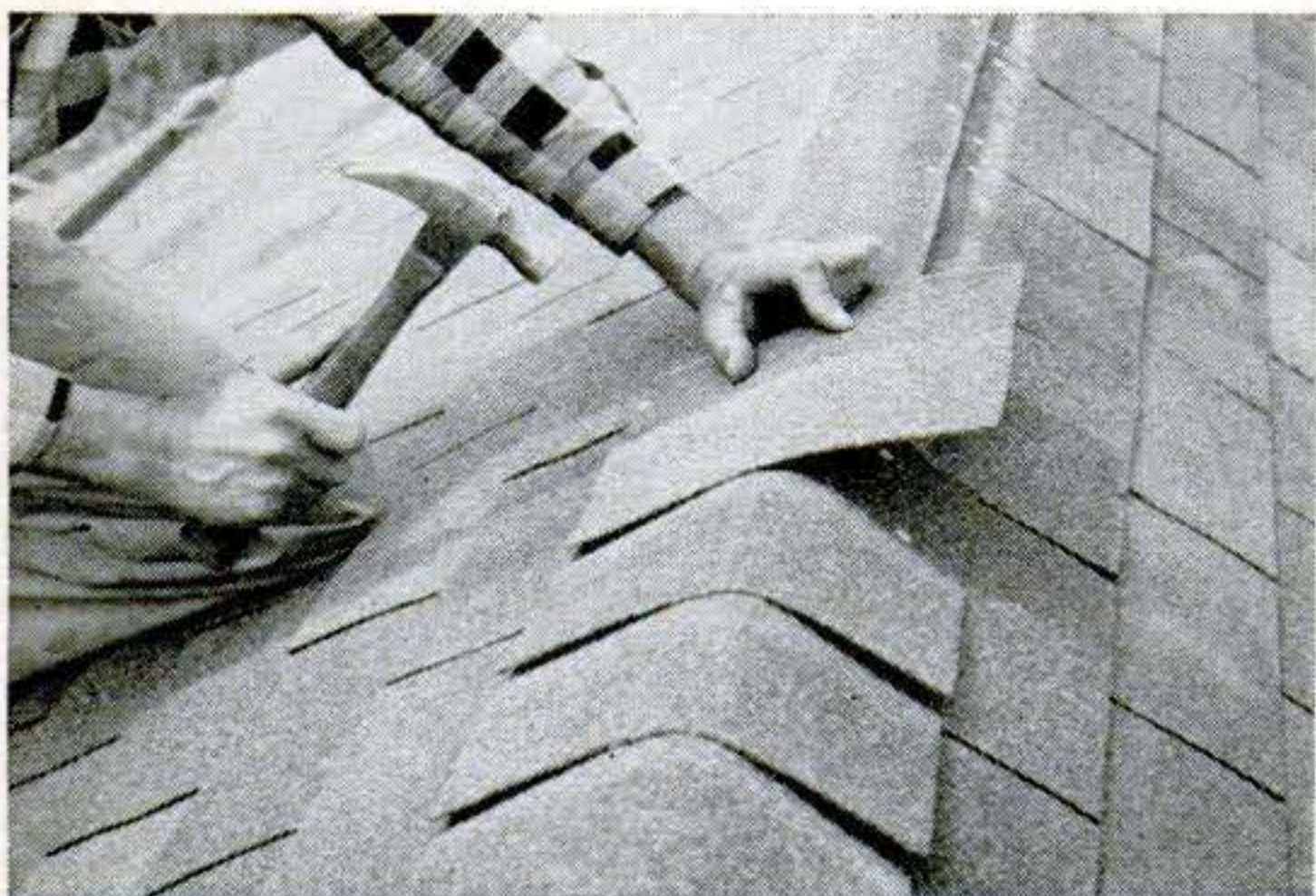
15. Finishing the roof. Cut out squares of composition shingles and lay them over the peak. Standard procedure is to lay the squares halfway from one end of roof peak and then start at the other end and lay squares to meet those you've already laid.
