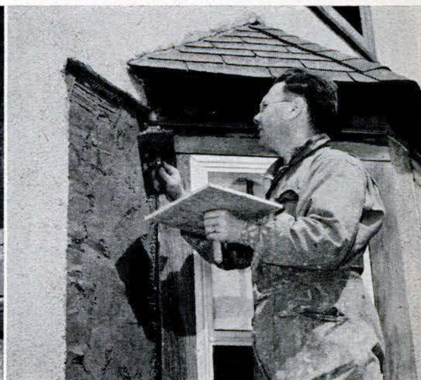
13. First coat should be about \frac{3}{8} " thick. Work it well into corners and along edges. The first coat is called the scratch coat.
