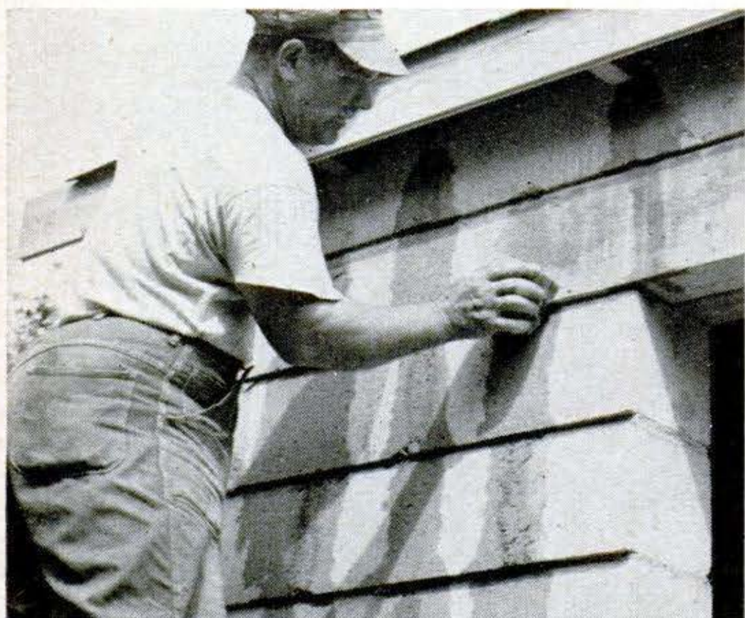
19. Preparing to paint. Joints between blocks must be smoothed before painting. Mix mortar and sand in equal amounts. Add water to make workable mixture. Wet joints, apply mortar and scrub with brick until joint is flush.
