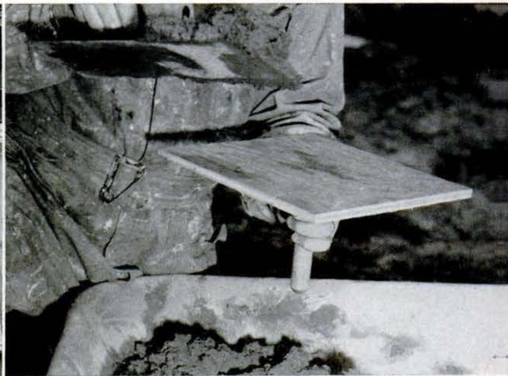
11. To carry mortar from the mixing pan to the job, you'll need a hawk. A 10" square of plywood with a broomstick handle will do.
