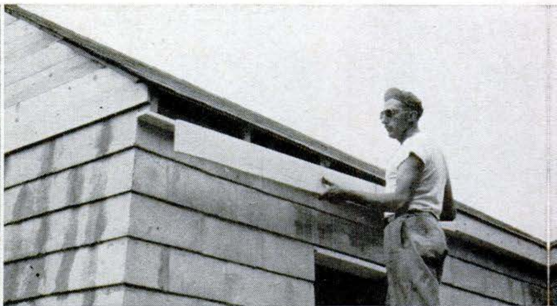
16. Installing trim. Ends of rafters on each side of garage are boxed in with trim. Trim boards on ends of garage lap over ends of side-trim boards. Fasten trim to ends of rafters with finishing nails. Set the nailheads and putty over them before painting.
