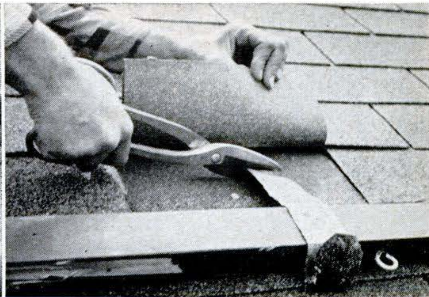
14. Removing toeboards. Lay shingles right over the tin strip. When you no longer need toeboard, bend up the shingle covering the tin. Snip the tin strip up under the shingle. Then the toeboard can be lifted off roof. Let the small piece of tin remain under shingle.
