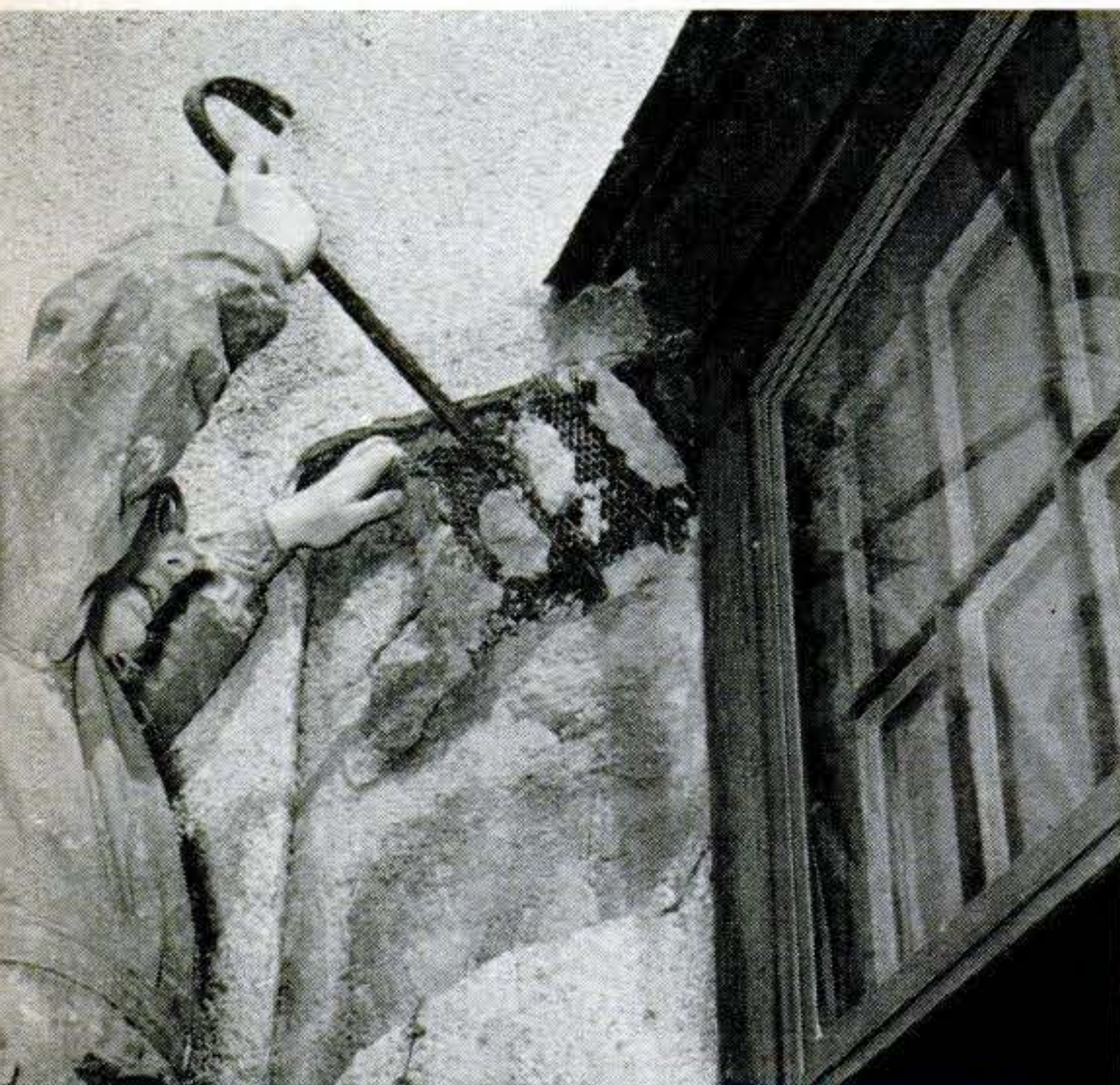
2. If lath has rusted from water seepage, it must be removed and replaced. A ripping bar is handy for this part of the job.
