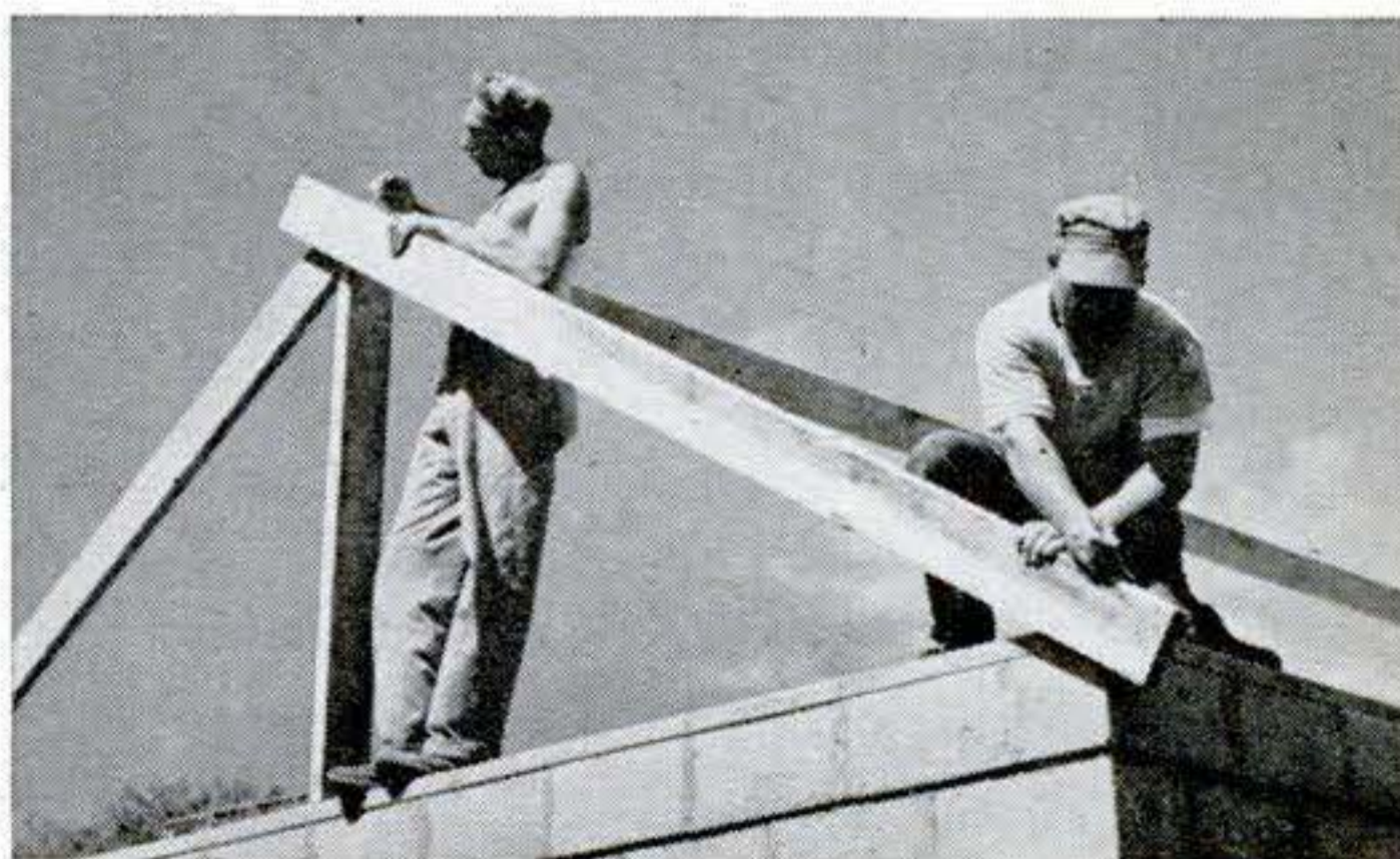
3. Marking rafter template. With ridge pole in place, mark a rafter for notch where it fits plate and for angle cut where it meets ridge pole. Notched end is trimmed to make it vertical. Drawing shows dimensions of rafters.
