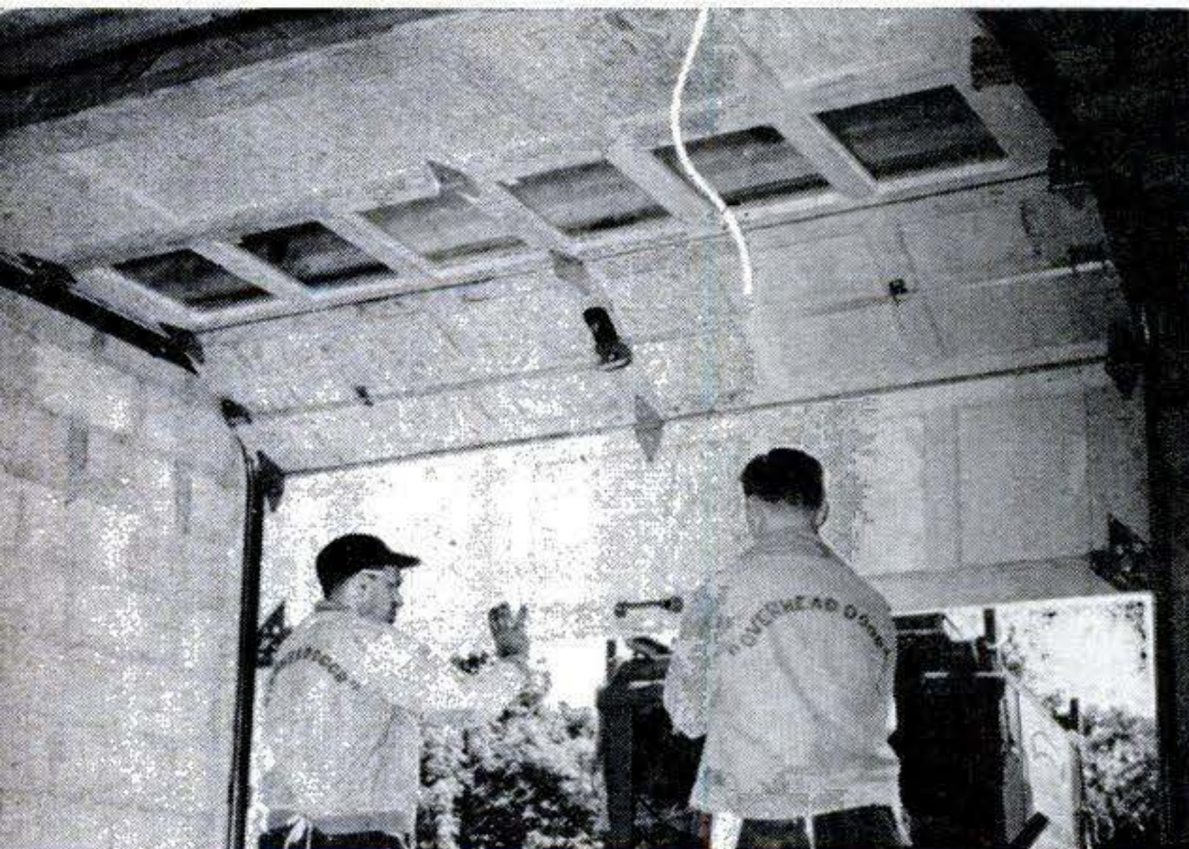
21. Installing main door. The kind that swings or slides up is best for a garage. You can install this type yourself by following the manufacturer's instructions. However, to cut costs, you can build hinged doors for your garage.
