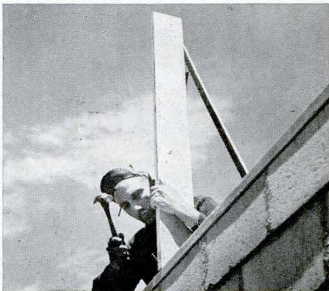
2. Supporting ridge pole. Find centers of end plates and nail two-by-six verticals there. These will support ridge pole. Nail on temporary braces until ridge pole and rafters stiffen structure. If you don't have a two-by-six long enough for ridge pole, join two with scarf joint, as in drawing on next page.
