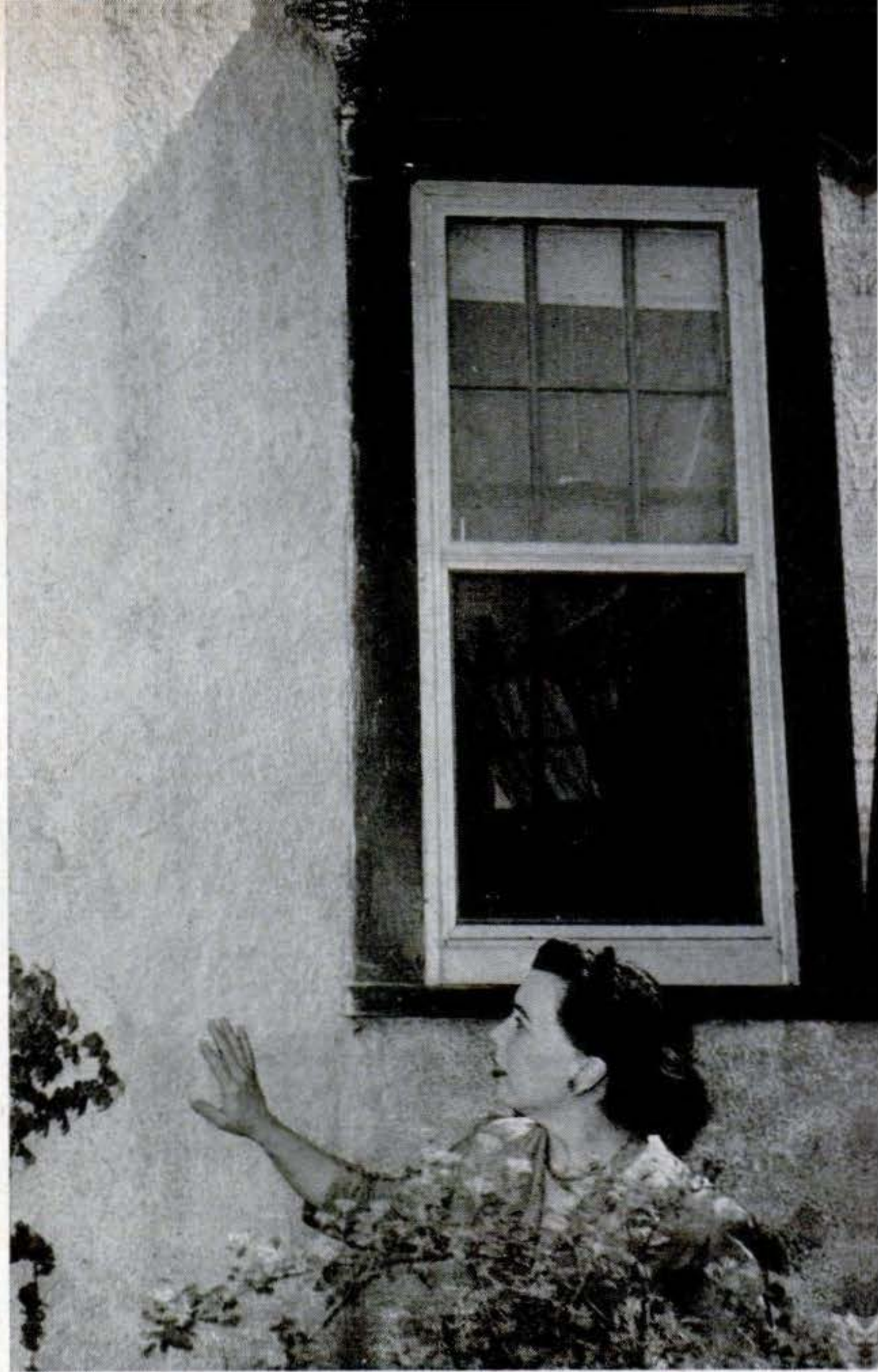
20. Finished patch, when dry, closely resembles old stucco surrounding it. When working near window or door frames, mask them.
