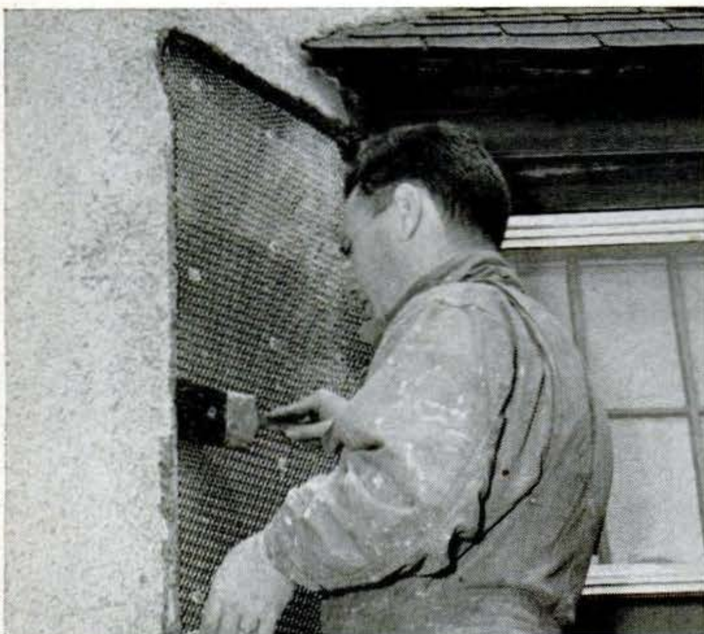
10. Soak old stucco thoroughly along edges of patch area before troweling on mortar. An old paintbrush is handy for applying water.
