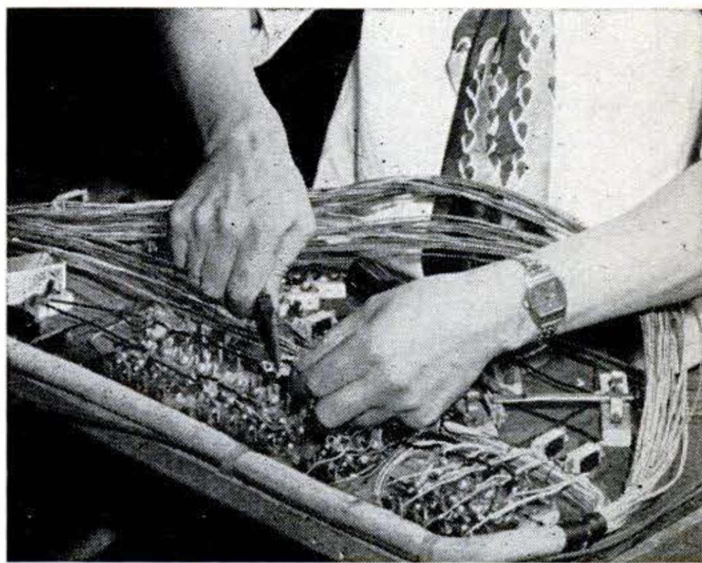
Maze of wires , some of the hundreds that supply power and operate switches, connects tracks with control station. Connections are made on huge terminal strips to simplify maintenance.
