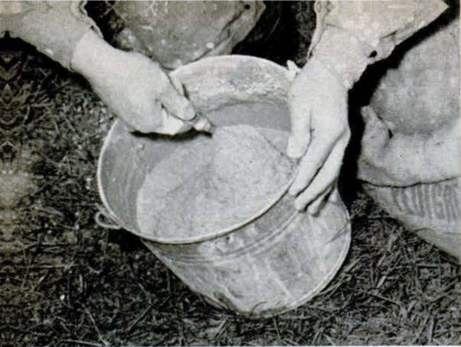
18. To match spatter-dash finish of this house, enough water and lime were added to the cement-sand mix to bring it to a creamy consistency.
