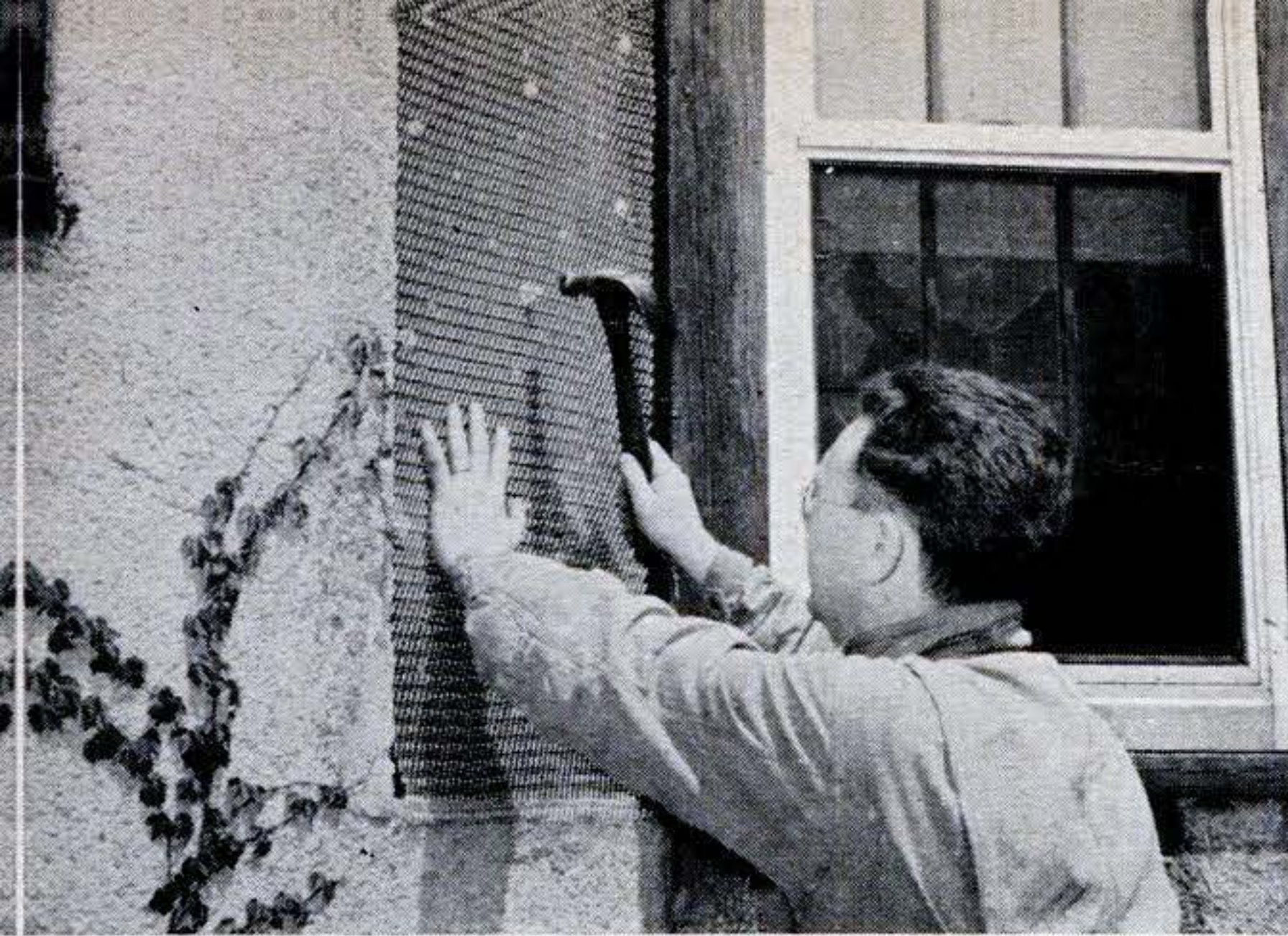
8. Fasten mesh over washers with large-headed galvanized nails. The brads through centers of washers leave enough room for nails.
