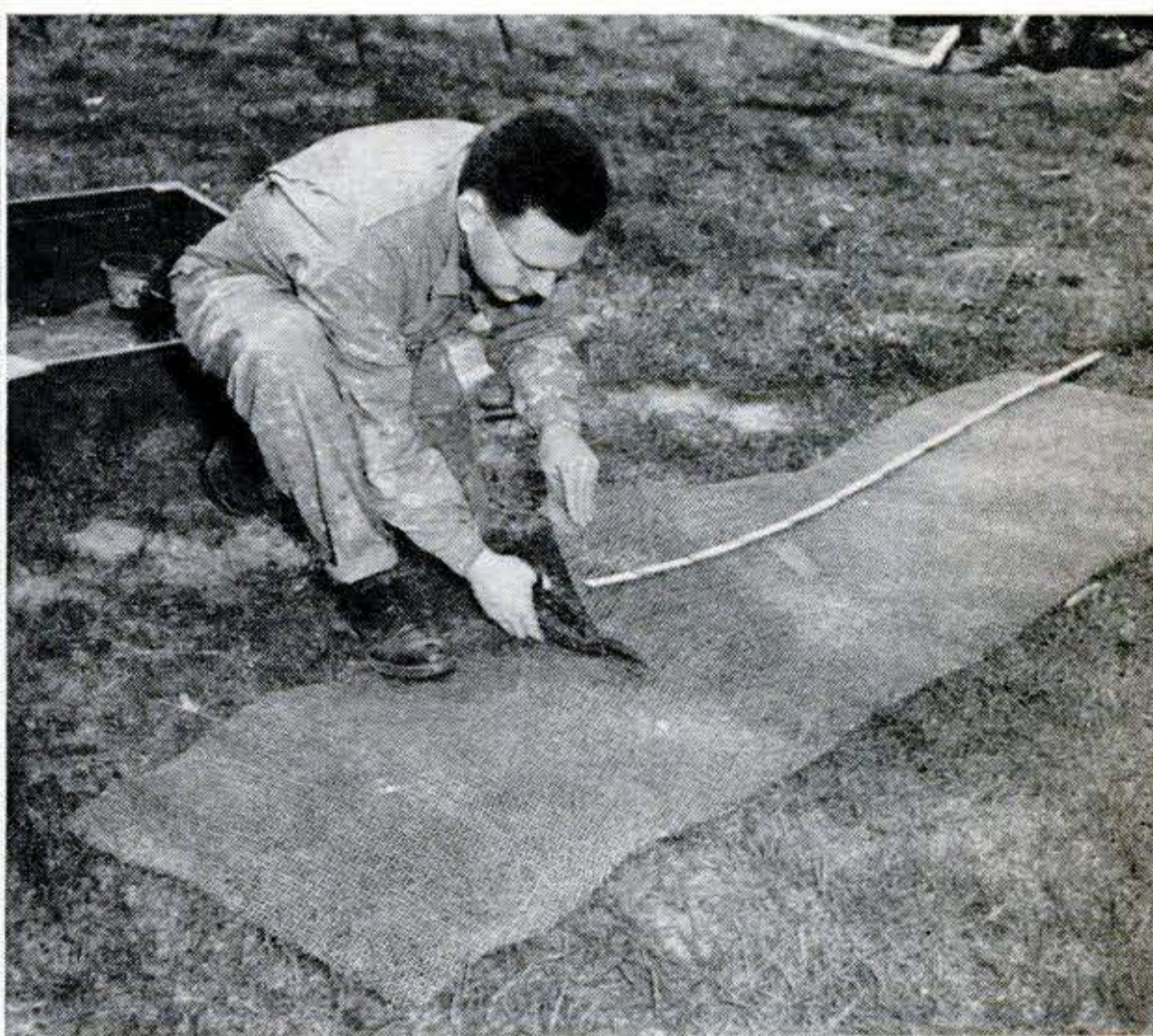
5. Wire lath goes on over the building paper. Use rustproof diamond-mesh lath. Cut piece to exact size so it fits snugly in patch area.
