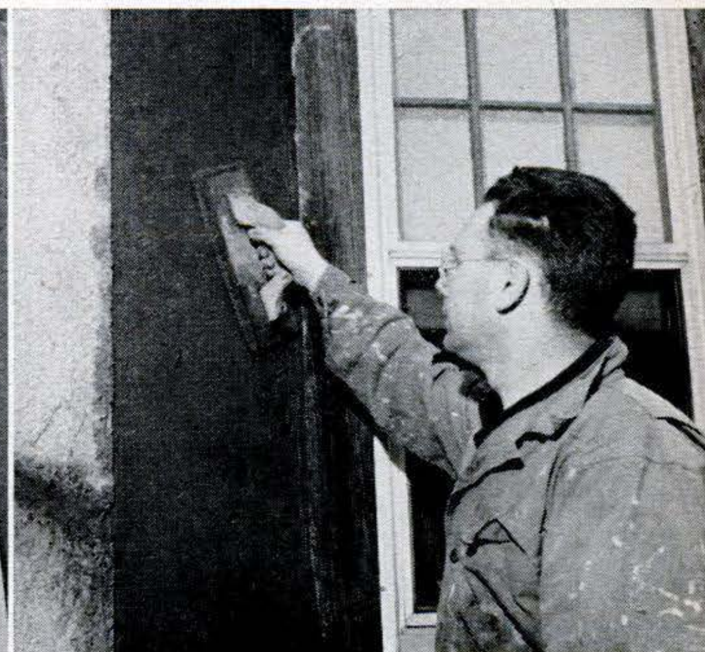
17. When second coat stiffens , go over the surface with a wooden float. Work with a circular motion. [Continued on next page]
