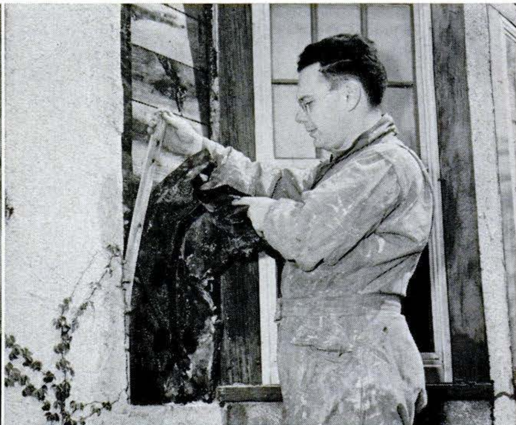
3. The old building paper may have deteriorated. Remove this paper and any furring strips that may have been nailed over it.
