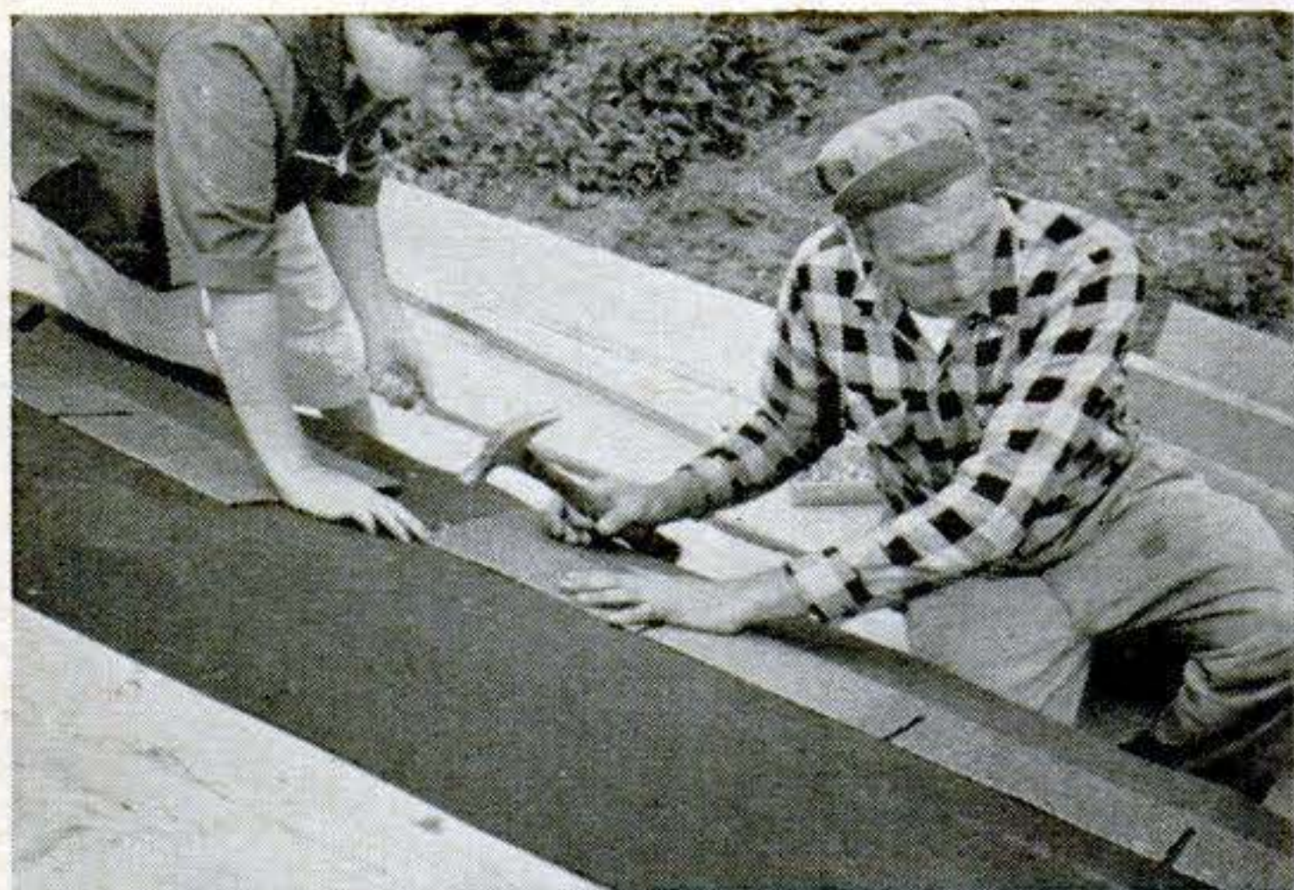
11. Laying drip-course shingles. Fasten roofing paper to sheathing with large-headed roofing nails. Then put down drip course of composition shingles. Lay drip-course shingles reversed—with tabs pointing toward roof peak and with straight edges overhanging eaves \frac{1}{2} ".
