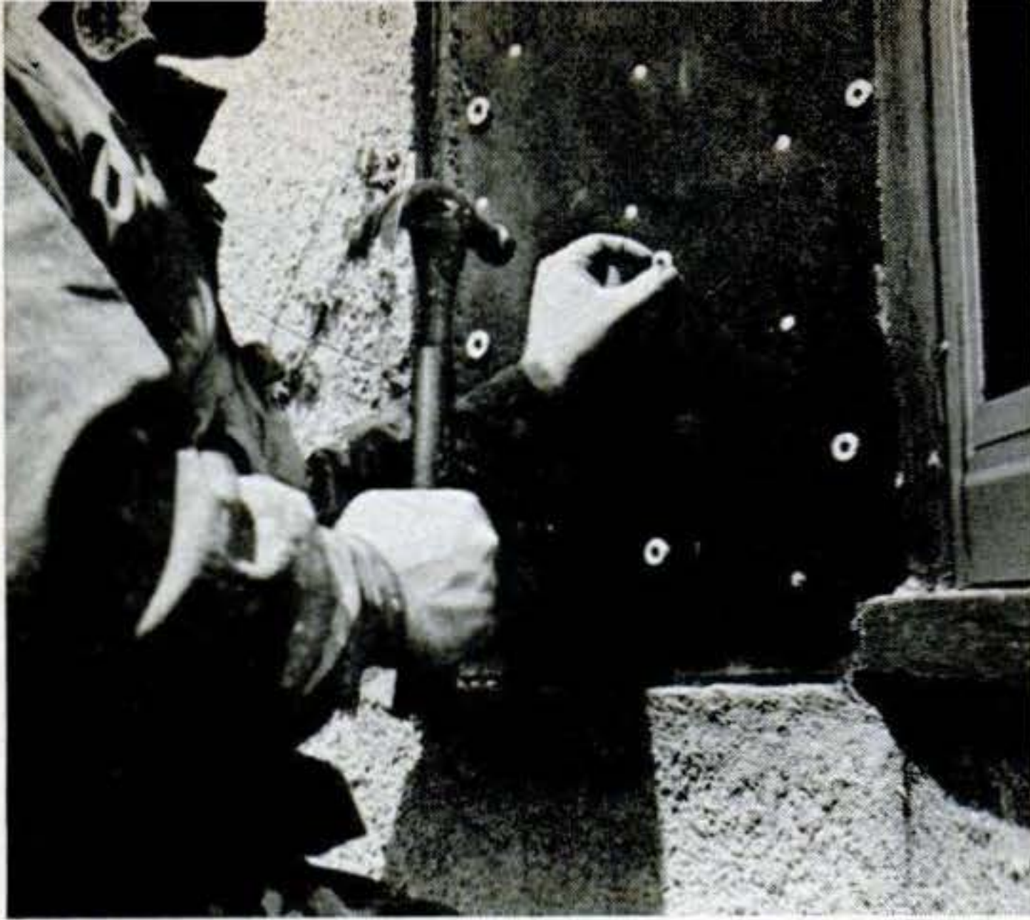
6. Don't nail lath flat against wall. If you have no furring nails, brad galvanized washers (above) to wall as furring points.
