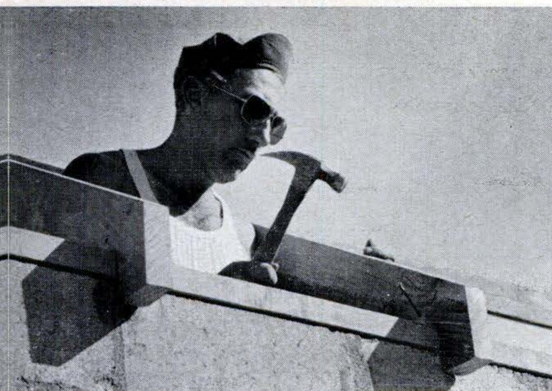
6. Nailing rafters to plates. Before nailing down rafters, measure to be sure they will be properly spaced. Drawing shows correct spacing. Drive nails in from side of rafters.
