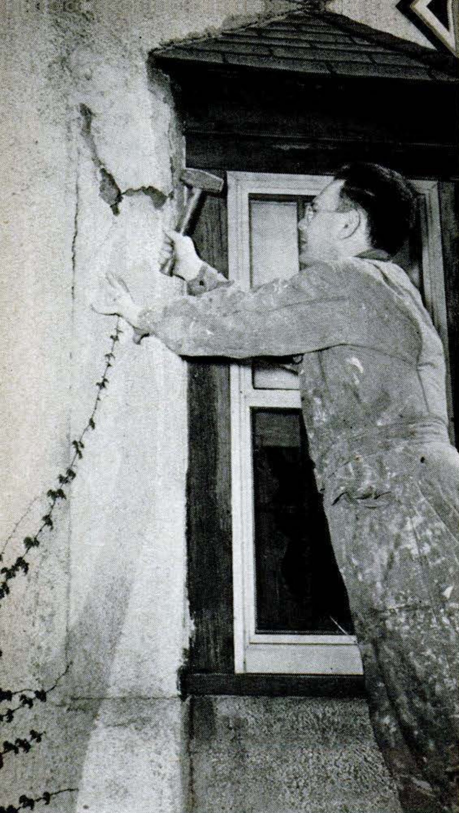
1. This old patch has started to bulge and crumble. Only solution is to knock out loose, cracked or crumbling mortar, and replace it.
