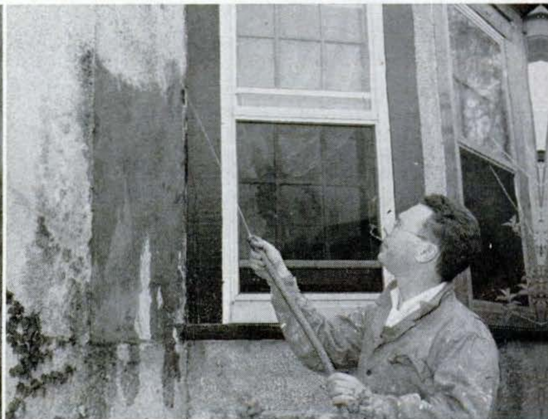
15. Wet down scratch coat thoroughly after it has dried and hardened for two days. Then put on second coat—sometimes called "brown" coat.
