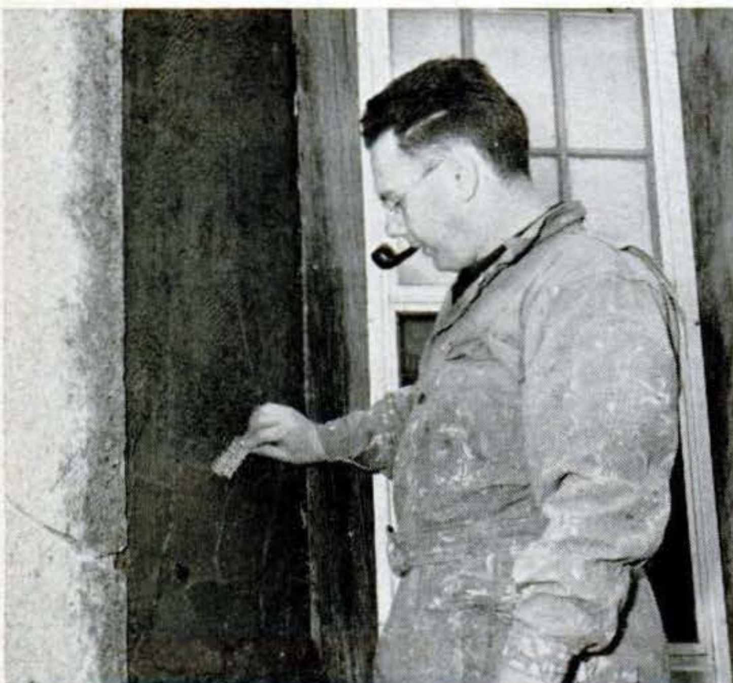
14. Cross-scratch the surface before it hardens, using a scrap of wire mesh. This operation gives the scratch coat its name.
