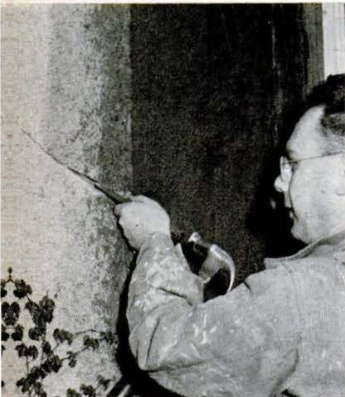
Undercut the sides of the crack so the crack is wider at the bottom than at the top. Use a hammer and a stone or cold chisel.
