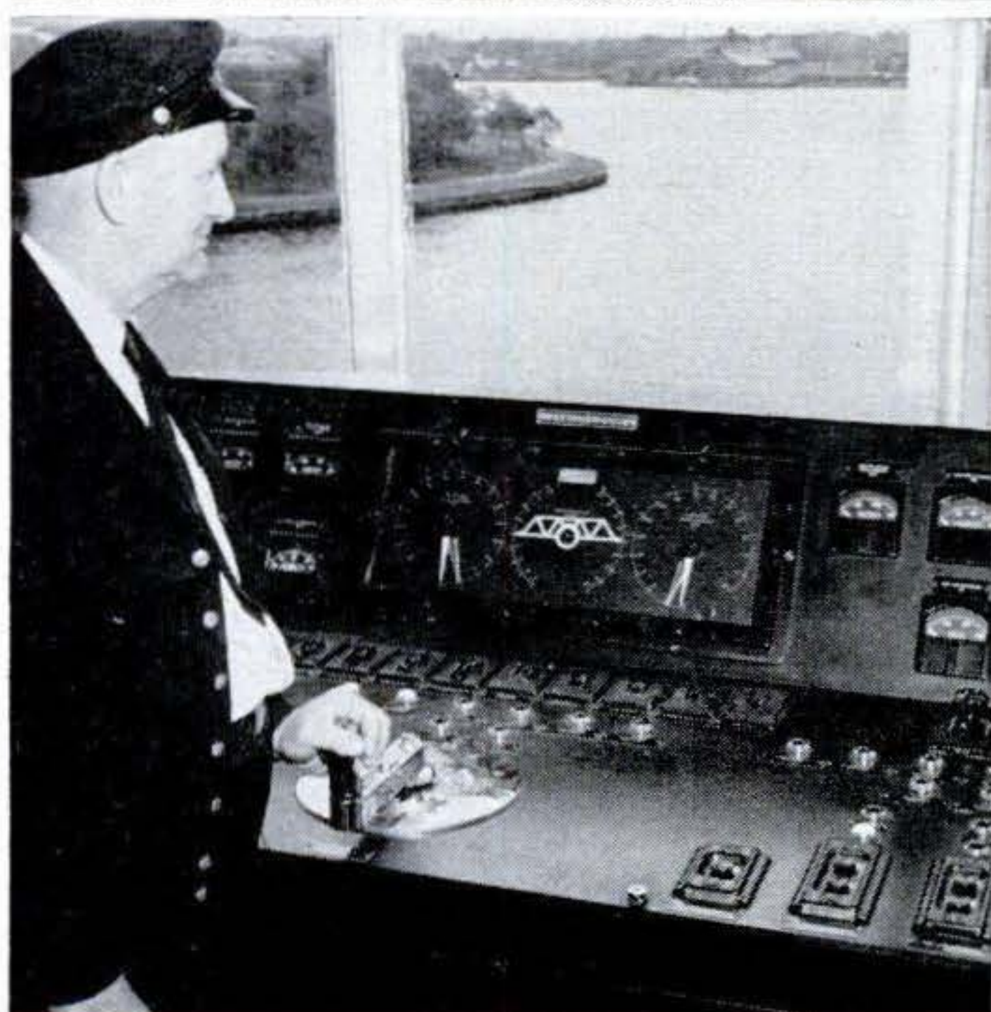
Control handle raises and lowers span. Center dial in background registers span tilt. Dials on either side show height of each end of span.
