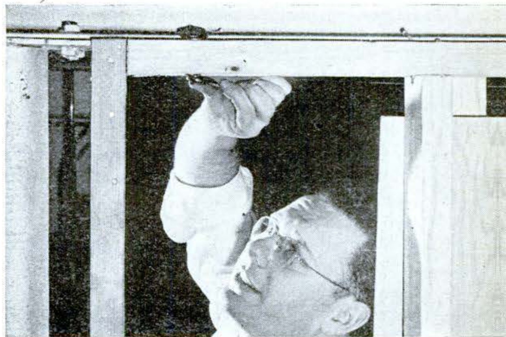
BOLTS through plate are another method of holding it to I beam. Use large washers under nut so they overlap flange.
