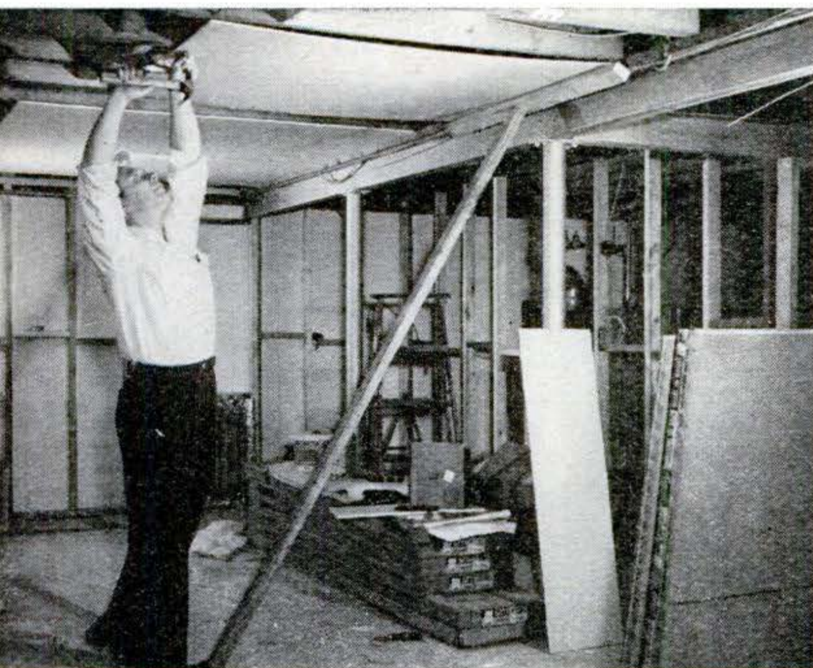
SHEETS of plasterboard can be nailed overhead by one man with the help of a T made of two-by-threes to hold up one end of sheet.
