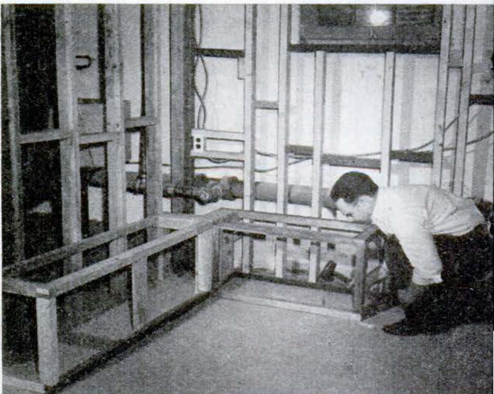
BUILT-IN BENCHES flank corner table. Screws and angle bracket tie framework together. Cut steel nails anchor bottom pieces to floor.
