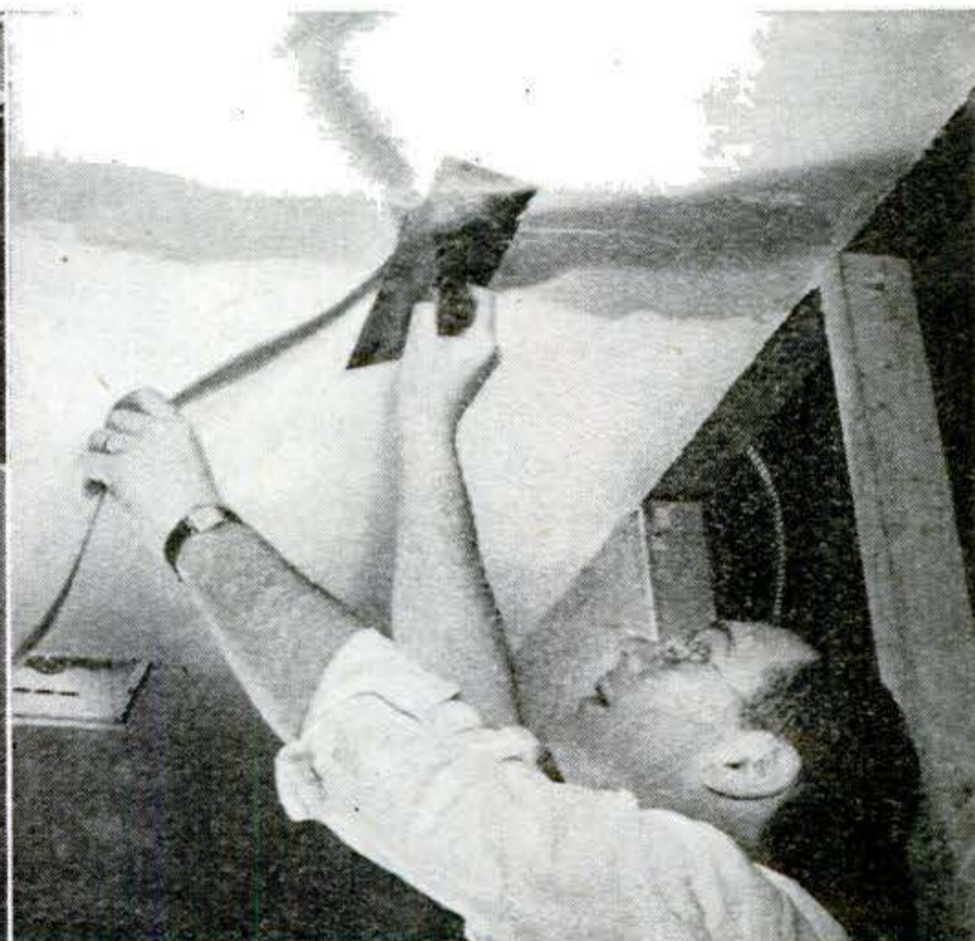
TAPE AND CEMENT cover plasterboard joints. Cement is spread along joint and tape pressed over it. More cement covers the tape.
