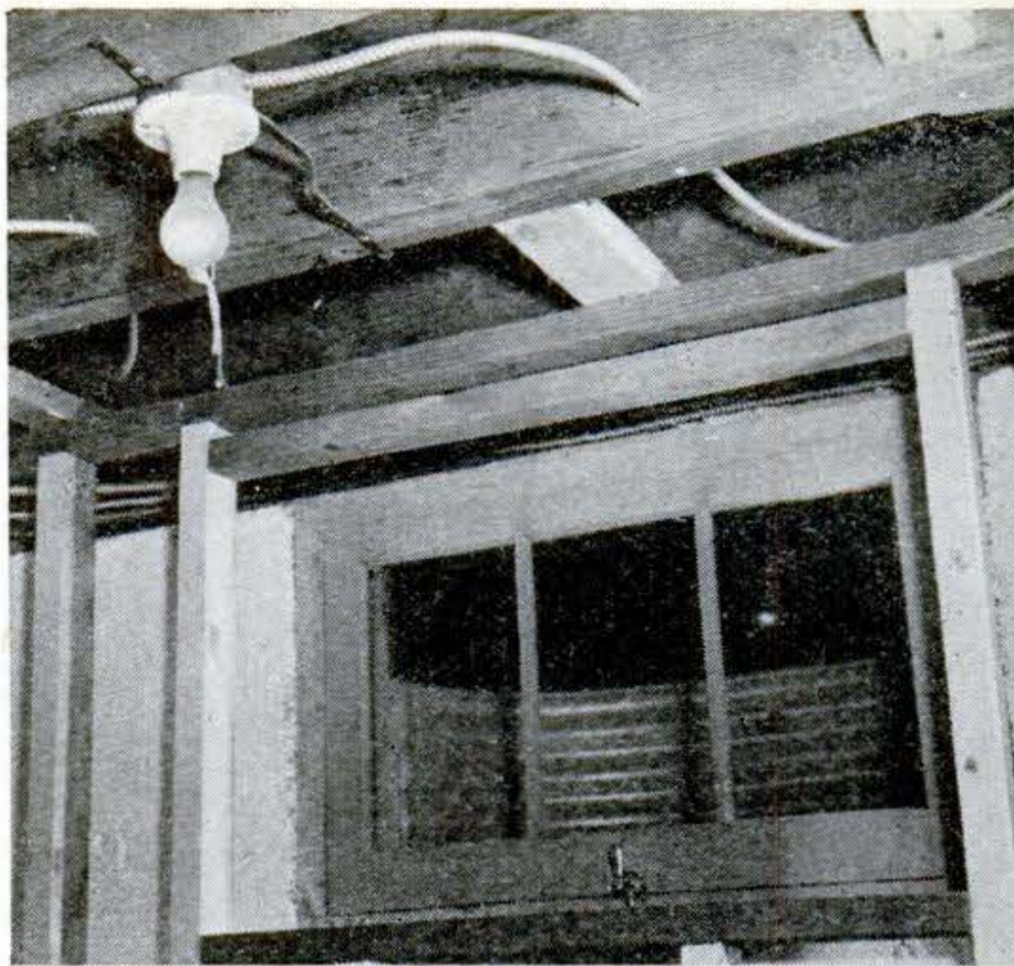
PLATES that parallel but fall between joists can be secured by nailing them to short pieces that have been spiked between joists.
