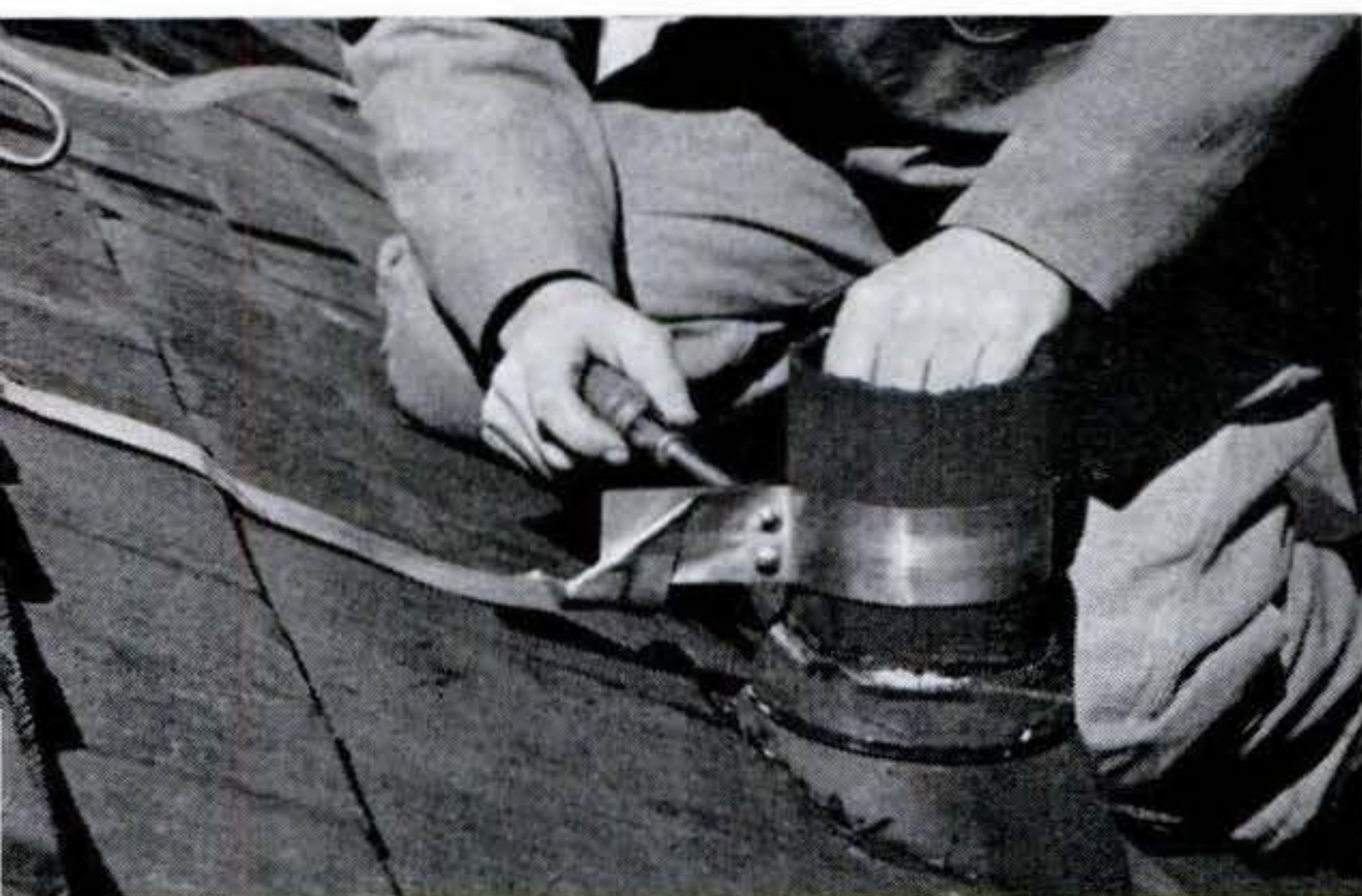
7 ROOF VENT is interconnected, or "cross-bonded," too. Metal like this acts as lightning rod but would carry charge into house.
