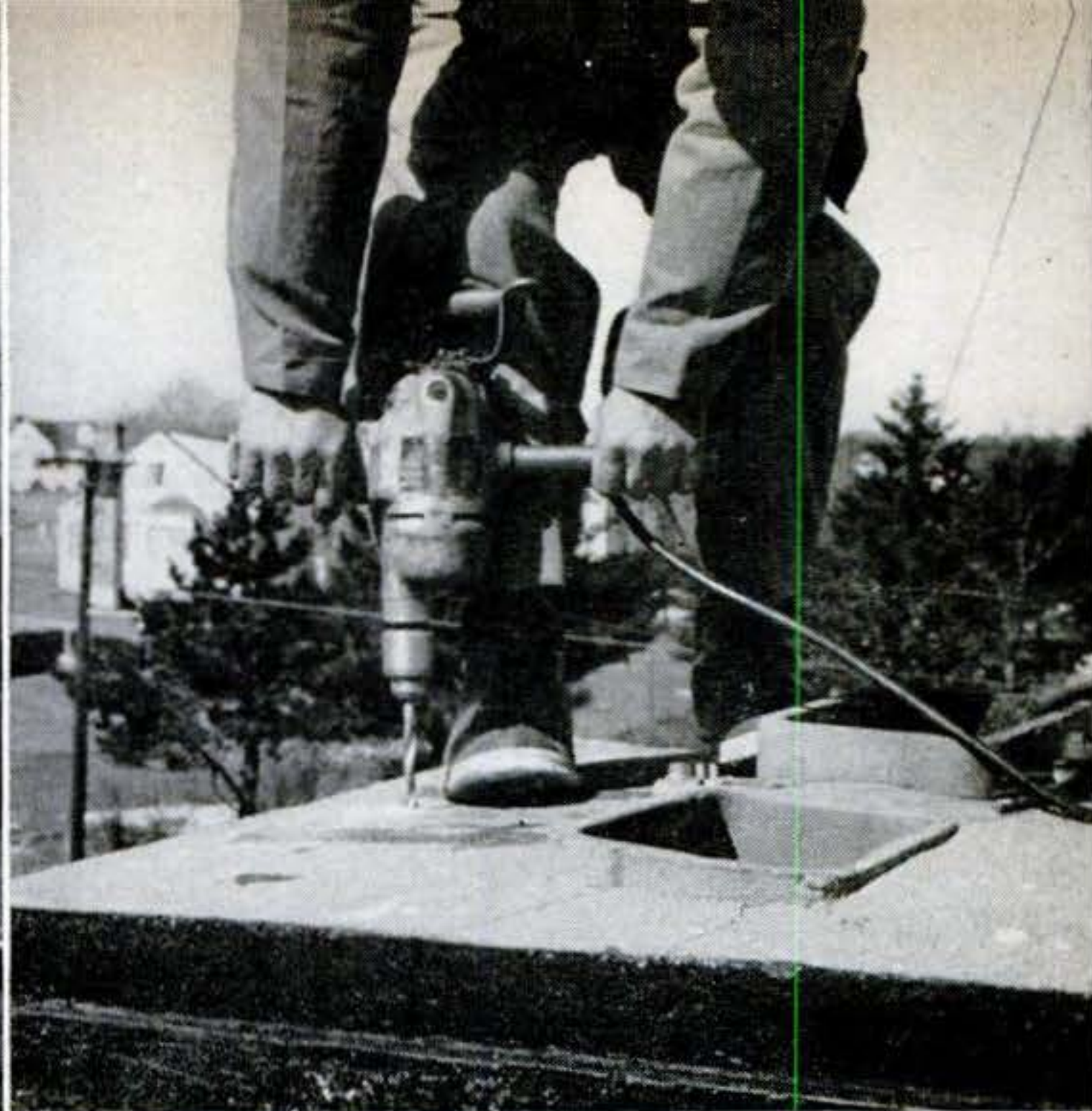
4 CHIMNEY IS DRILLED for lead anchors that hold masonry saddle. Chimneys, favorite lightning targets, are always rodded.
