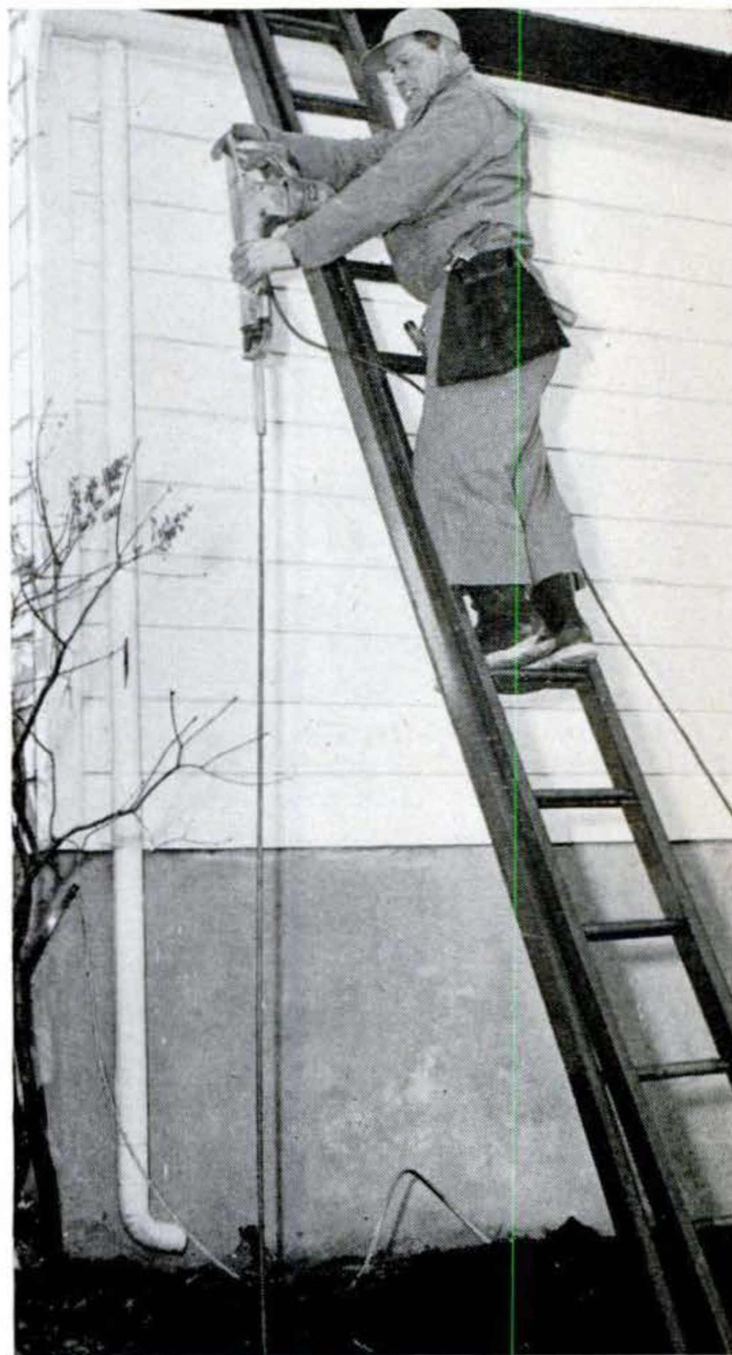
11 GROUND BAR , a 10-foot copper rod, is driven with an electric hammer. It is joined to cable below ground as shown on next page.
