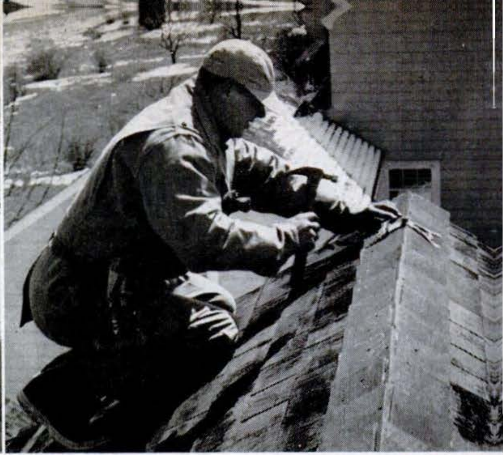
2 RIDGE SADDLE nailed to peak will hold rod. Underwriters' Laboratories sets rules for number of rods and spacing.
