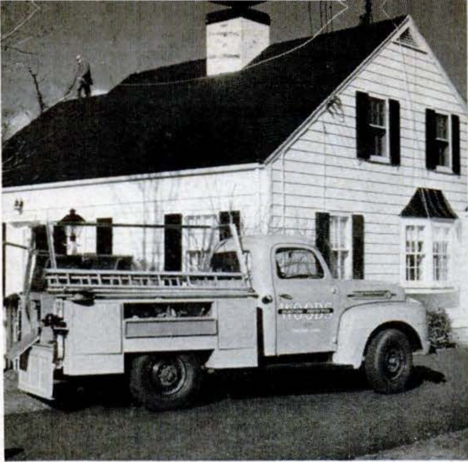
1 CABLE IS STRUNG along roof and down both ends of house. Truck-workshop carries fittings to suit all structures.
