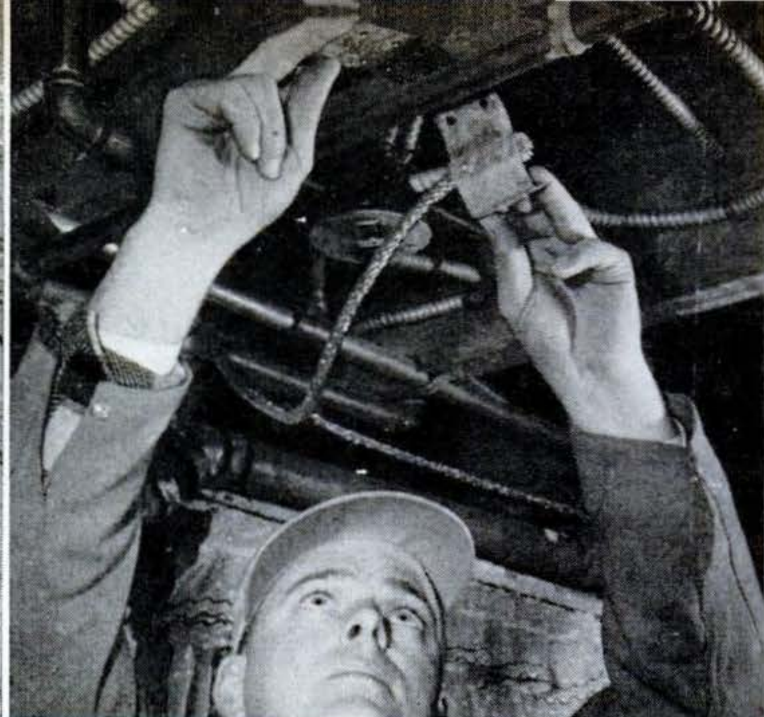
13 CELLAR BRANCH CABLE is bonded to water pipe. Clamps, tees and connectors are specially made, can stand 2,000-pound pull.
