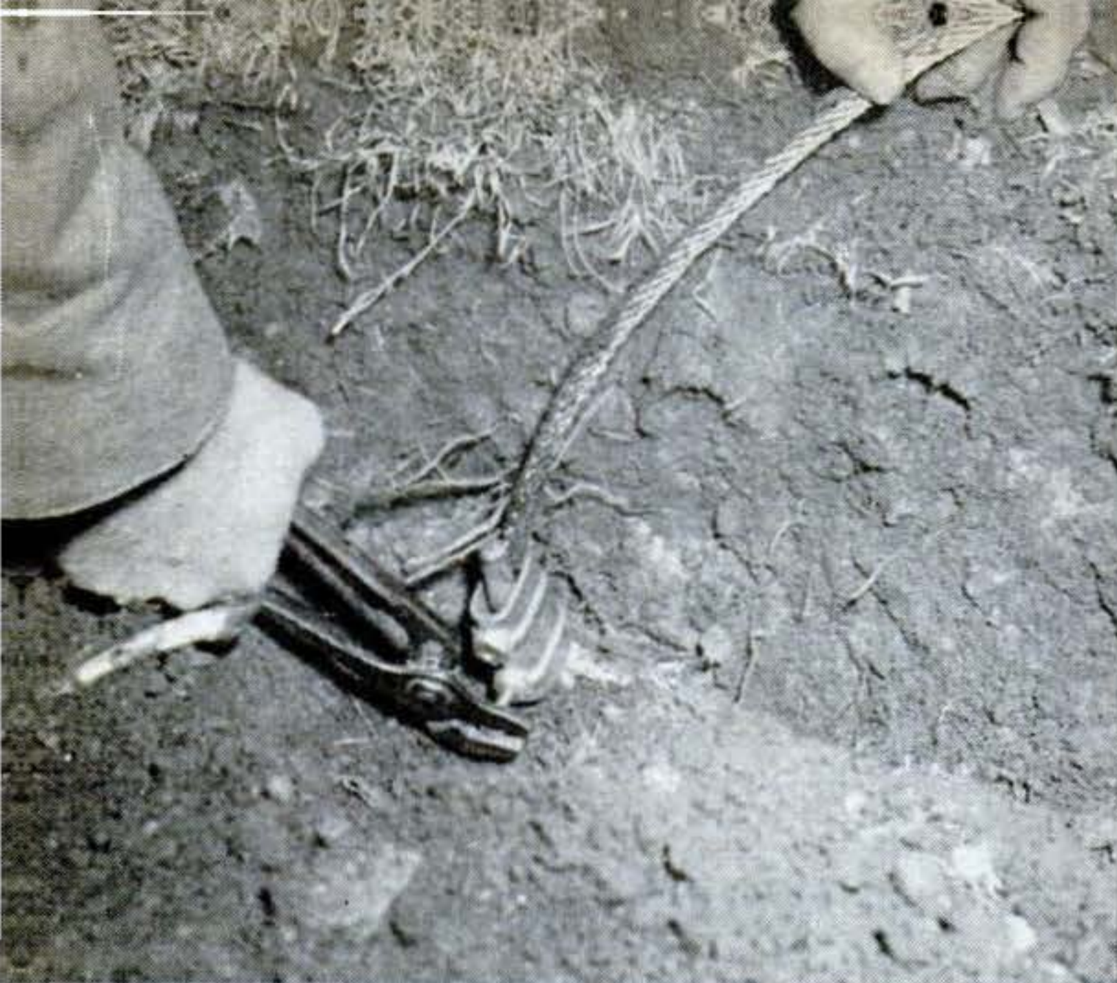
12 GROUND-BAR CLAMP links cable and rod a foot or so below ground. At least two grounds are used; this house got three.
