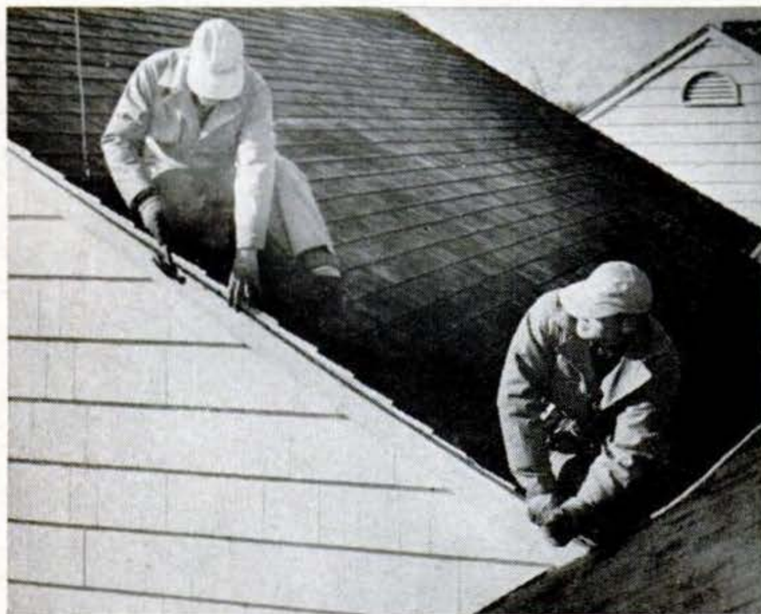
8 CABLE goes under eave. One man pulls it tight while another nails and clamps it. First paint job will hide it completely.
