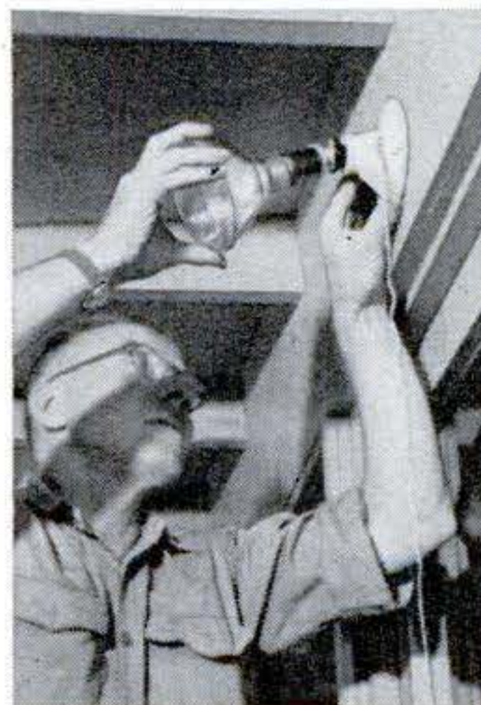
QUICKEST WAY to controlled yard lighting is a porcelain socket on the side of house protected by roof. Add swivel and reflector bulb. Mount socket on an octagon box recessed in wall.
