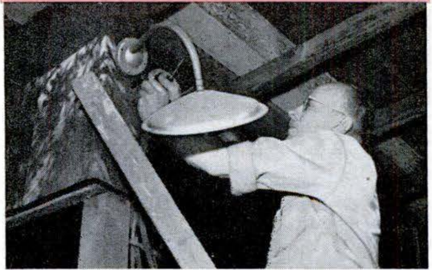
UTILITARIAN LIGHT outside an outbuilding is provided by a simple fixture like this. Conduit serves as the bracket. A switch is placed in easy reach elsewhere, often at the house.
