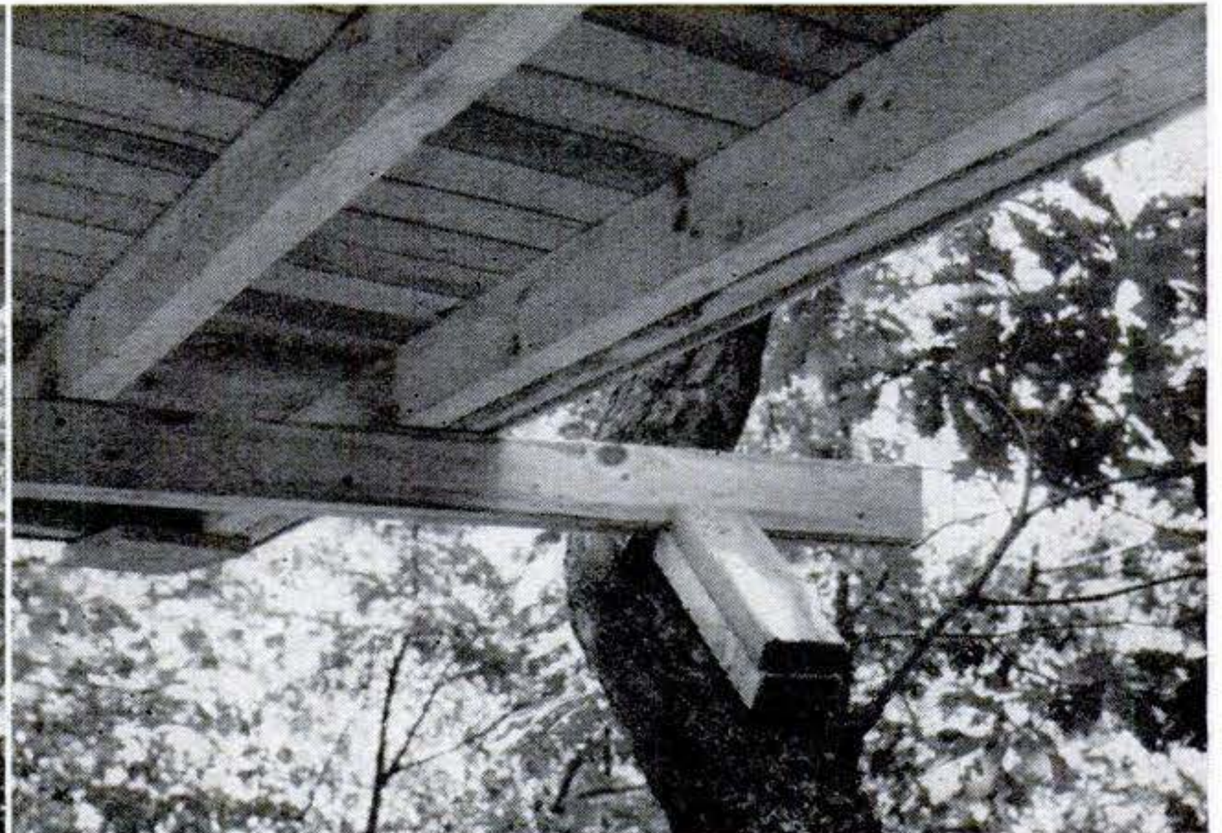
NATIVE PINE AND FIR were used, much of it green; but there is less warping than in a steam-heated apartment. The substructure was left open to make safety inspection easy.
