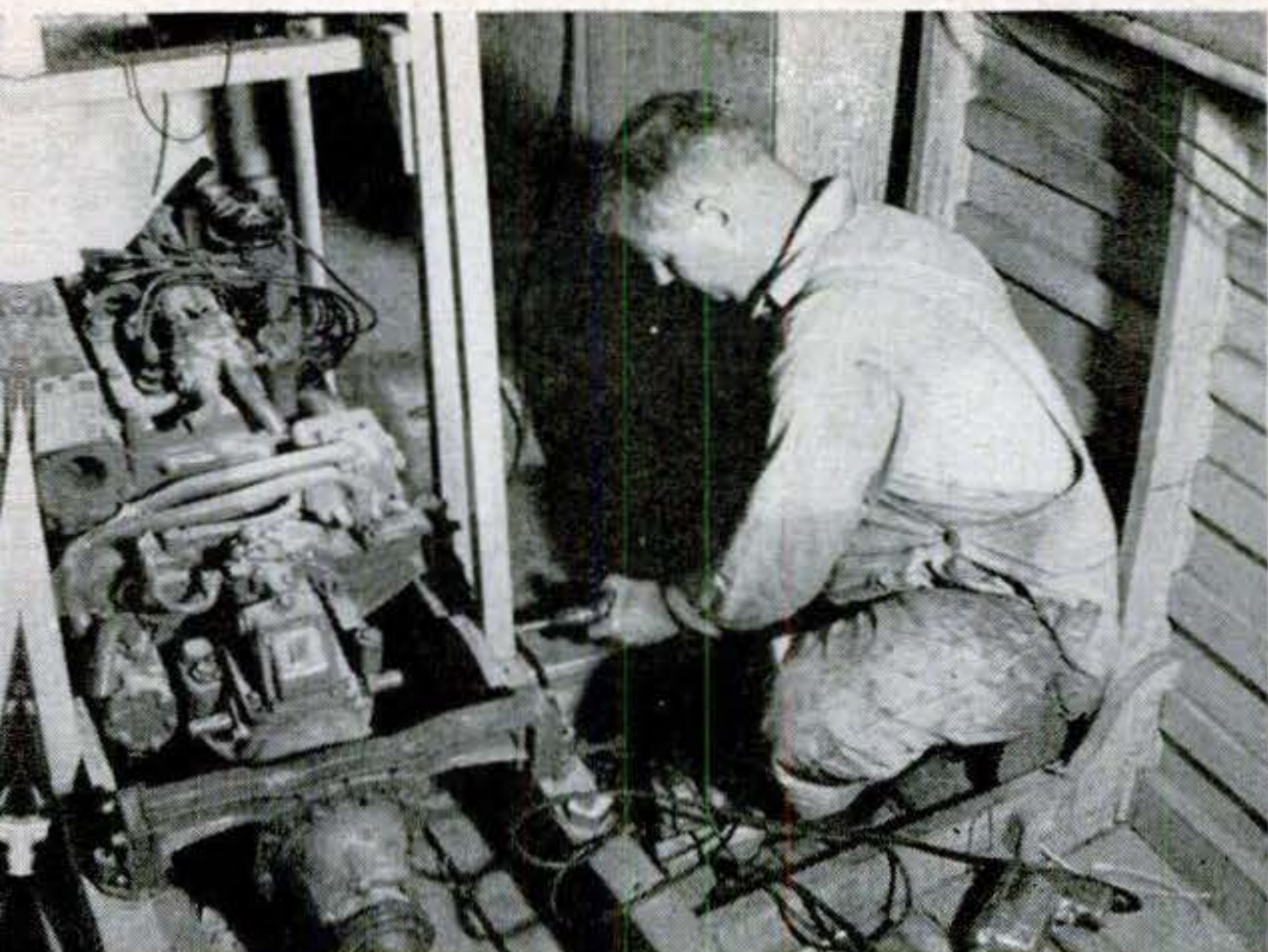
INSTALLING A POWER PLANT isn't the headache with Trident's facilities that it can be in backyard or basement sites for boatbuilding.
