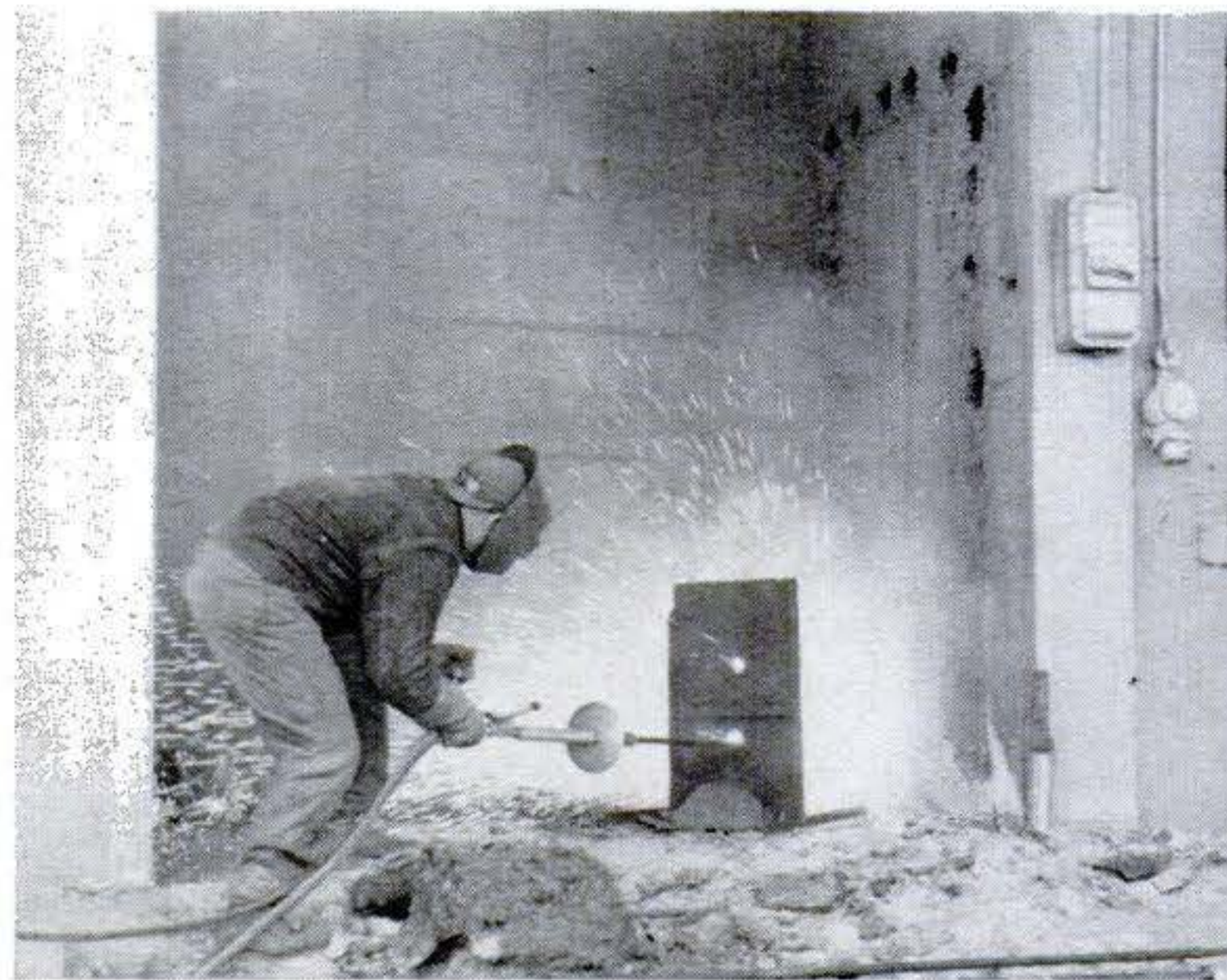
HOT LANCE. Intense heat—nearly 10,000 degrees—melts through a 1½-foot concrete wall (above) at Hill Air Force Base in Utah. The iron-pipe lance, consumed by its own heat, is replaceable. It does two weeks' work in a day.
