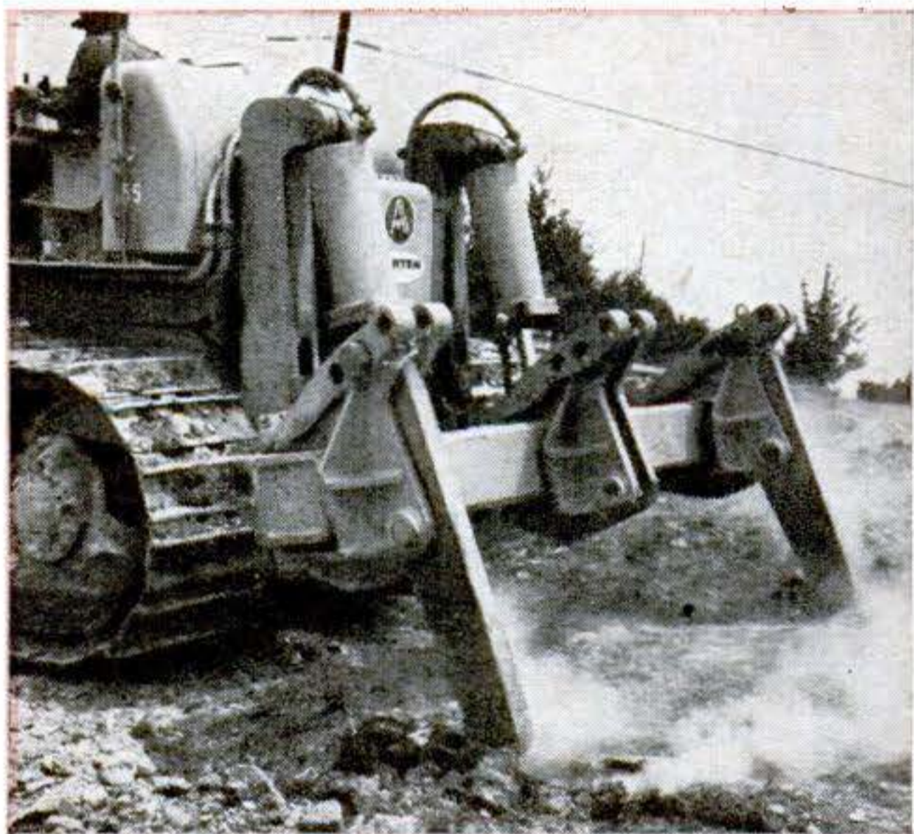
2 TUGGING IN LOW GEAR , tractor's pull and weight sink teeth into breaking rock.
