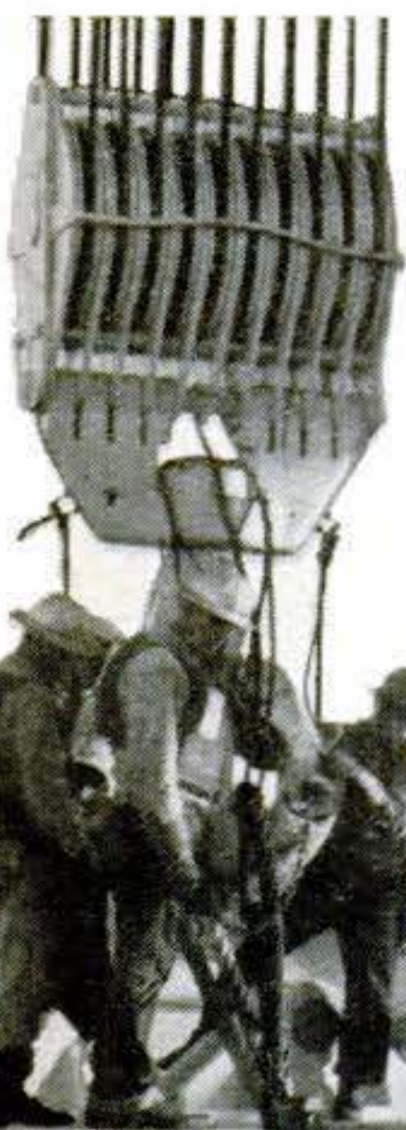
Massive 20-part lower block of the Herman B derrick is brought down slowly to pick up one of the special 2½-inch hoisting cables before the strongback is lowered. The Bolin's block can be seen at far right in picture.
