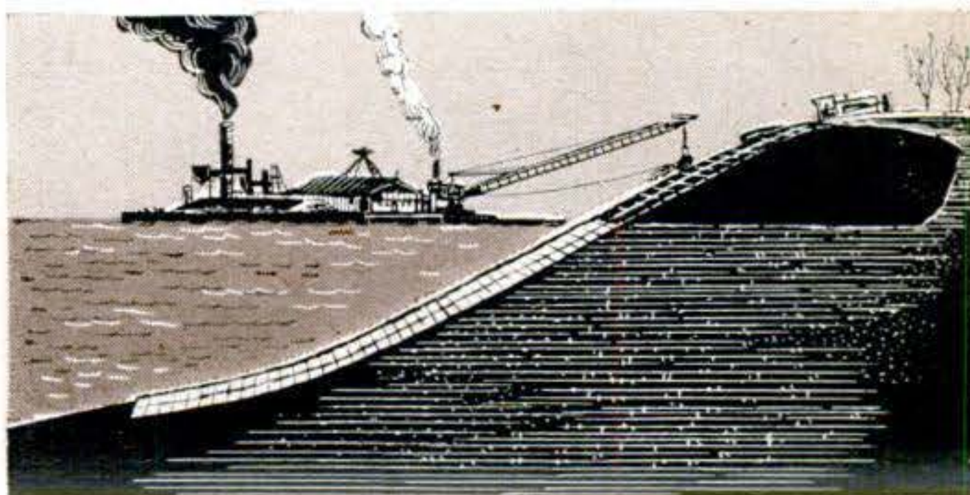
Wires holding carpet to barge are cut away, and carpet is left on bottom to control floods.
