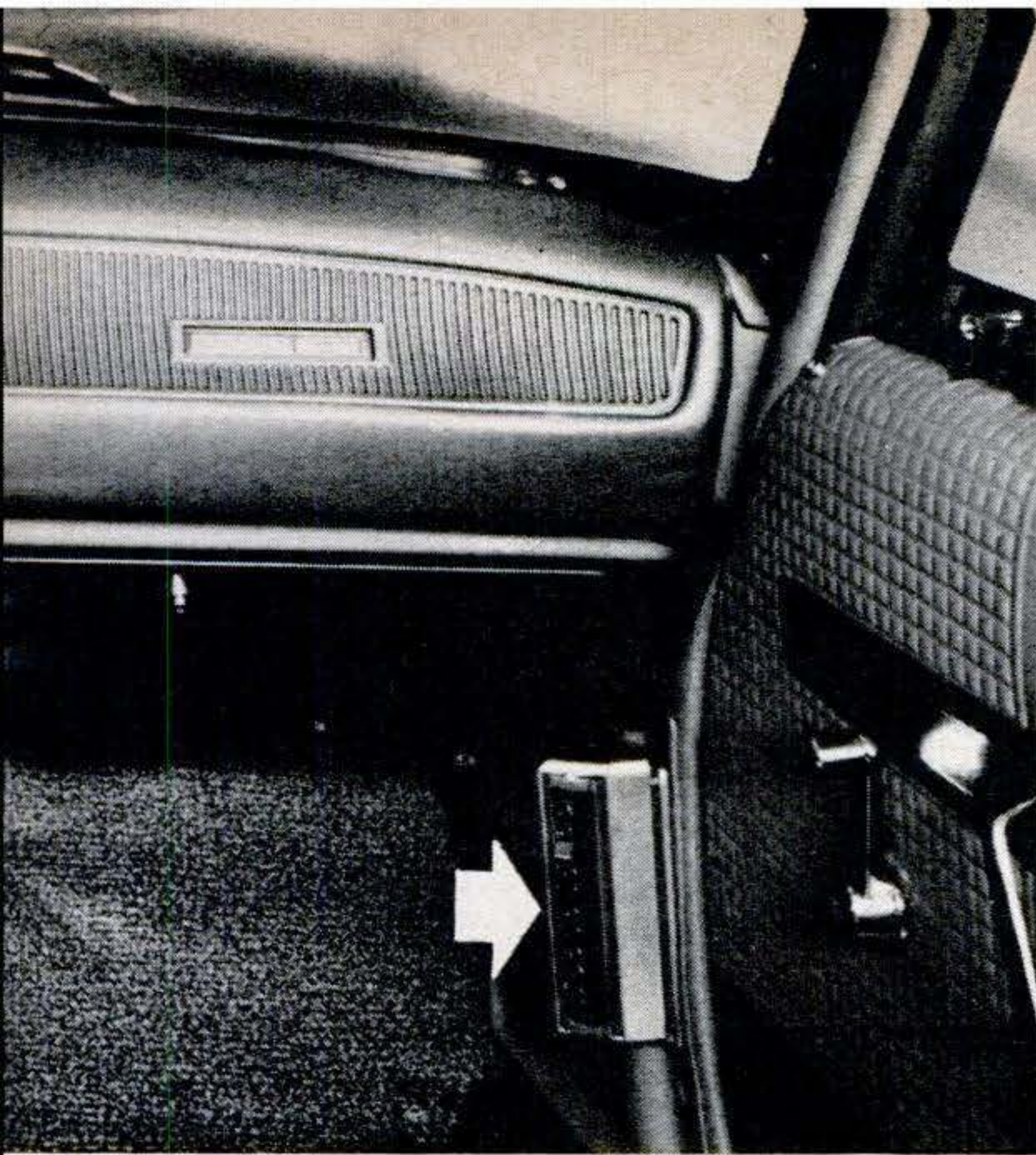
outlets (arrows) as in this Dodge installation.
