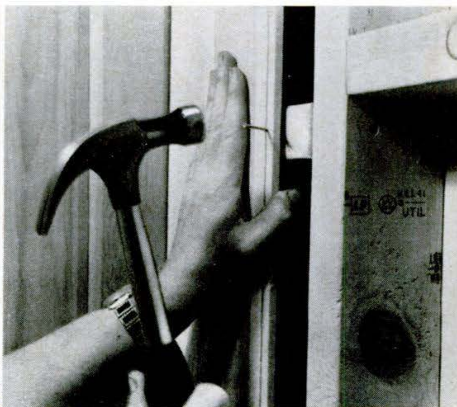
Start sixpenny finishing nails in the tongue and drive them at an angle through the solid wood behind it. The groove of the next piece covers nails.
