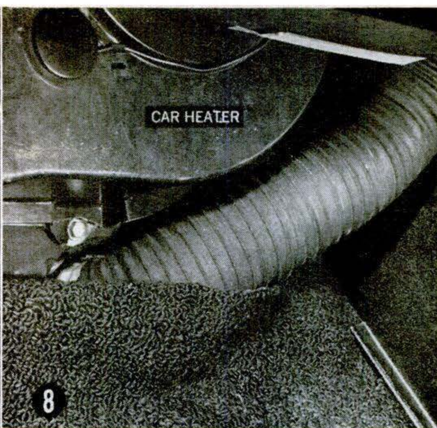
Standard flexible cloth tubing connects blower to panel. System's cost was as follows: junk parts, $13; refrigerant oil, $.75; Freon, $4; belt, $1.40; tubing and fittings, $4.37; miscellany, $1.22.
