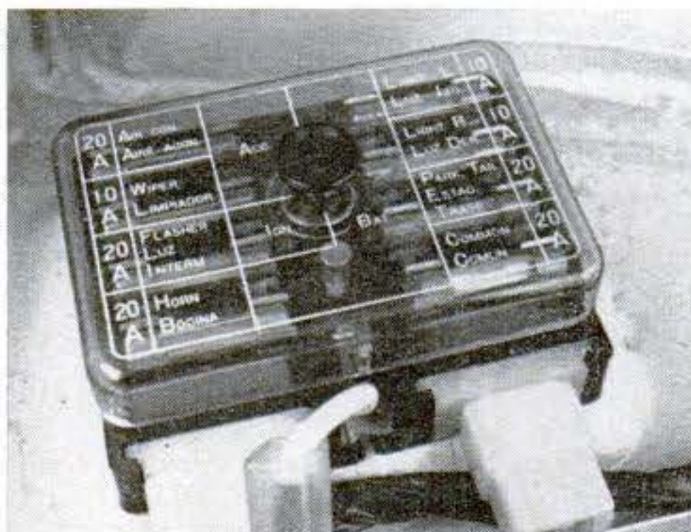
Datsun fuse box is located under the hood (right rear corner), and is labeled in two languages: English and Spanish.
