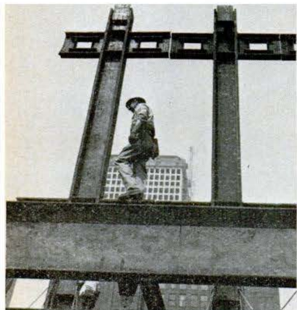
Structural-steel columns arrive welded to 15-foot spandrels—with welds pretested ultrasonically. At the site, ironworkers bolt the units together with splice plates.
