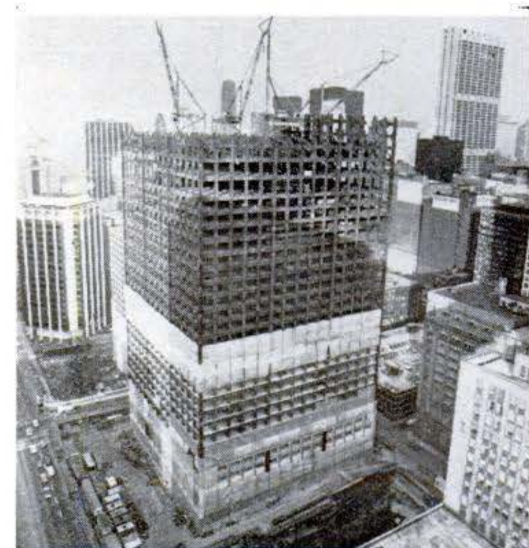
Sears Tower is shown as it appeared last December—about one-third completed. It's rising at the rate of two floors a week.
