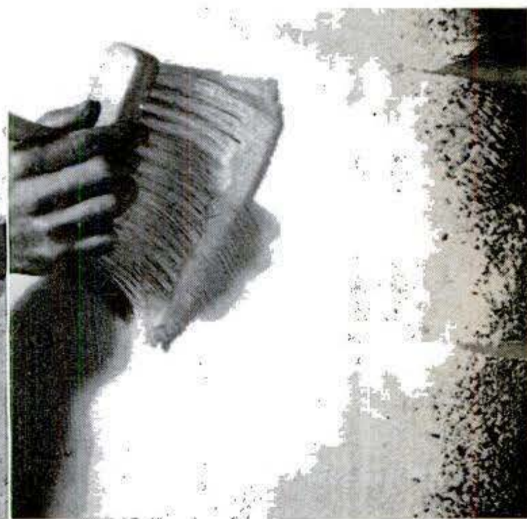
job. Final step: cementitious paint to fill remaining cracks and pinholes, smooth the wall, and make the color uniform.
