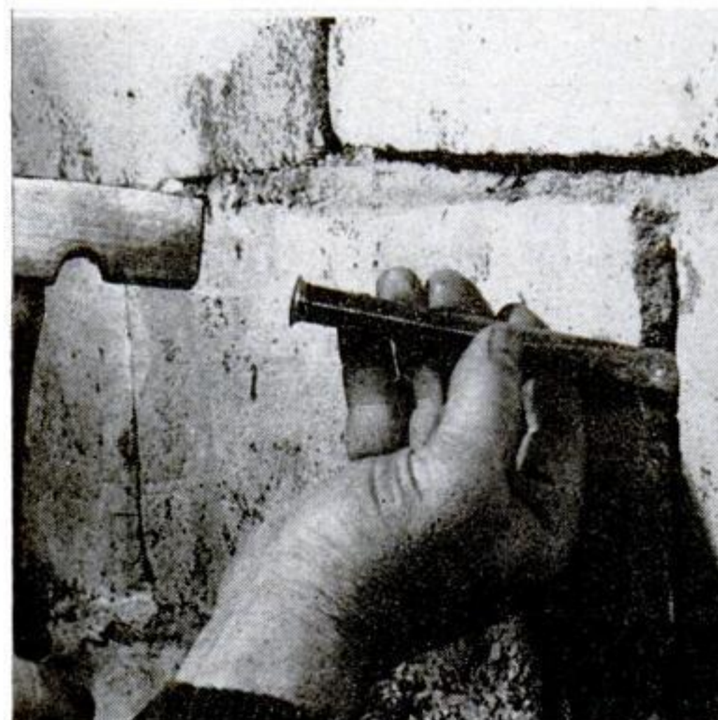
Hammer and chisel-chip the edges of crack. Undercutting avoids thin, nonsetting edge in patch. (Widen crack to 3/4" for ordinary
