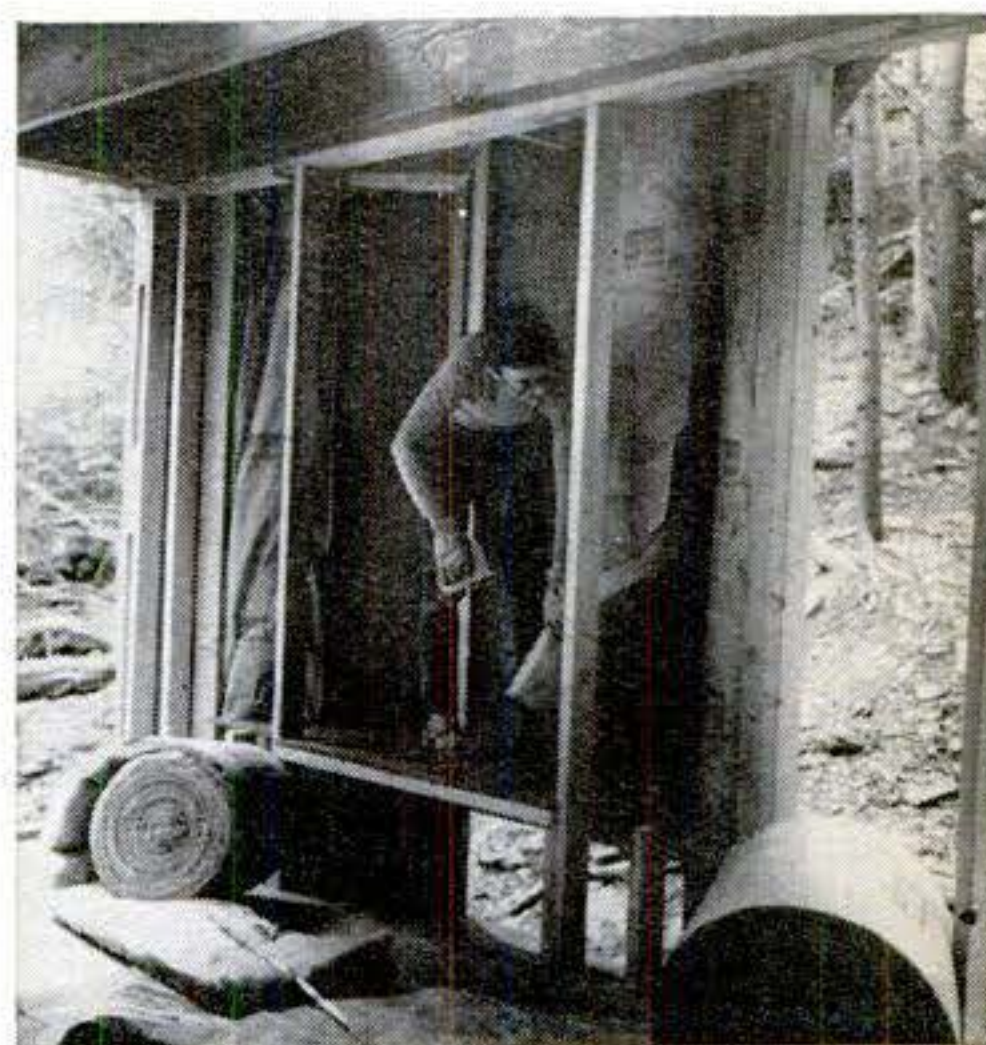
Chase is part of wall, so must be fully insulated if house is to be winterized. One roll each of 15" and 23" Fiberglas does it.
