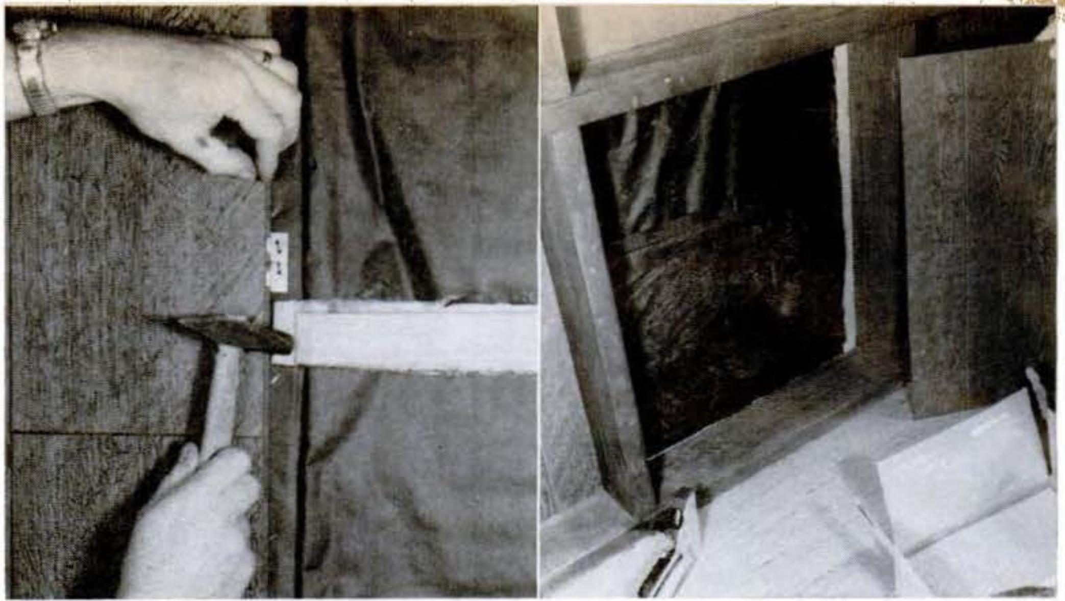
Paneling goes up with special clips that provide automatic spacing. Note header between studs to which framing for storage cabinet will be nailed once paneling's done.
