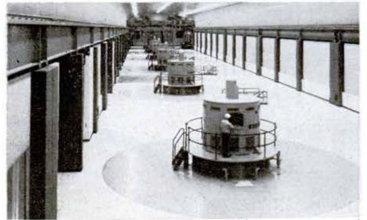
Underground power plant at Oroville dam. Floor covers bulk of electrical generators.
