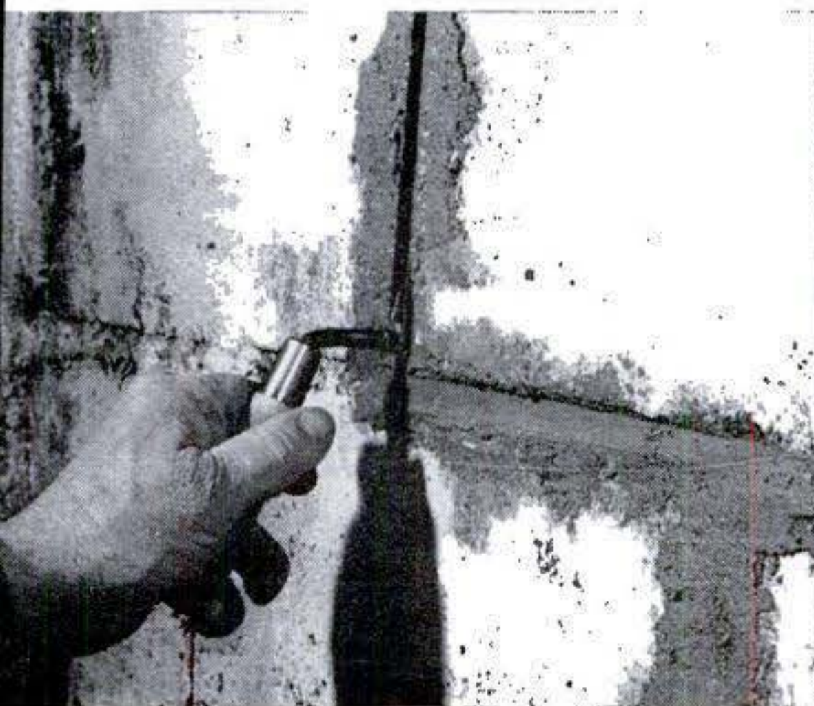
or small mason's trowel. Narrow tuck-pointing trowel (above) is handy for forcing material into crack, filling it completely.
