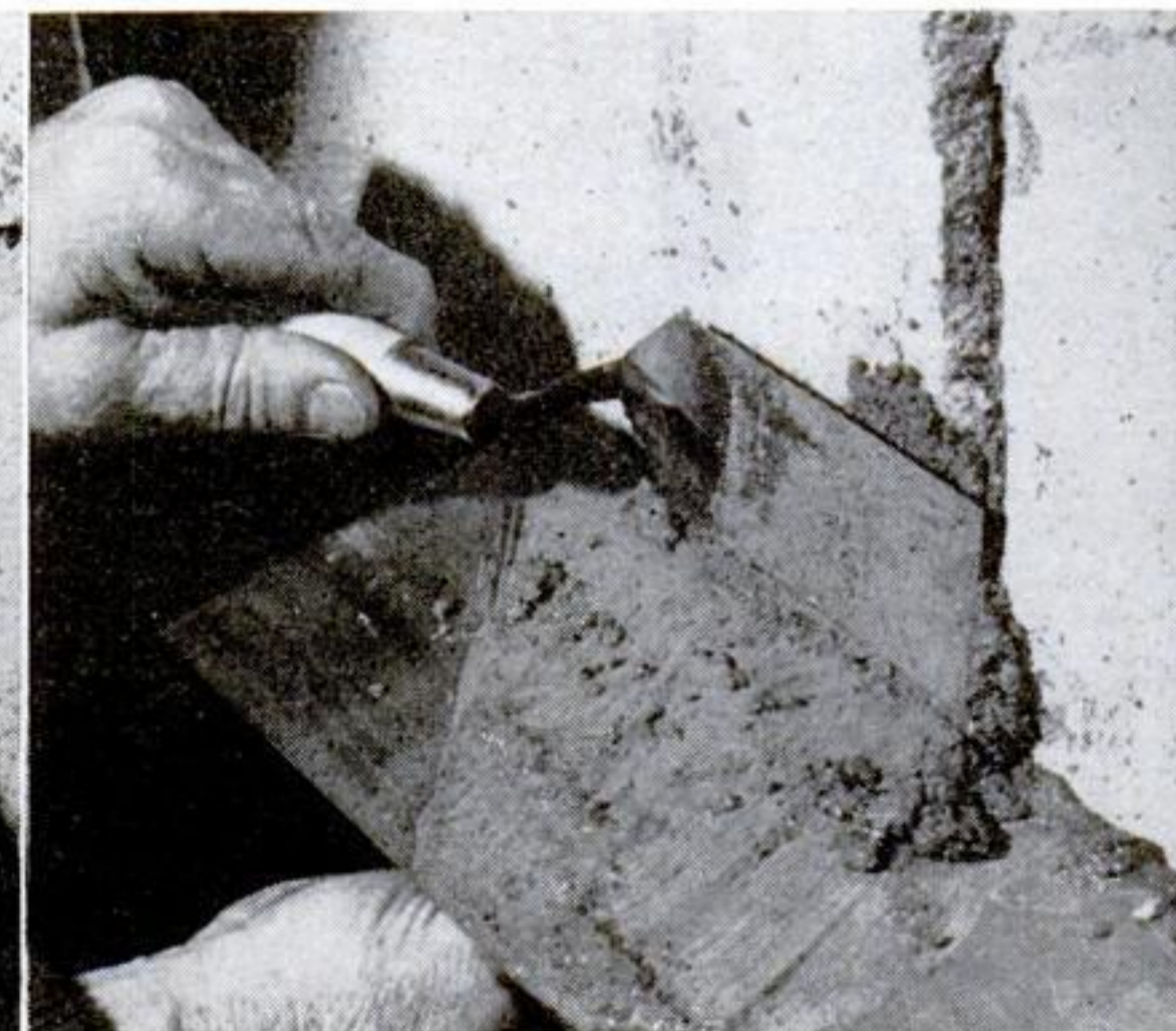
patching cement or hydraulic cement.) Above, holding plaster trowel as "hawk," trowel mortar in firmly with square-ender
