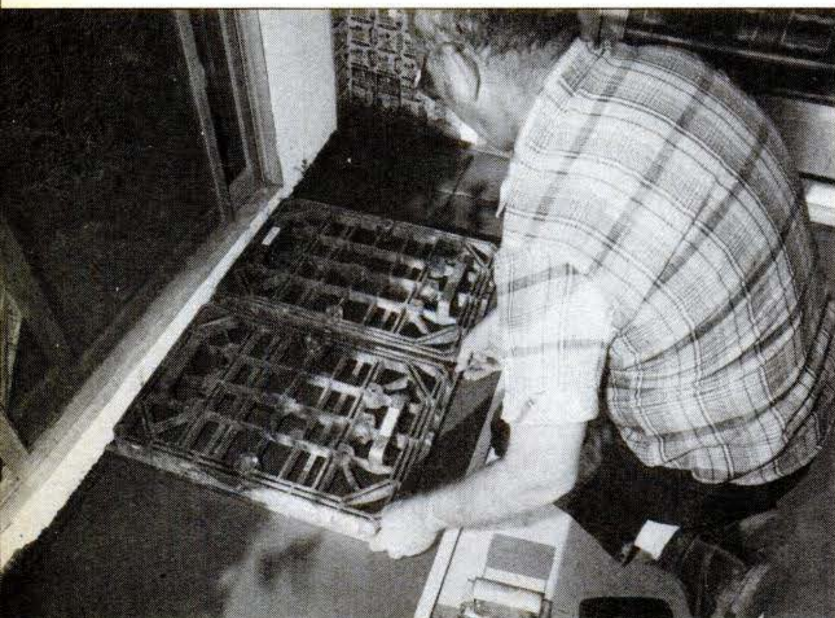
Working from knee board permitted greater care in positioning pads, but area under board needed extra float.
