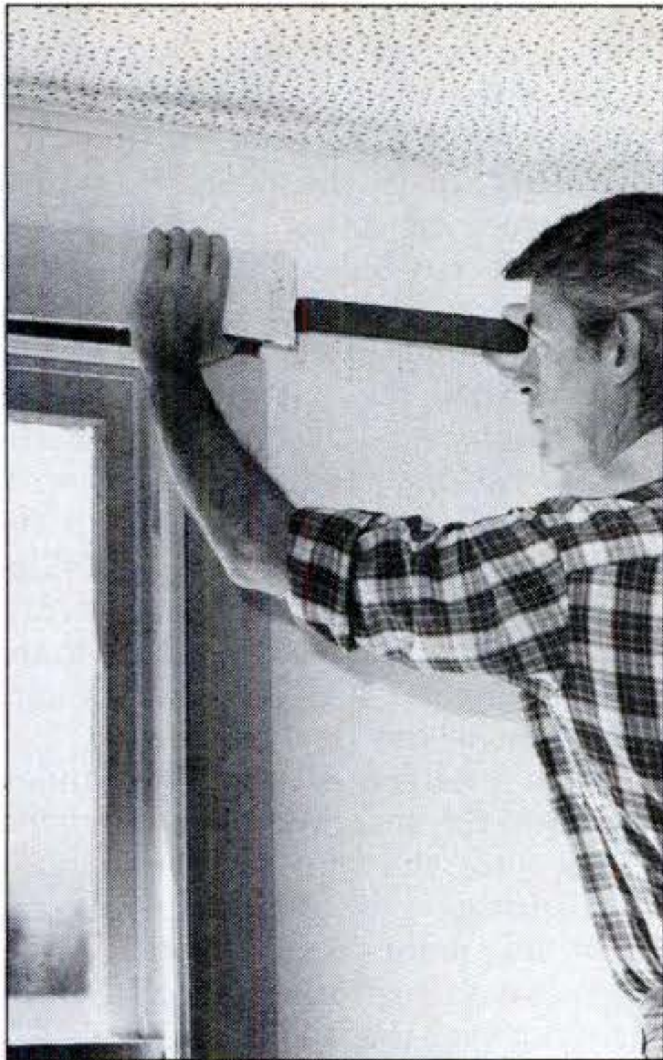
Replacement of old window starts with removal of interior casing to expose the wall. Height matches the sliding door.
