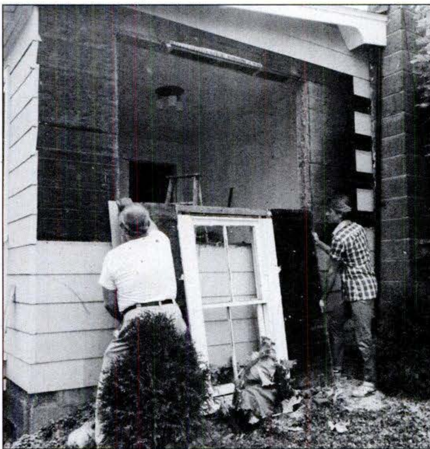
Wall section, complete with old window, is lifted out and lowered to the ground. It can easily be dismantled.
