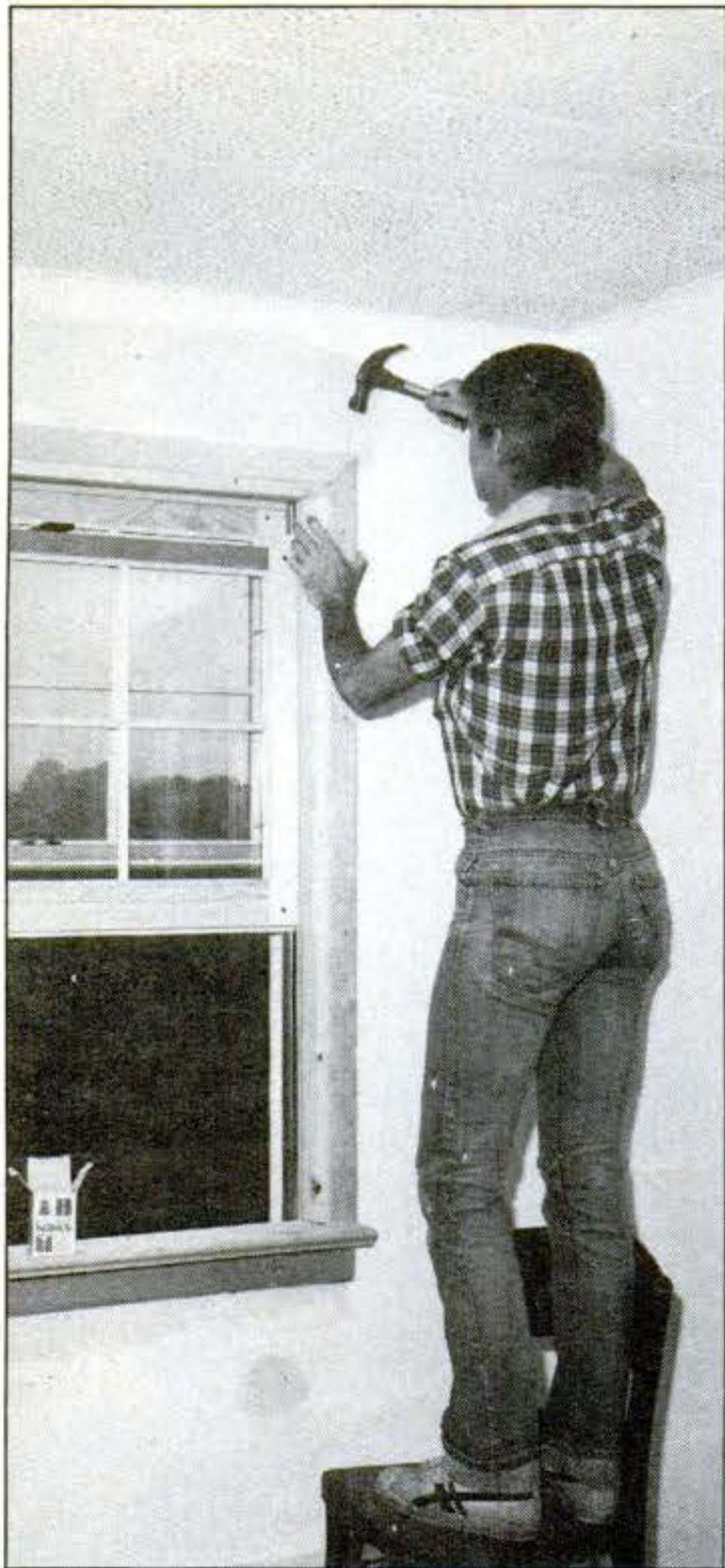
Interior trim is nailed in place after sanding the wall smooth. Wood can be painted or stained to match decor.
