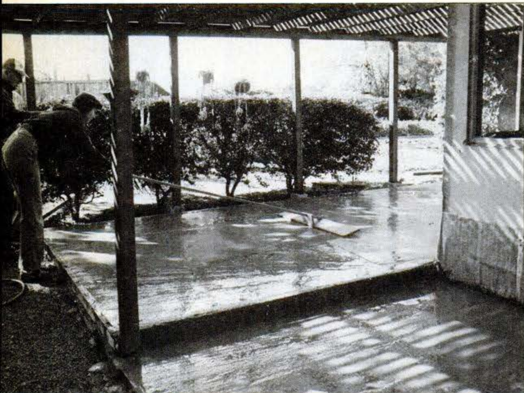
Slab to be stamped is prepared in usual way. Bull-float immediately after strike-off to maximize stamping time.
