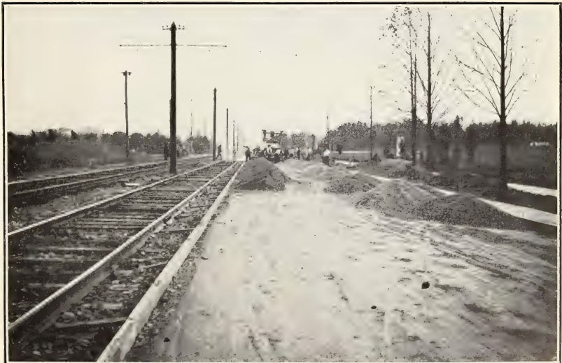
FIG. 2.—SAND AND GRAVEL PILED ON SUBGRADE READY FOR USE. EXPERIMENTAL CONCRETE ROAD, CHEVY CHASE, MD.
