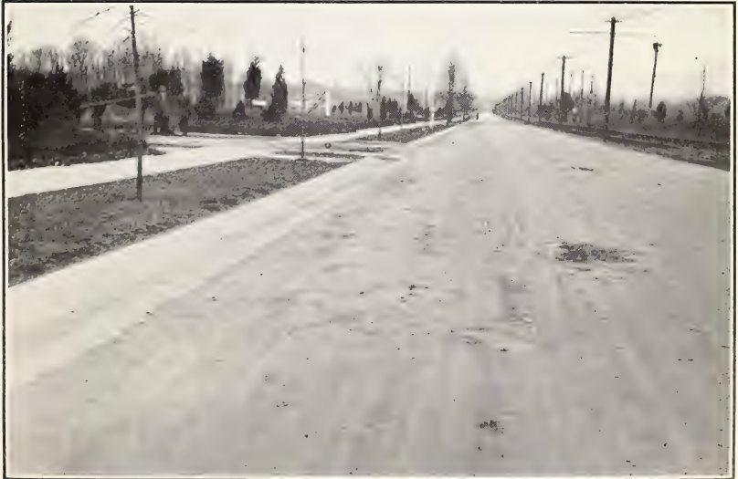
FIG. 2.—SHOWING UNSATISFACTORY CONDITION OF BITUMINOUS WEARING SURFACE AFTER LESS THAN ONE YEAR'S SERVICE.
