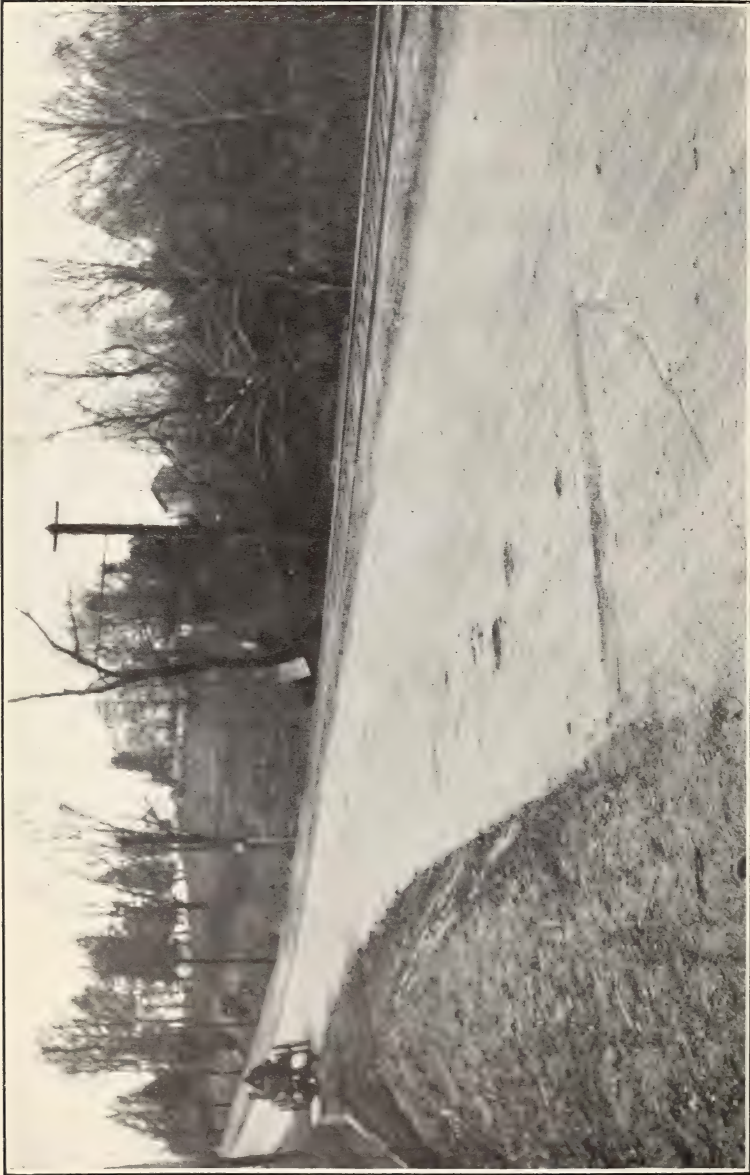
FAILURE OF CONCRETE PAVEMENT CAUSED BY SETTLEMENT OF EMBANKMENT.
