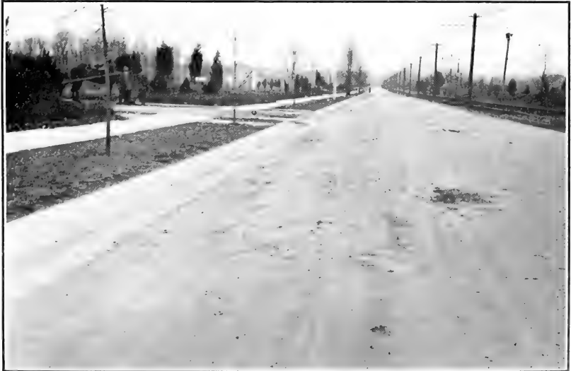
FIG. 2.—SHOWING UNSATISFACTORY CONDITION OF BITUMINOUS WEARING SURFACE AFTER LESS THAN ONE YEAR'S SERVICE.
