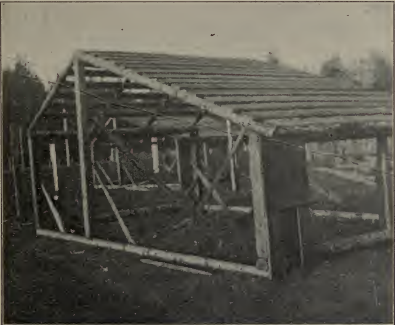
The frames of houses may be made from trees about 3 inches in diameter. The above shows a Tolman house in the course of construction.
