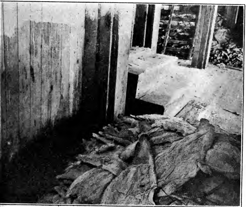
FIG. 3.—Marked reddening on the wall near the floor in the storeroom.
