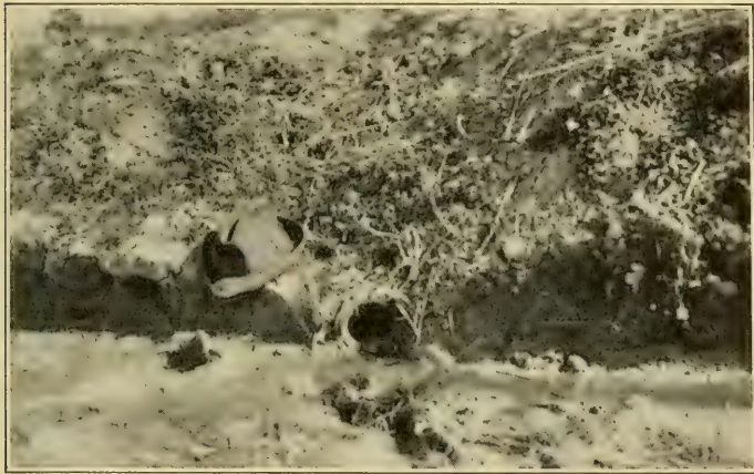
FIG. 29. — Drainage outlet that is likely to clog.
