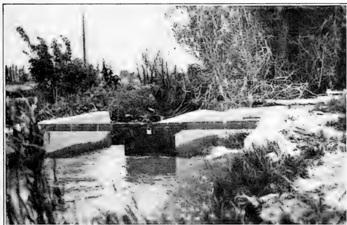
FIG. 26. — Cement dividing gates save trouble.
