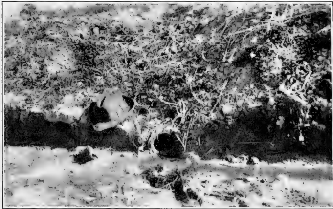
FIG. 29. — Drainage outlet that is likely to clog.
