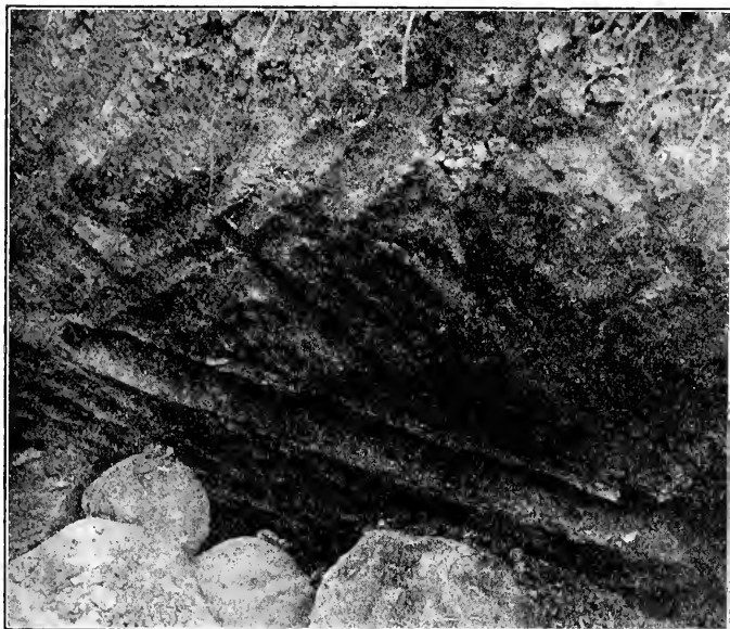
FIG. 77. Section of a 20-year-old tile drain in heavy clay soil. Note the more open structure above the drain.
