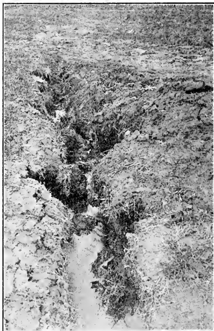
FIG. 93. A poorly constructed outlet for a line of drain tile.
