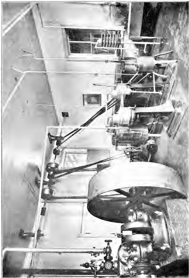
FIG. 67.—A corner of a separator-room, showing a good arrangement of machinery. (Creamery at Walker, Ia.)
