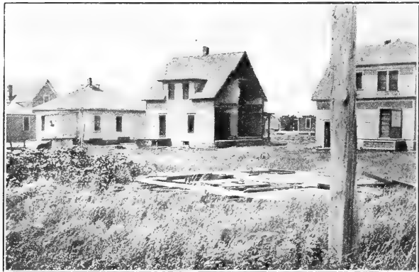
FIG. 4. House with end blown outward.
