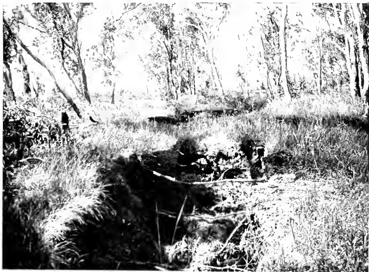
Trench formed by subsurface drainage, Greenmount, W.A. 1. Looking downhill; 2. Looking uphill.
