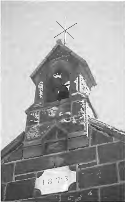
Fig. 2. Stables, 'Larra', designed by Davidson and Henderson 1873; detail with lightning conductor. (Photo: author.)
