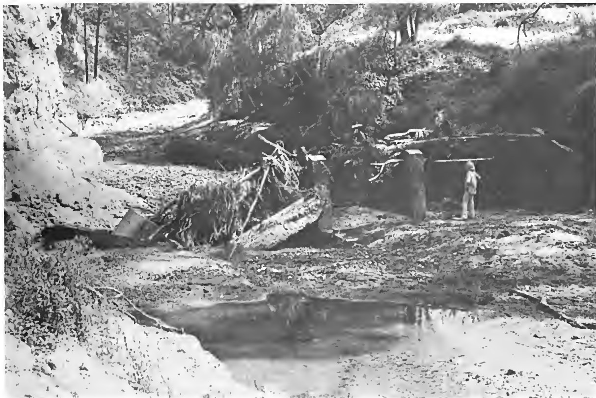
Fig. 6—Wood and concrete drop structure across Eaglehawk Creek outflanked by bank erosion. Looking upstream.
