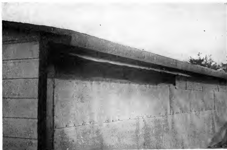
FIG. 67.—An efficient rear ventilator for summer use. It allows the air to enter the back of the house, and circulate between the sheathing and the roof, cooling the roosting quarters on summer nights. This is most valuable for shed-roofed houses that are covered with paper.
