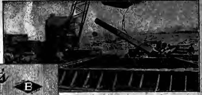
Temporary treating-plant constructed of wood and lined with galvanized sheet iron. Used for creosoting over 250,000 feet B. M. of timber for floor-framing of industrial plant.
