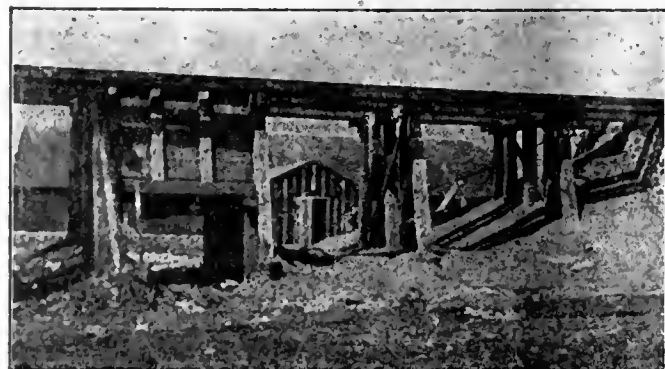
Trestle in coal-yard of copper mine, portions of which were treated by the Brush Method nine years ago. Treated timbers are in perfect condition.
