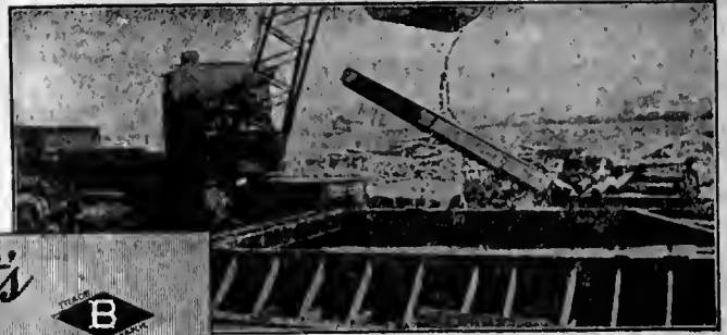
Temporary treating-plant constructed of wood and lined with galvanized sheet iron. Used for creosoting over 250,000 feet B. M. of timber for floor-framing of industrial plant.
