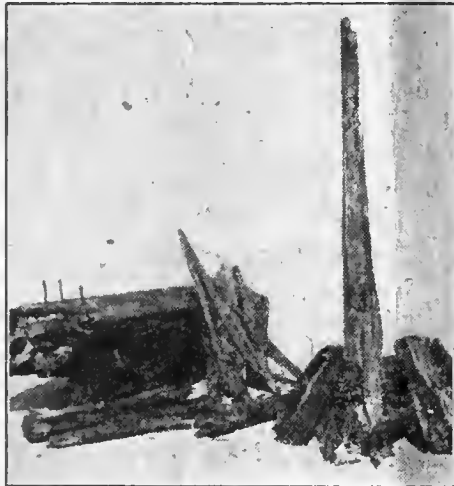
8 x 12 inch timber destroyed by decay after nine years' service in a paper-mill.
