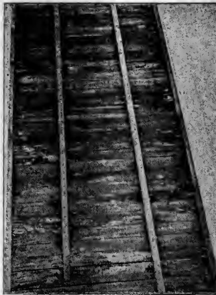
A "close-up" section of roof weakened to a danger-point due to decay of planking. (Courtesy American Lumberman.)
