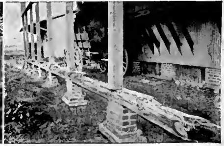
Untreated sills and posts in contact with brick foundation piers entirely destroyed by white ants (termites).
