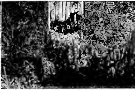
Serious deterioration of telegraph pole near ground line due to white ants (termites).
