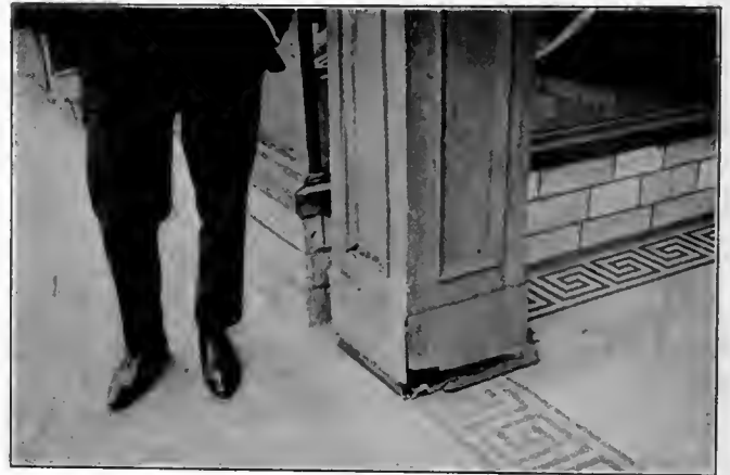
BASE OF PILLAR ROTTING
