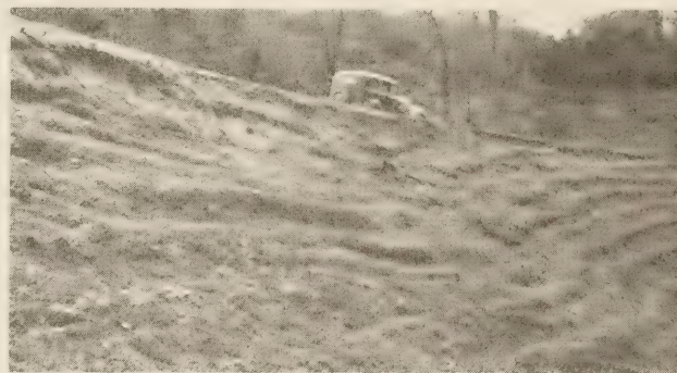
FIGURE 13.—PARTIAL FAILURE ON A FILL PROTECTED BY HAY WATTLES.
