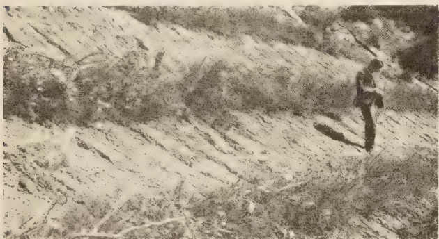
FIGURE 7.—FILL SLOPES PROTECTED ACCORDING TO METHOD A. PICTURE SHOWS A SECTION ABOUT 70 FEET BELOW GRADE.
