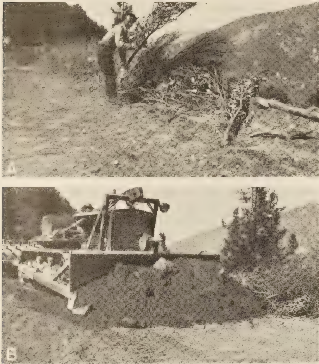
FIGURE 5.—A; PLACING A LAYER OF BRUSH. B; A BULLDOZER COVERING A BRUSH LAYER WITH EARTH. THE BULLDOZER IS PULLING A SHEEPSFOOT ROLLER USED TO COMPACT THE FILL.
