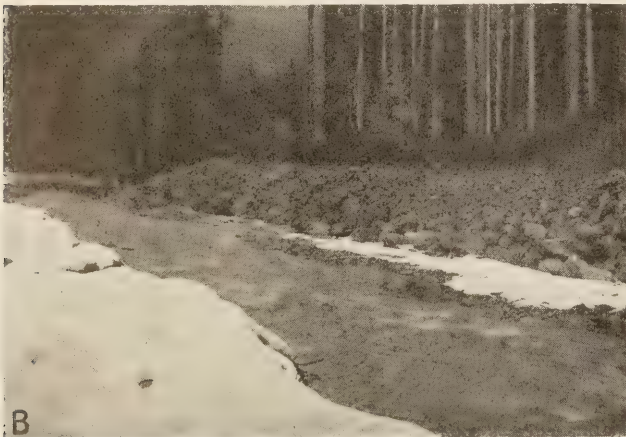
FIGURE 8.—TWO CHANNEL CHANGES: A, THIS CHANNEL CHANGE STRAIGHTENS A MEANDERING STREAM. THE RIPRAPPED SLOPE BEARS THE FULL FORCE OF THE CURRENT AROUND THE CURVE. B, THE LARGEST ROCKS ARE PLACED AT THE BOTTOM OF THE RIPRAPPED SLOPE.
