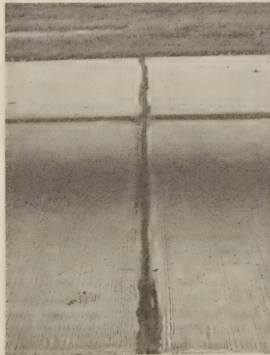
Figure 24.—Present condition of a surface-type, weakened-plane joint, typical of those at which the continuous reinforcement is structurally sound.
