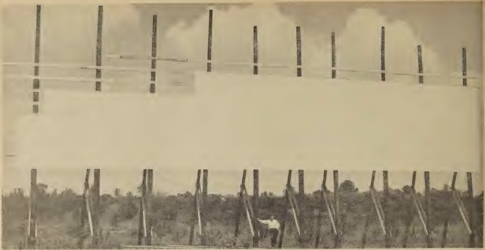
Closeup view of giant billboard under construction shows relative size of normal-size man. According to the number of 4- by 8-foot plywood sheets and the size of supporting structure, the completed sign will be 34 feet long and 20-24 feet wide.
