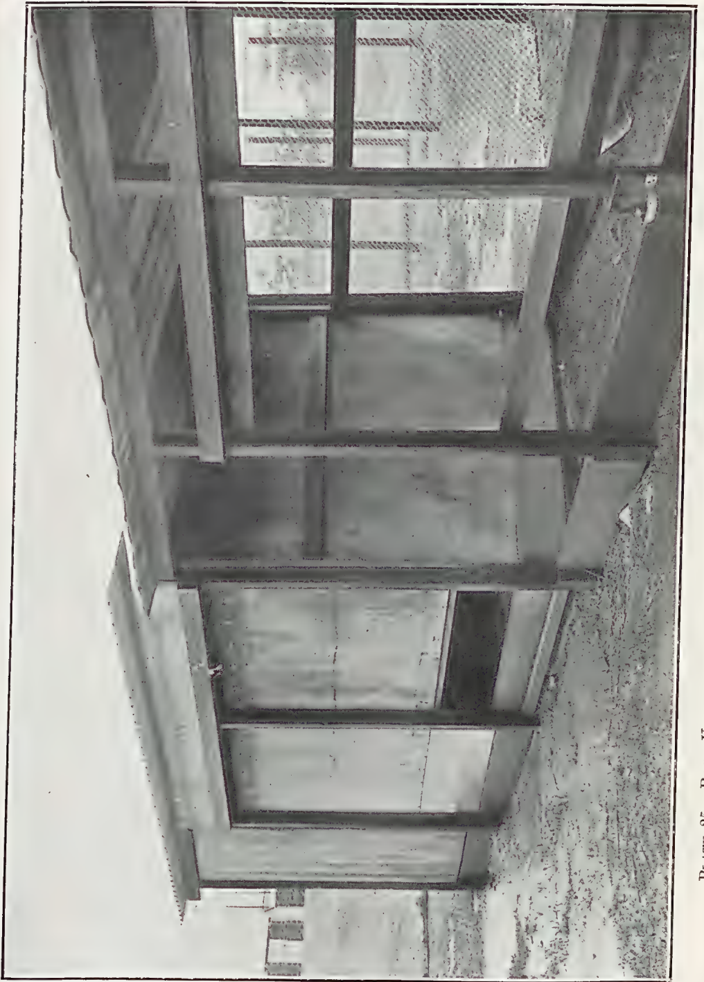
PLATE 25.—BACK VIEW, SHOWING A COMPLETED HOUSE AND FRAMING WALLED WITH ROOFING FELT.
