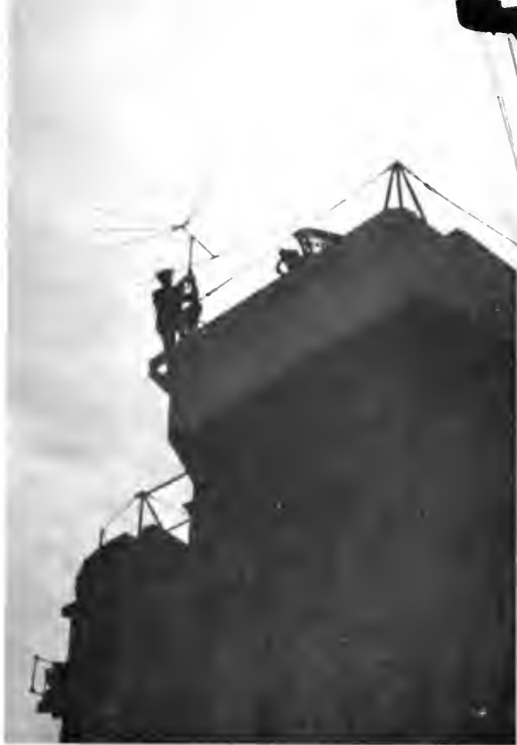
LEFT. AN RCA TECHNICIAN, WORKING HIGH ON THE SUPERSTRUCTURE, ERECTS A TELEVISION ANTENNA FOR ONE OF THE TV RECEIVERS ABOARD A CANADIAN CARRIER.
