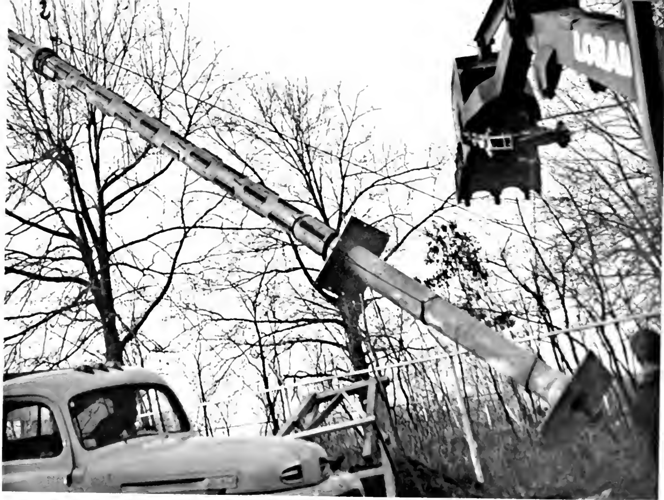
WORKMEN HOIST THE 30-FOOT UHF ANTENNA INTO PLACE AT NBC'S NEW EXPERIMENTAL TELEVISION STATION NEAR BRIDGEPORT, CONN.
