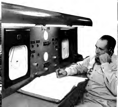
Employee of Sunray Oil Company checks information supplied him by microwave circuits extending throughout the company's pipe-line system.
