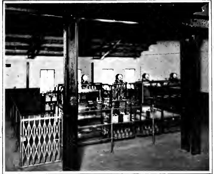
BEAM STATION EQUIPMENT
