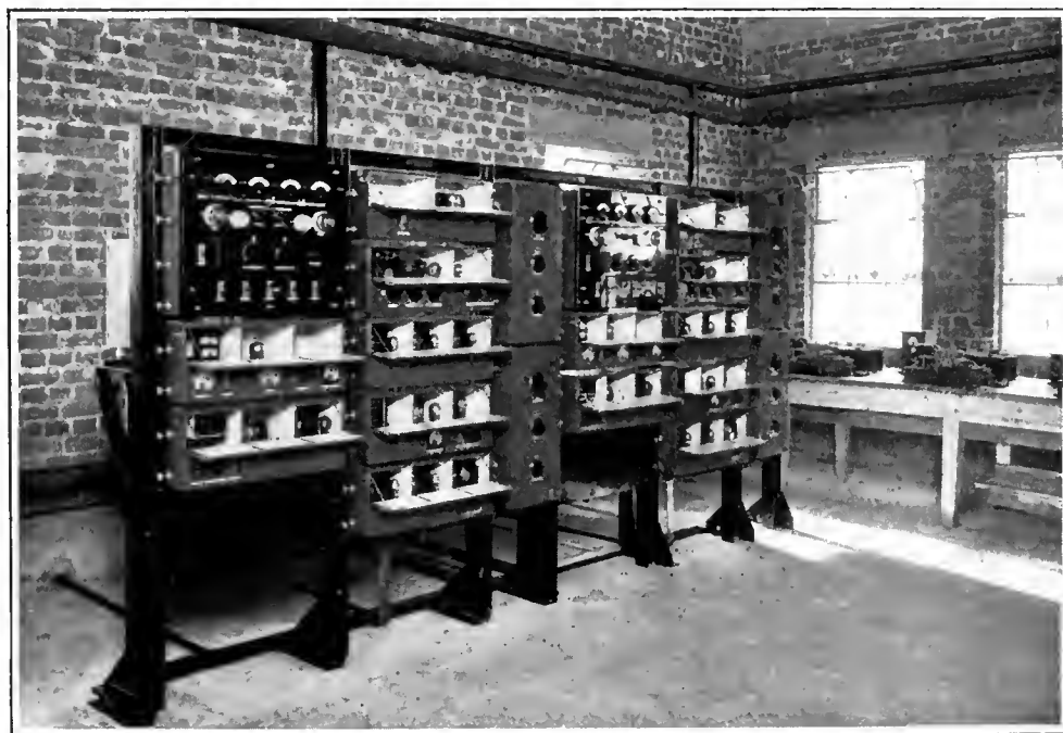
RECEIVING EQUIPMENT AT THE BRIDGEWATER STATION
