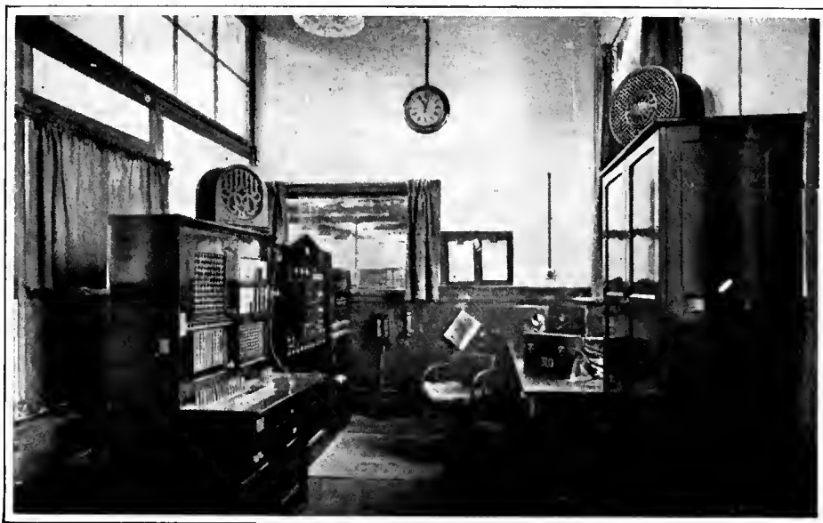
CONTROL ROOM OF 3 LO, MELBOURNE
