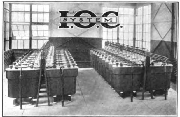
I. O. C. System installation General Electric Co., Pittsfield, Mass. This is one of five plants we erected for the General Electric Co.
