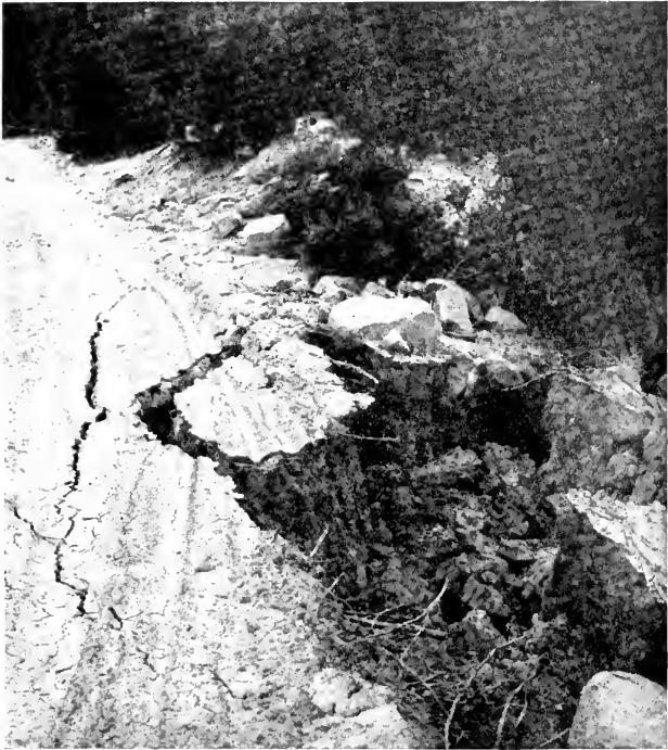
FIG. 55. — A WAGON ROAD ALONG A STREAM UNDERMINED DURING A TORRENTIAL FLOOD.
