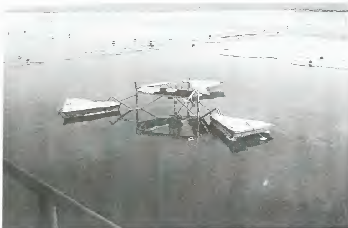
New Solarbee Treatment equipment at the Wastewater Treatment Plant
