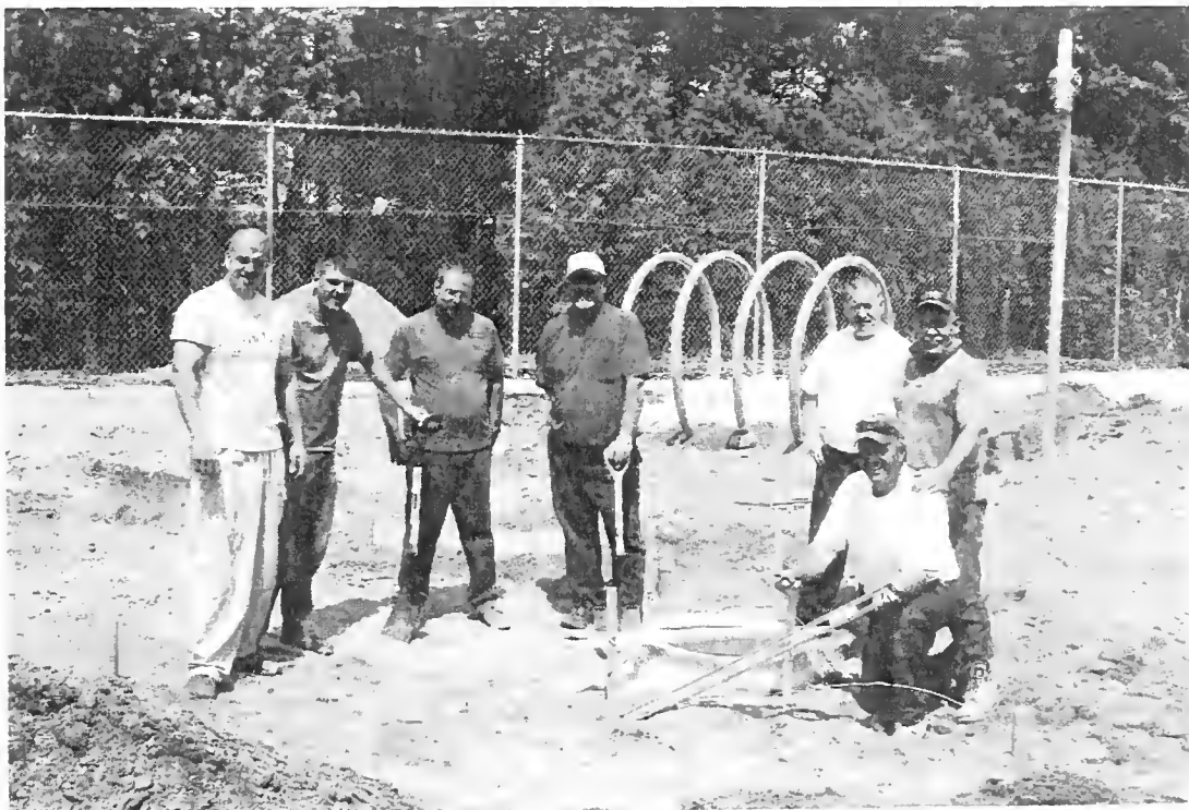
Parks & Recreation Dept. & DPW employees installing the new splash pad at the Rec. pool on Hampton Road. L-R: Mike Gingras, Brian Shea, Wayne Almon, Jim Colbert, Justin Hall, Steve Tucker, Dick Rowe
