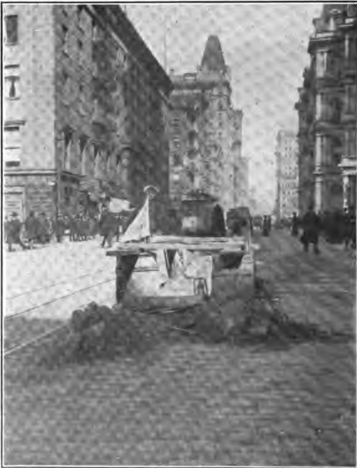
PITOMETER BOX AT BROADWAY AND FULTON STREET.
