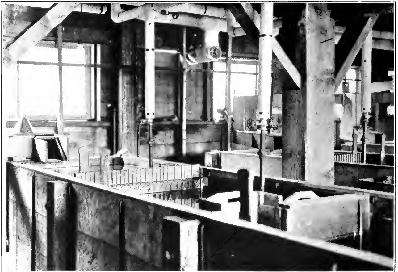
OIL SEPARATING TANKS AT WARDS COVE REDUCTION PLANT.
