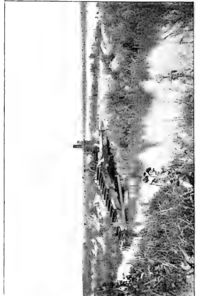
3. Supplementary engine and elevator for carrying water from dredge cut to pond, Monroe, Mich.
